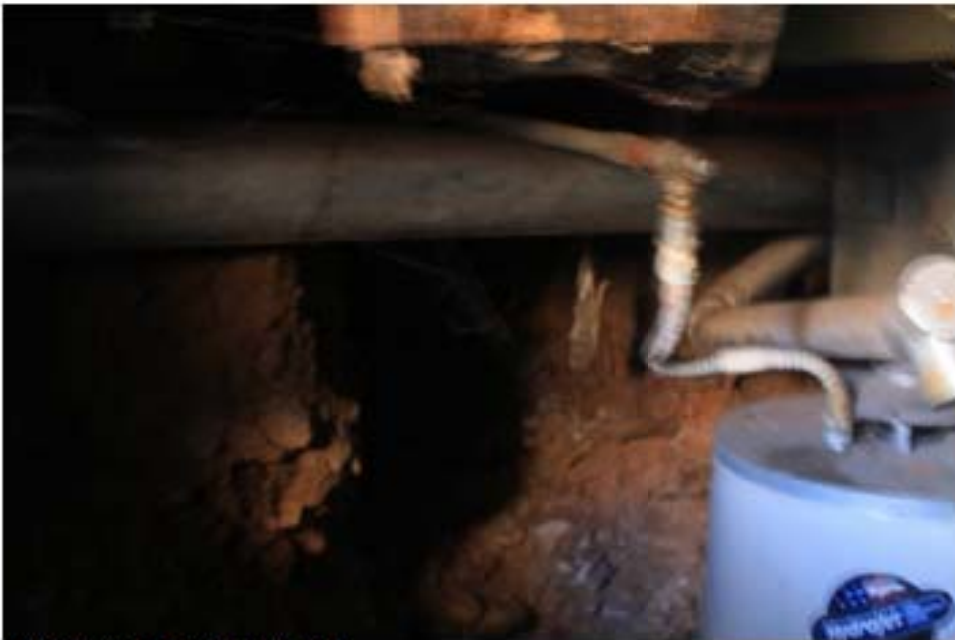
Hot water heater-venting?
