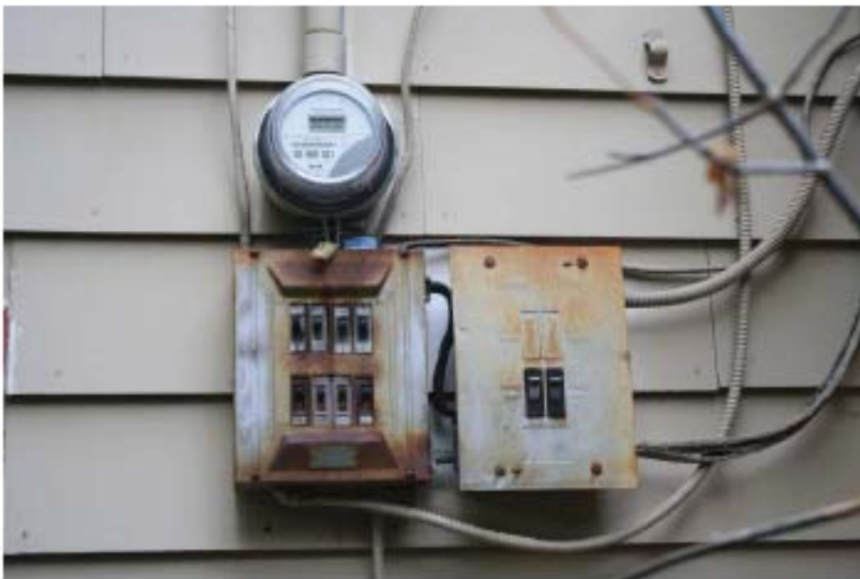
2. Closeup electrical service
