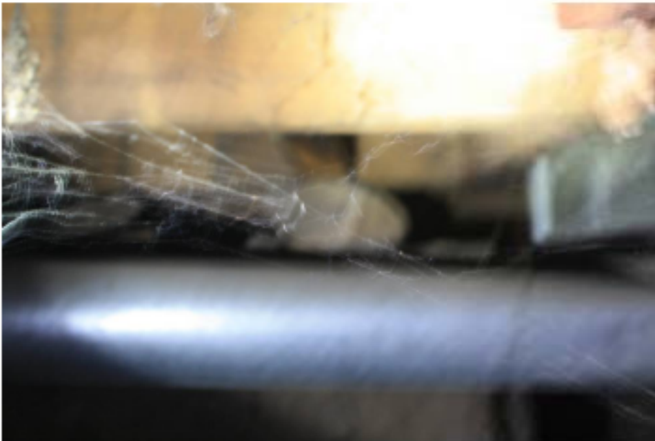
Duct work-exposed no insulation
