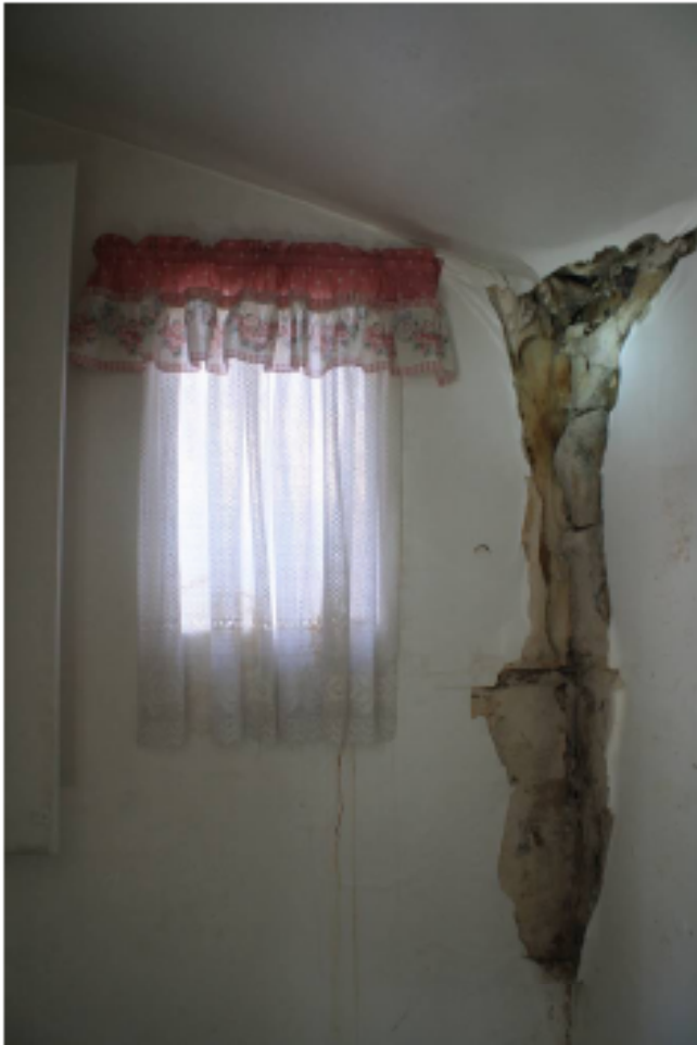
Visible mold-probably hidden mold
