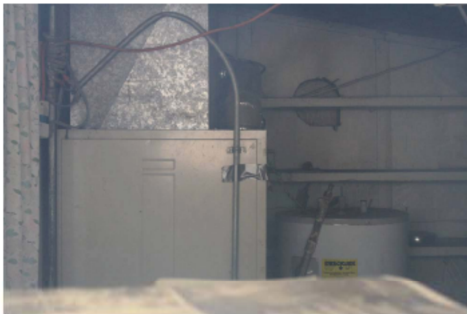
1.Mechanical room-furnace and water heater
