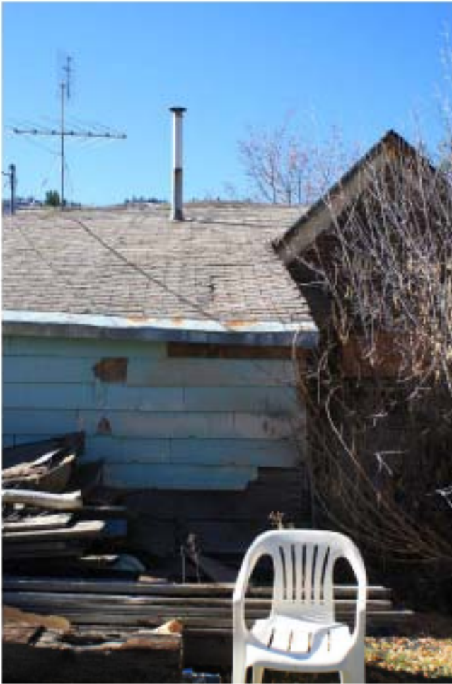
Northeast corner- roof damage and different wood siding
