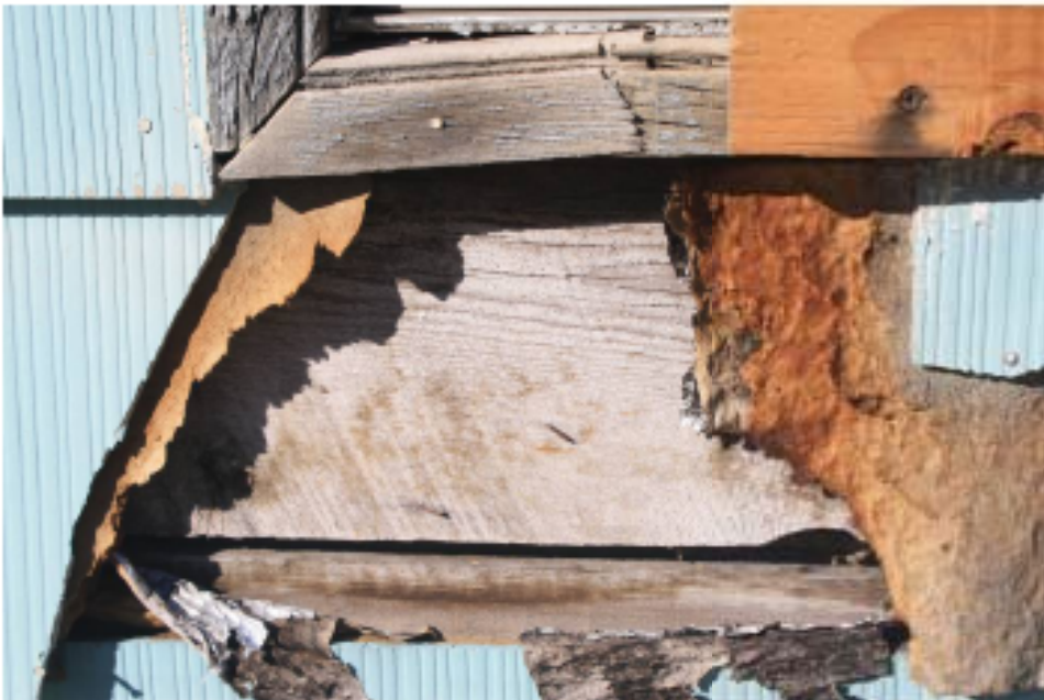
Typical 2" historic wood casing. This particular one is on the kitchen window.
