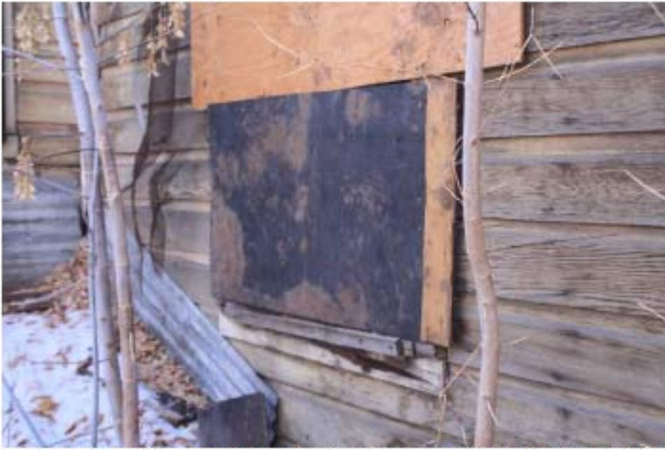
East bedroom window-existing aluminum slider 2'11"W X 2'-0"H and 6'-0" off floor Casing unknown. Historic window 2'-8"W X 5'-0"H 2'-5" off the floor- window style and casing unknown.
