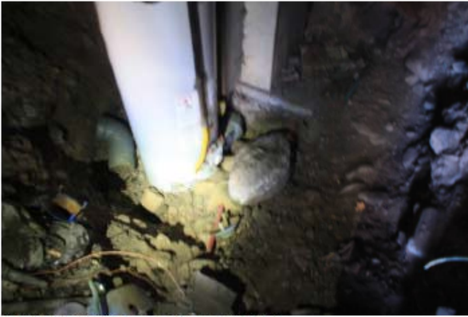
Damage to existing foundation-rubble fallen
