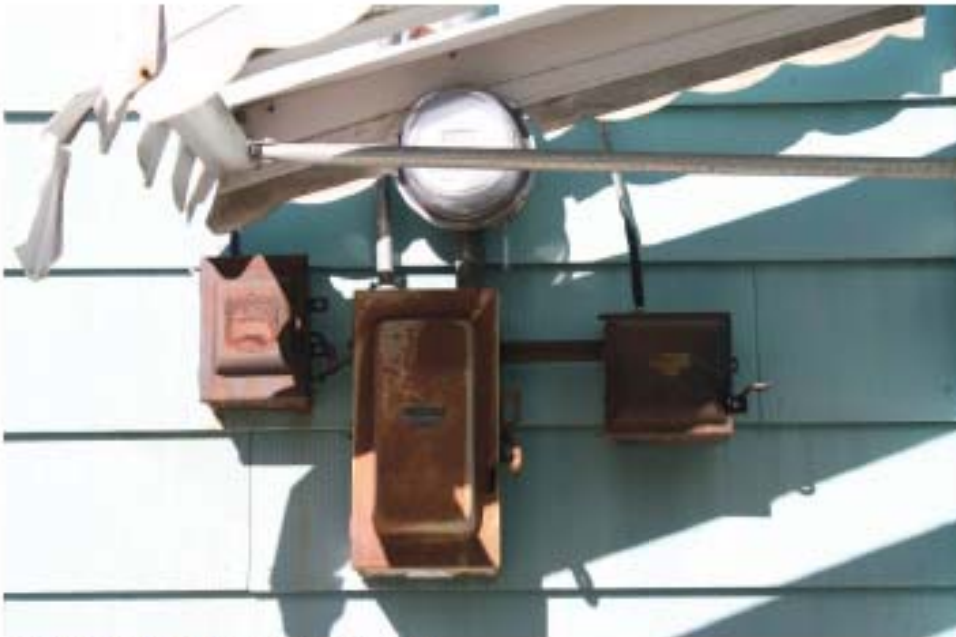
Electrical service-south elevation
