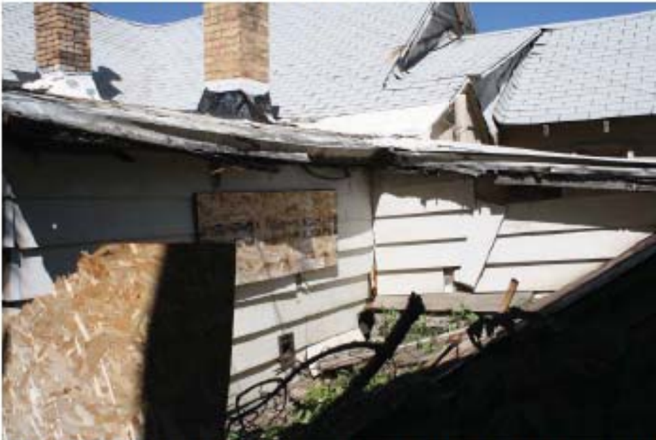
6. South elevation space between mechanical and root cellar. Covered stairs to root cellar to north.
