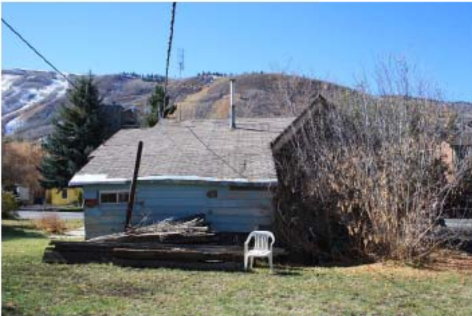
Damage on east-rear portion of shed roof. Roof penetrations.
