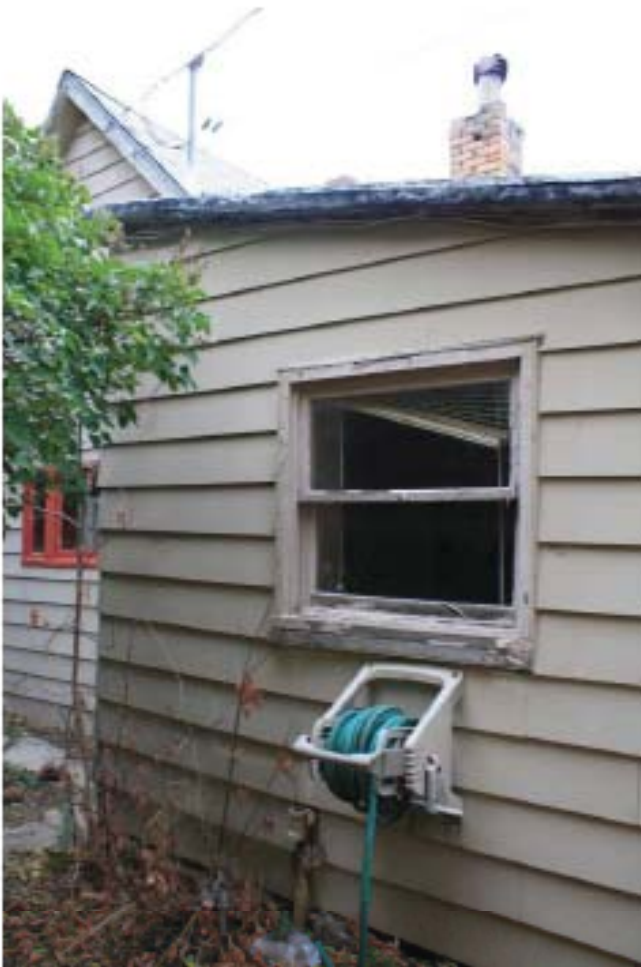
The kitchen window is a wood, single-pane, double hung window. This window is 3'-8 1/2" off the ground and is 3'-0"W X 2'-8"H. The paint is peeling and there is some raw wood. The window detail is similar to above.
