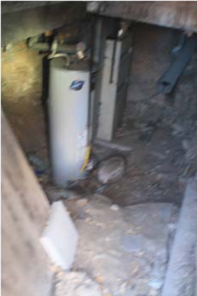
Water heater and furnace in excavated crawl space
