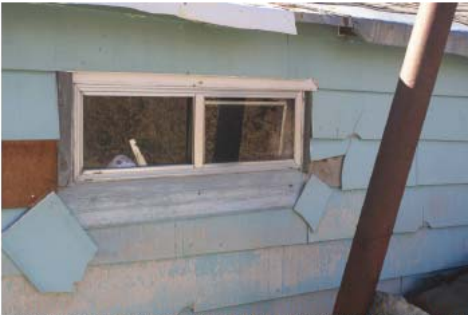
East bathroom aluminum slider 3'-1\"W X 12\"H and 48\" off the ground-patched together casing
