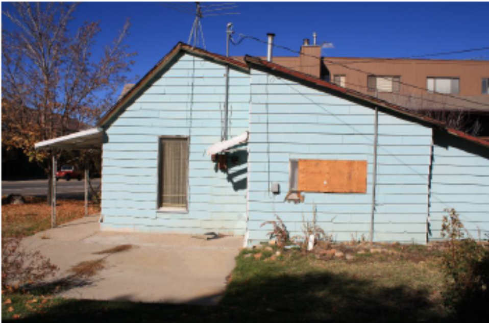
South windows-southwest 2'-7"W X 5'-8"H fixed 24"off slab. Center kitchen window 4'-11"W X 2'-0"H aluminum slider 3'-7" off ground. 2" historic wood casing
