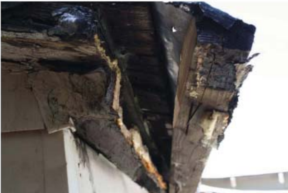
7. Fascia at southeast corner
