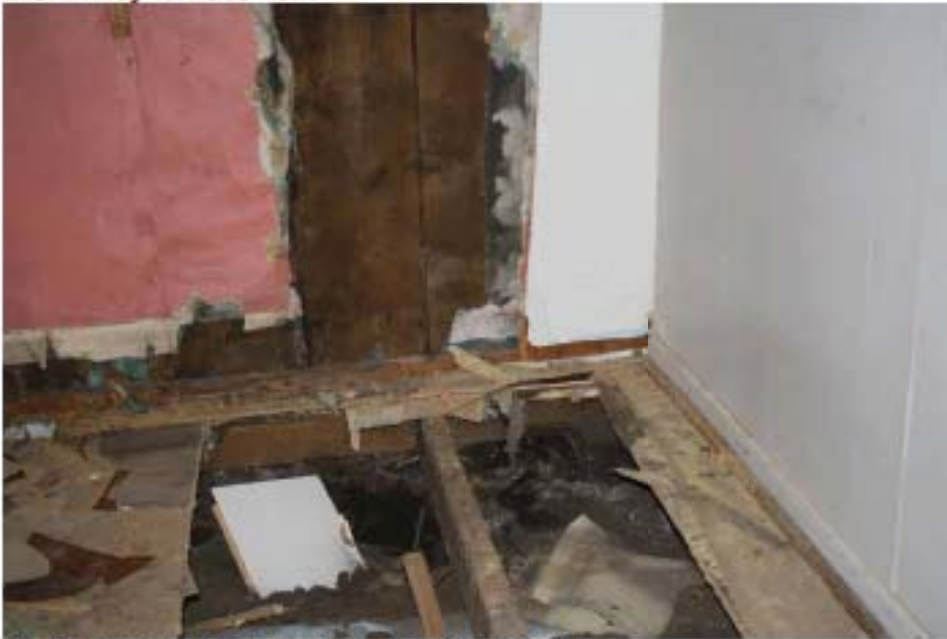
3. Duct work in foreground under floor joist
