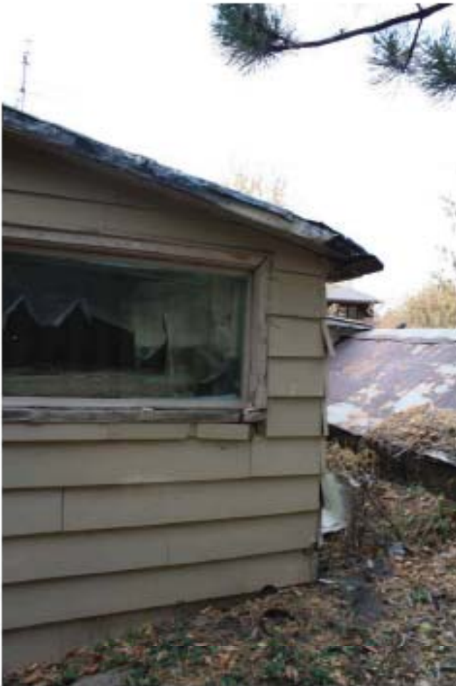
5. Southeast corner mechanical room
