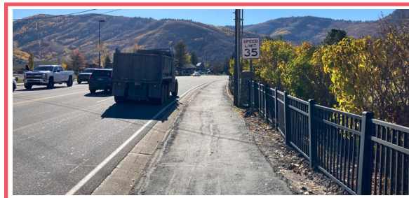
Kearns Blvd Sidewalk | Deficient
