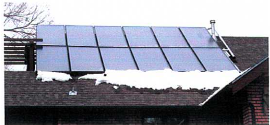
Solar panels visual impacts are minimized
