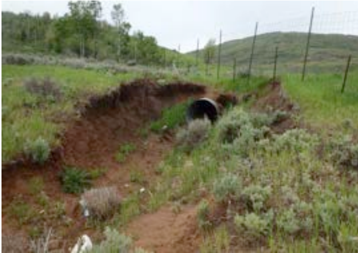
Figure 25: Culvert that carries water from the Highway to the drainage on the East Parcel of the Property. Photopoint 17.
