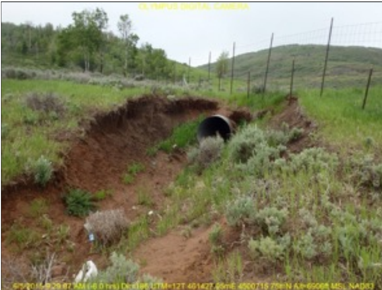
Figure 5. Eroded culvert outflow on the East side of the property degrading soil, vegetation and wildlife conditions
