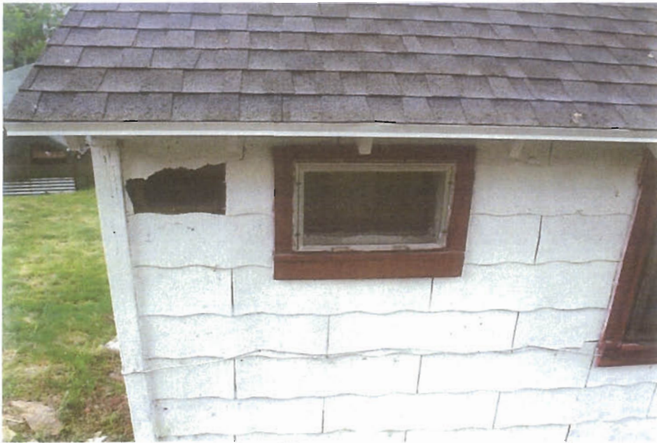
West elevation closet window. Fixed window added later 2'-0" wX14" h. 5'-4" above the ground. 1X4 trim with apron
