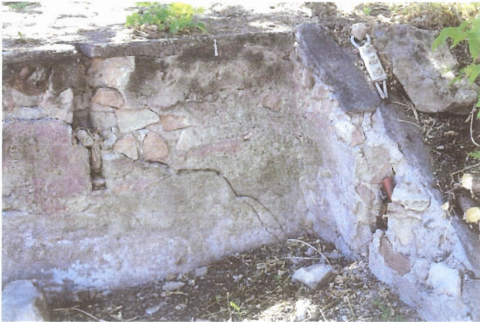
Foundation wall possible cast in floor joist on left center of photo.
