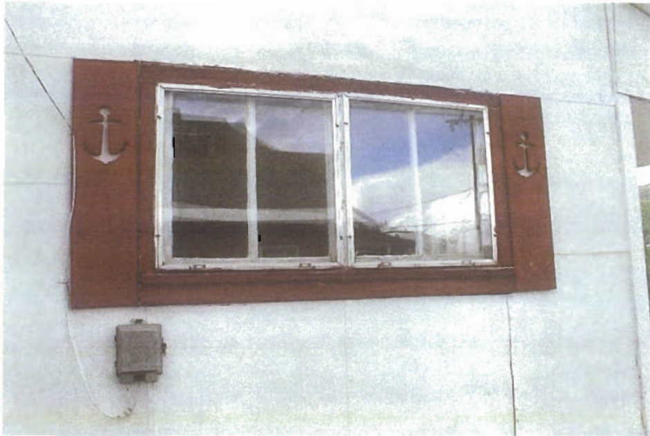
South facing entry window similar to kitchen window 2'-8 1/2" w X 2'-6" h and 4'-3" off the ground. Casement windows are divided in half with 1" muntins. 1X4 trim with apron. This window also replaced another single window.
