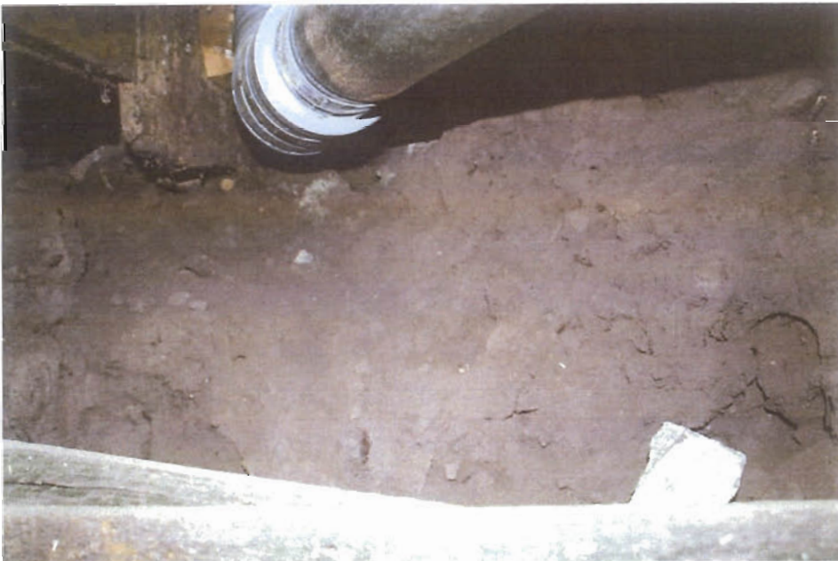
Joists bearing on dirt
