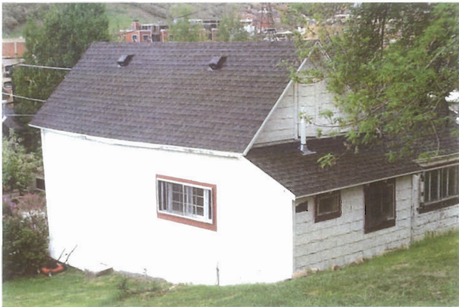
Northwest corner- Roof venting
