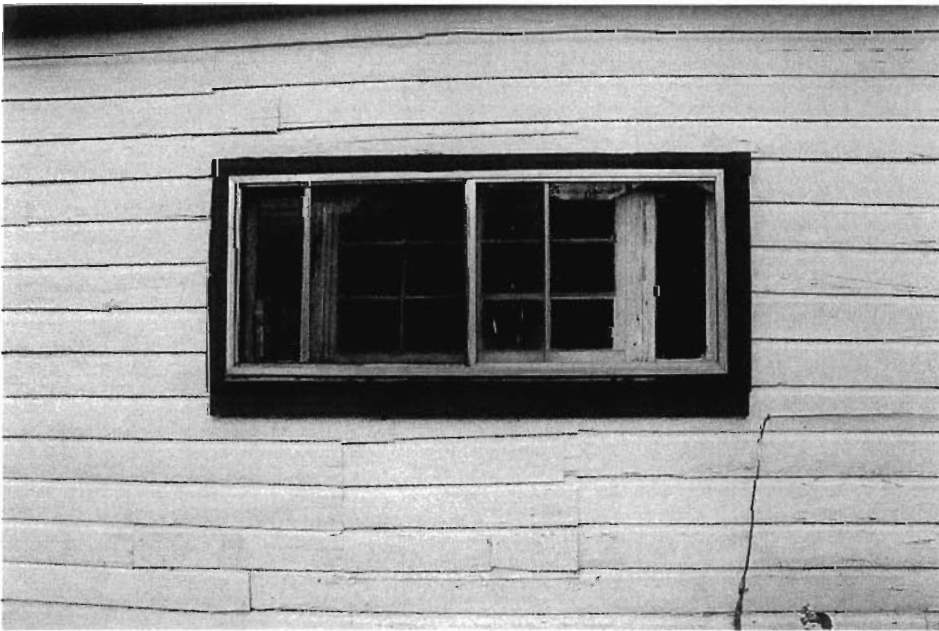
Example of window modification
