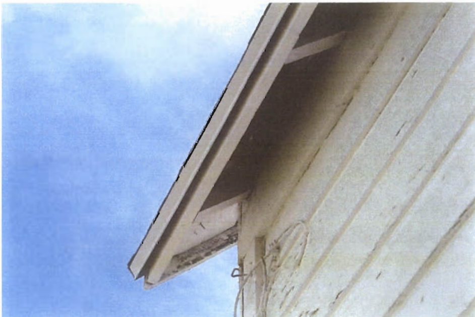
Typical overhang trim profile view 1X10 rim 2X4 rafter overhang and 1X4 fascia
