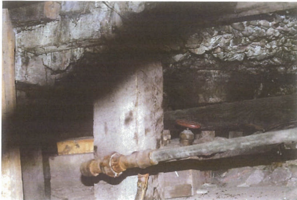
Crawl space excavation, precarious shoring and bearing
