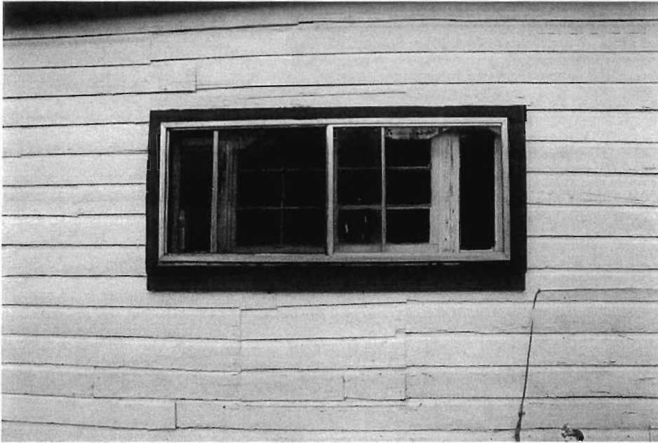
North bedroom exterior Note evidence of old window. Trim 1X4 with apron.
