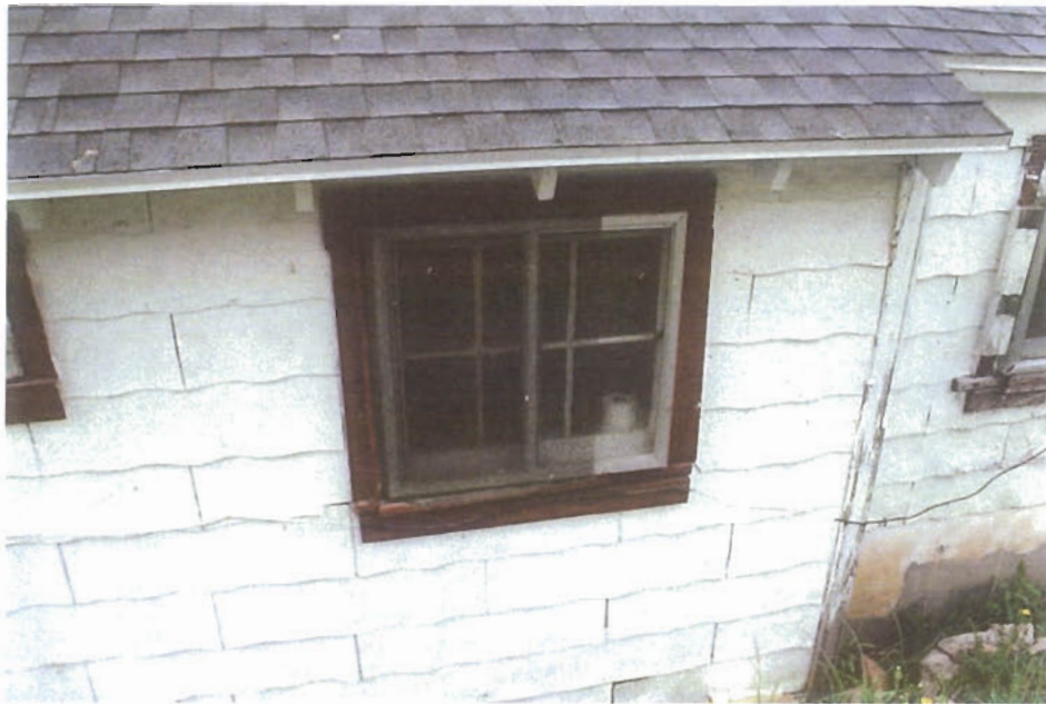
West elevation bathroom window casement 3 over 2 muntin pattern 2'-8" w X 2'-6" h and 4'-1" off the ground. 1X4 trim with apron
