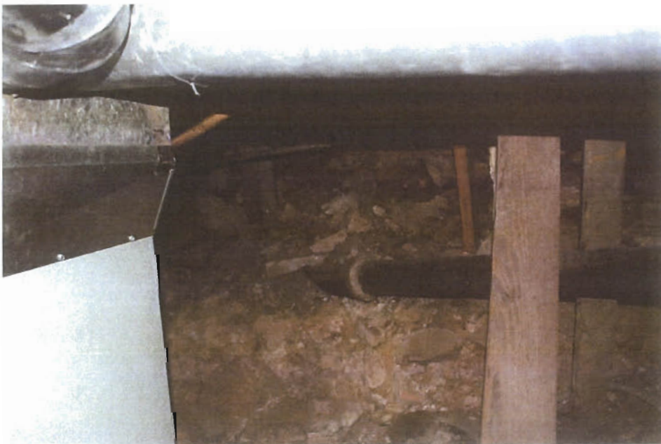
Over excavation for mechanical systems- haphazard shoring of floor joist and sloping floors highlight bearing issues.
