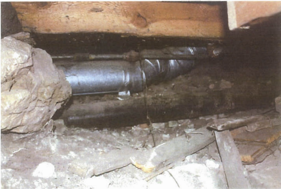
Duct work-crawl space
