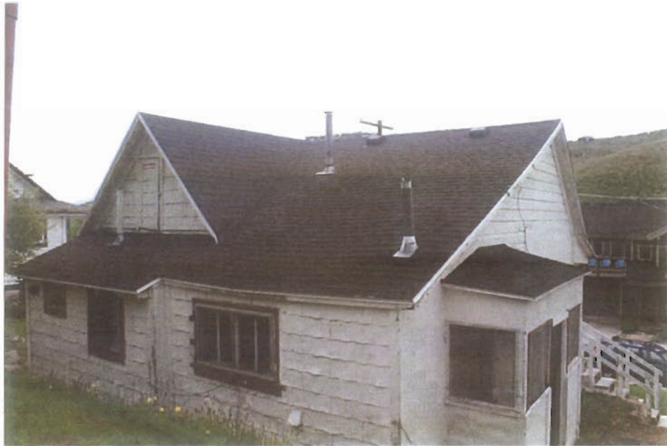
Southwest corner- Sag over kitchen in foreground. Venting
