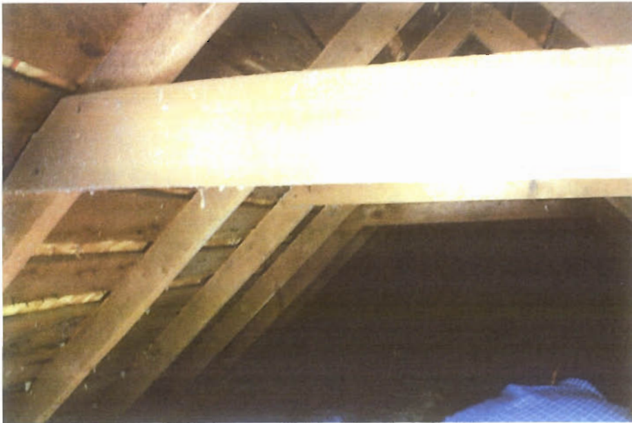
2X4 @ 24" o.c. roof framing and 1X6 collar ties @ 48" o.c. 2x4 ceiling joist @ 48" o.c. + solid 1X12
