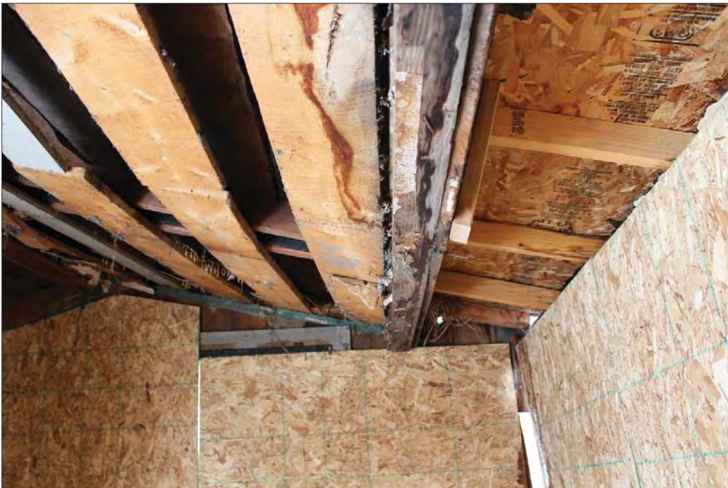
Figure 9. Interior of outbuilding with modern plywood sheathing for support, facing southeast. Note change in roof construction at right side, where the third addition begins. Roof framing and sheathing were added when building was moved.
