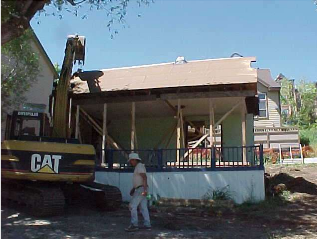
Date of photo: 7/11/2002 Front side of demolition of the roof, porch, internal structure, foundation, and steps.
