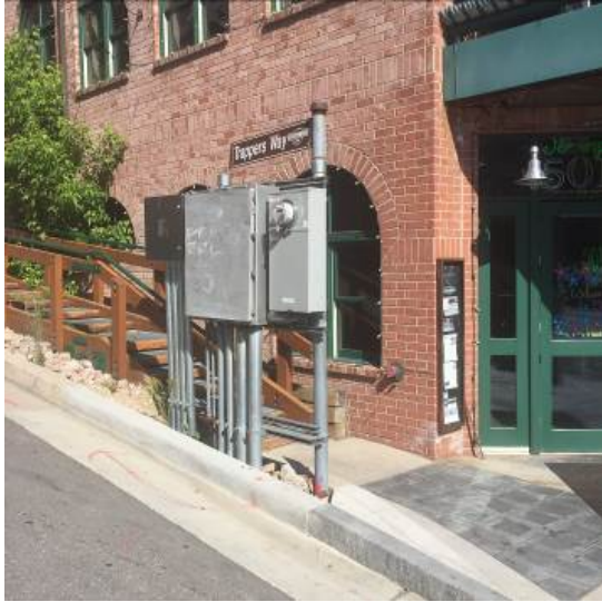
These electrical meters adjacent to 501 Main Street are highly visible and not shielded.
