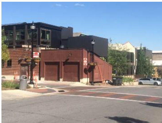
Mechanical equipment at 508 Main Street was installed on the shed roof of the garage and wrapped with the black fencing that shields it from view.
