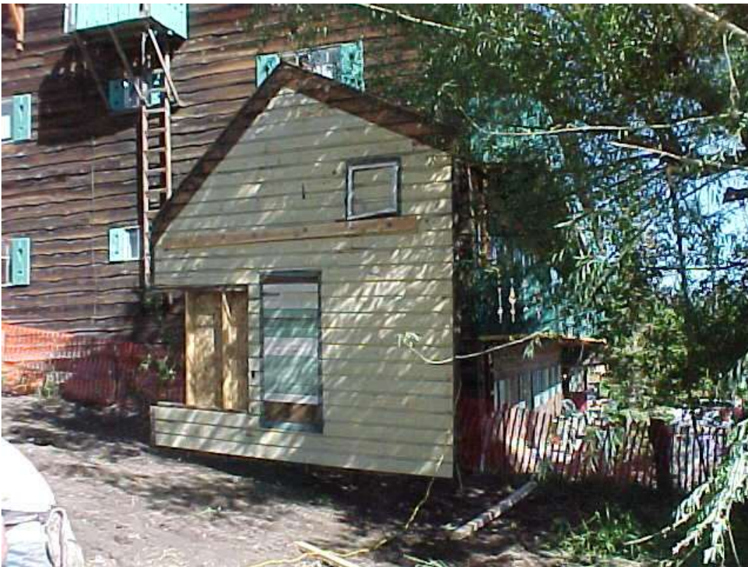
Date of photo: 7/11/2002 Right side panel
