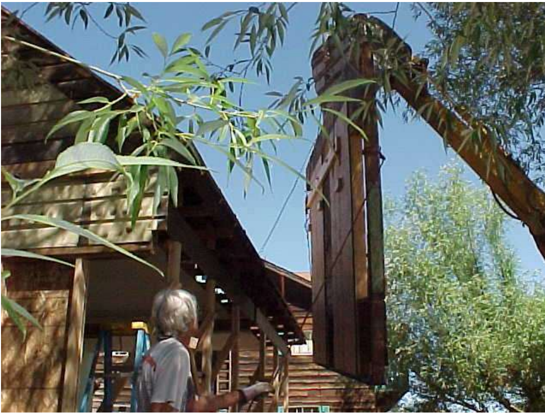
Date of photo: 7/11/2002 Removing half of the front panel of the house that includes the front door and left side window.
