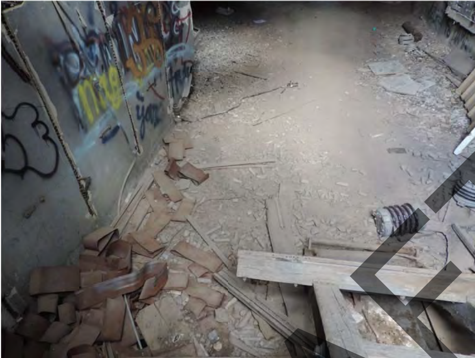
Alliance Tunnel change room interior, detail of mining debris. From west exterior. July 2016.
