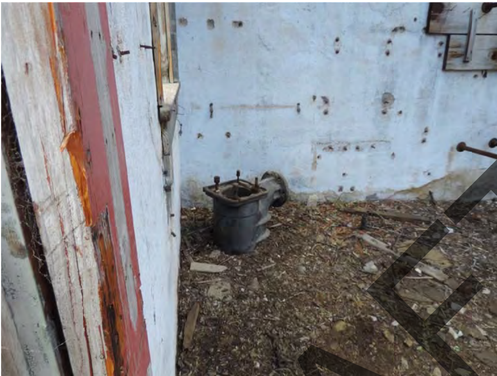
Alliance Tunnel pump house, former water main detail. From southwest exterior. July 2016.
