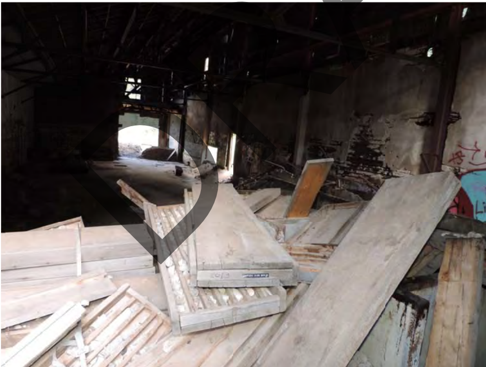
Alliance Tunnel change room interior, detail of mining debris. From west exterior. July 2016.
