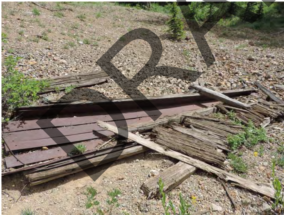
Jupiter Mine Ore Bin, detail of debris. From east. July 2016.
