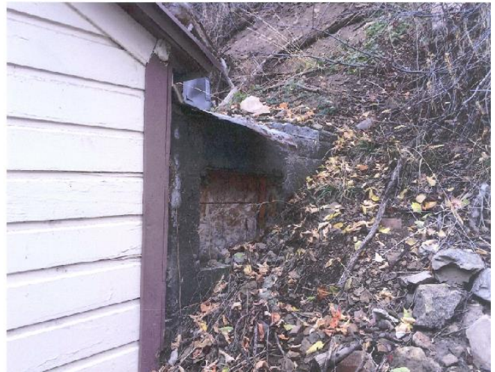
Photo of north elevation. The root cellar is the concrete structure built into the hill.
