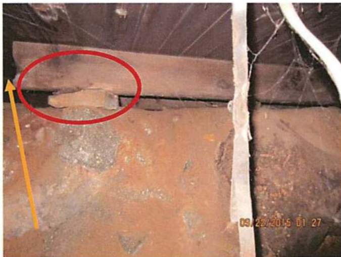
Photo 25 The red circle shows a direct load at the end of a cut off floor joist. The blocking is bearing directly on soils. The yellow arrow shows the removal of a floor joist. The area above is the dining room
