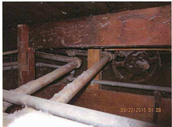
Photo 4 Unsecured gas lines, unknown valves that are not properly maintained or marked
