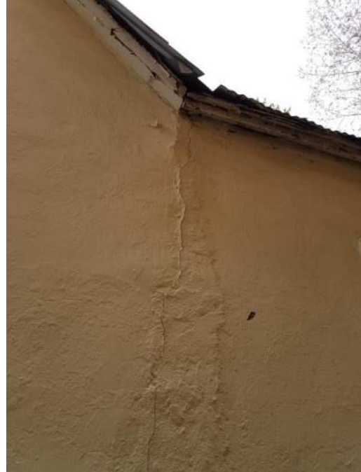
Common defects of the exterior siding materials
