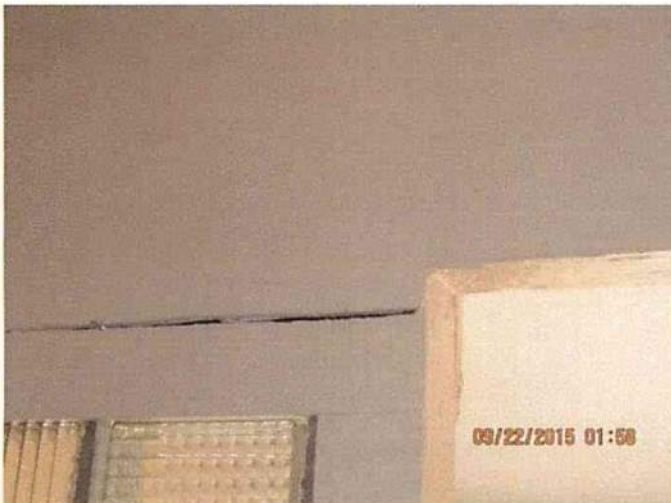
Photo 15 Structural separation in second floor bedroom. Consistent with missing point loads and missing foundation
