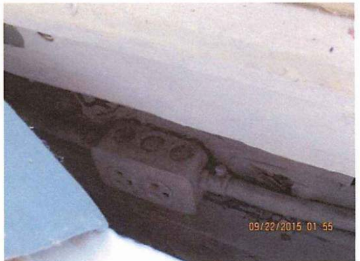
Photo 21 Outlets located under windows that are damaged. Moisture and decay surrounds the electrical outlet
