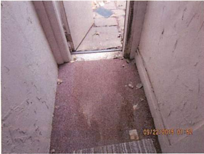
Photo 35 Egress from the back of the dwelling serving 50% of 8 units or 22 occupants cannot be used. Gates are locked to prevent escape and no safe access to the front of the building is provided. Limited egress, direct violation of the fire code for egress requirements for type R-3 buildings and occupant load
