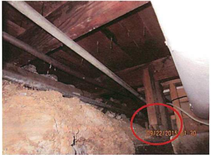
Photo 18 Several shims have been used to level the building. These shims have not been properly installed
