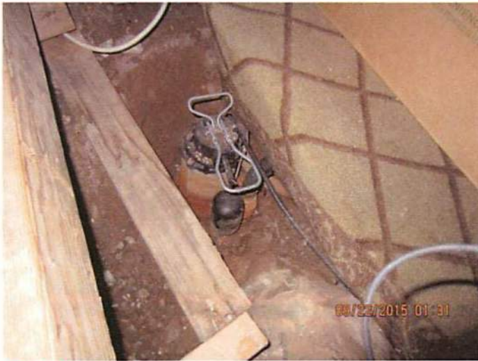
Photo 5 A sump was installed to remove water from the area but was not properly maintained and currently is not in working condition
