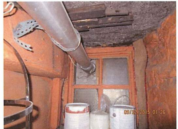
Photo 10 Vent line for hot water heater exceeds the maximum length. Possible carbon dioxide (CO 2 ) concerns. Located in deli
