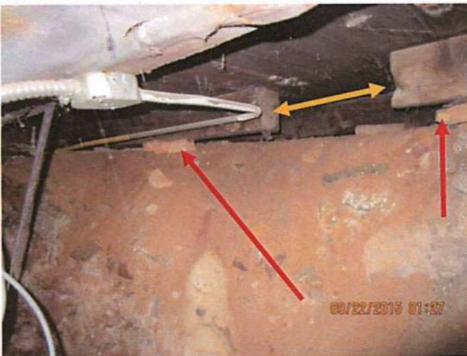
Photo 3 The red arrows show improperly installed shims are blocking to level the floor above. Not permitted on dirt . The yellow arrow shows the removal of floor joist, this is consistent throughout the floor area
