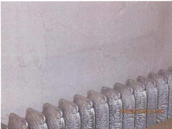
Photo 12 Example of the radiator heating system that uses the boiler to heat the building
