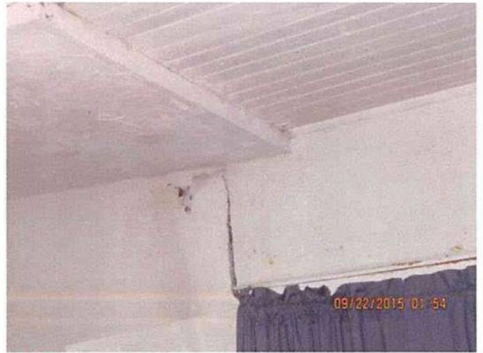
Photo 12 Structural separation in second floor bedroom. Consistent with missing point loads and missing foundation
