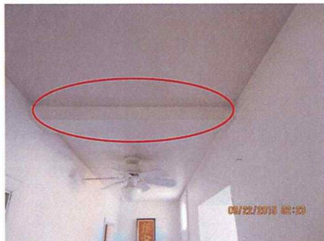
Photo 9 The third level of the structure was added in the 1970's. The addition will need to be evaluated by a structural engineer. The support beam in this photo is missing a point load.
