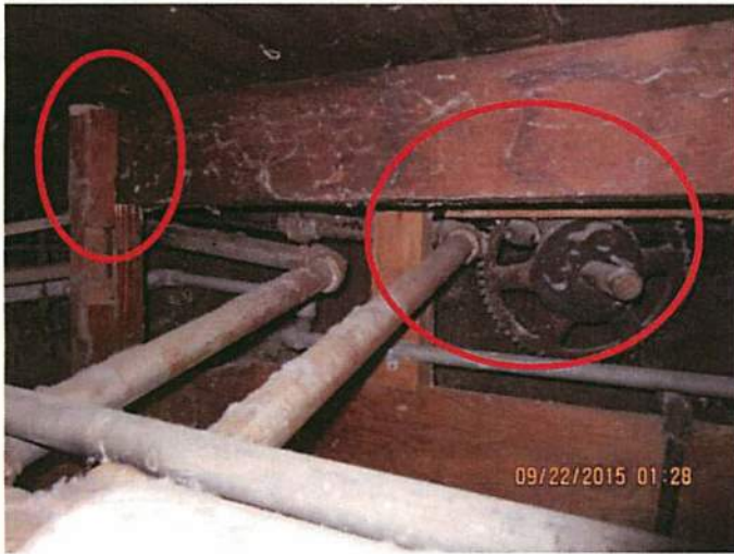
Photo 23 The addition of bracing and shims to prevent settling of the building. Cannot have bearing directly on soils. All bearing is directly on soils. Engineer to justify
