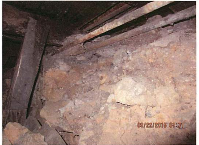
Photo 6 Water lines used for the heating of the building are damaged by decay and deterioration. Erosion and sloughing of the rubble foundation. Severe stability concerns for the structure
