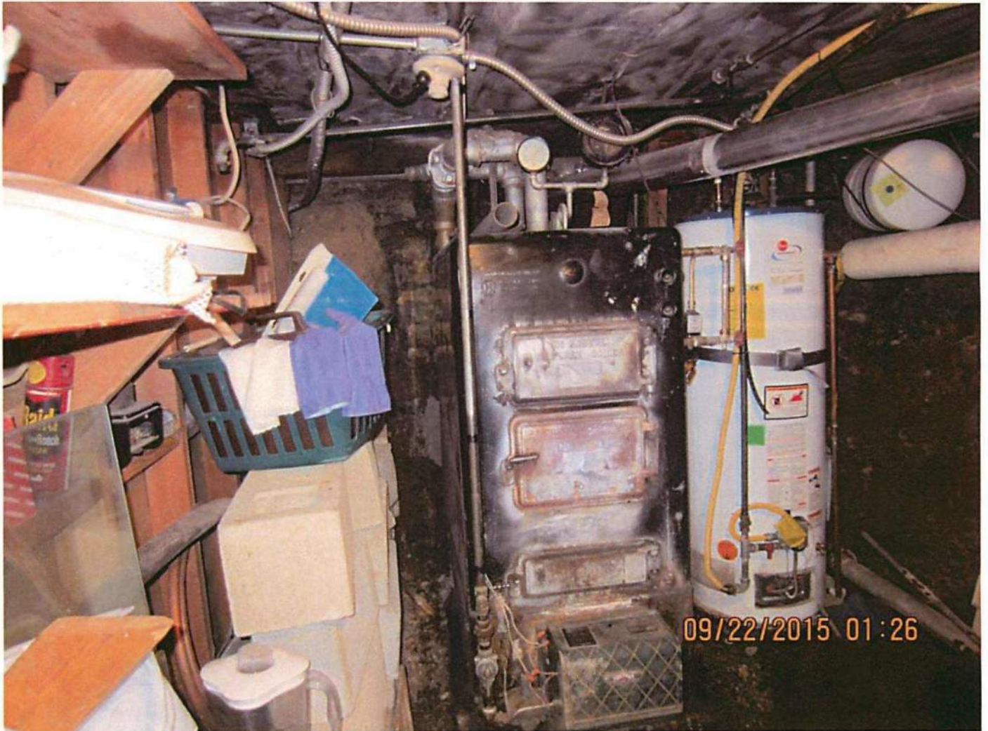
Photo 11 The building is being heated by a 1930's era boiler that has been converted from coal/wood to natural gas. The boiler has no current state boiler inspection tags and required by state law to be inspected annually. It is advised the state boiler be notified for a immediate safety check on the boiler. The gas line that feeds the boiler is unsafe and should be terminated .
