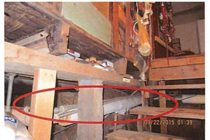
Photo 10 Example of missing foundation under support member. Connection to support from attic 3rd floor
