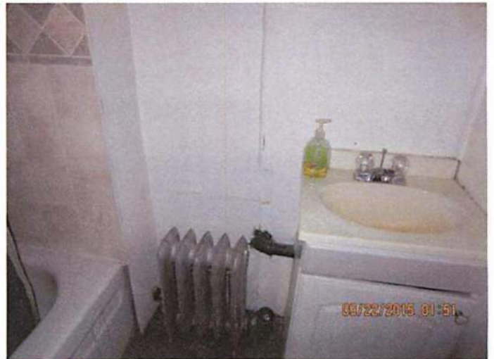
Photo 13 Example of the radiator heating system that uses the boiler to heat the building
