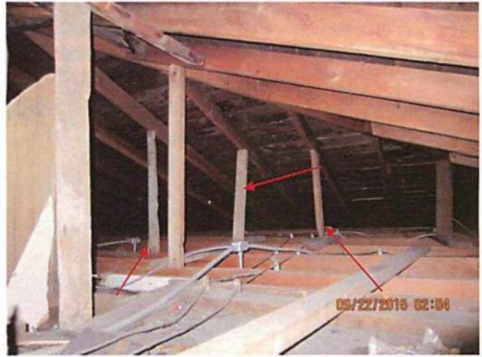
Photo 2 Support members for roof are not adequate for the purpose being served. Engineer to justify
