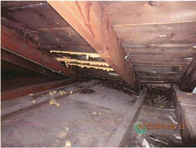
Photo 28 Roof leaks being repaired with a product that is not designed for such use
