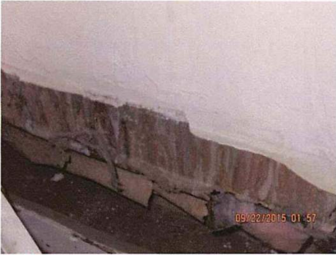
Photo 22 Decay and deterioration noted throughout the building, cause appears to be lack of proper maintenance and infiltration of water from damaged roof
