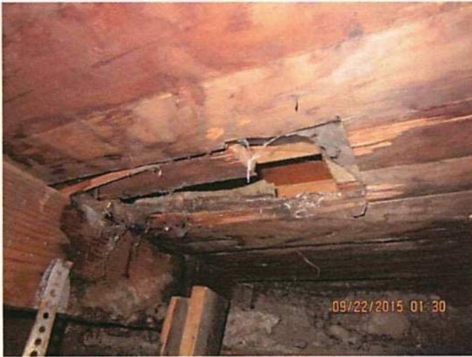
Photo 19 Several shims and braces have been used to level the building. These shims and braces have not been properly installed
