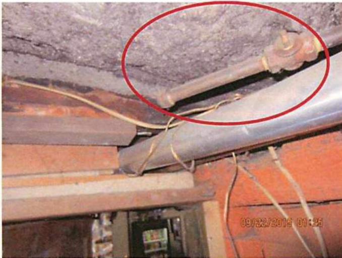
Photo 1 Gas lines that have terminated in hidden rooms that are not properly secured. This room is located in the deli in the front area between entry doors
