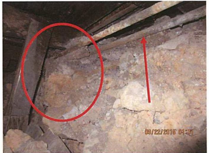
Photo 4 The red circle shows movement of the rubble foundation and decay of the floor joist members resting directly on top of the rubble. The red arrow shows decay of water lines used to heat the structure
