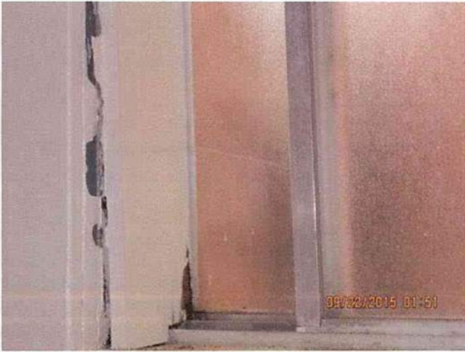
Photo 11 Noted settling around the bathroom window on the second floor. Consistent with improperly installed support beam on third floor.
