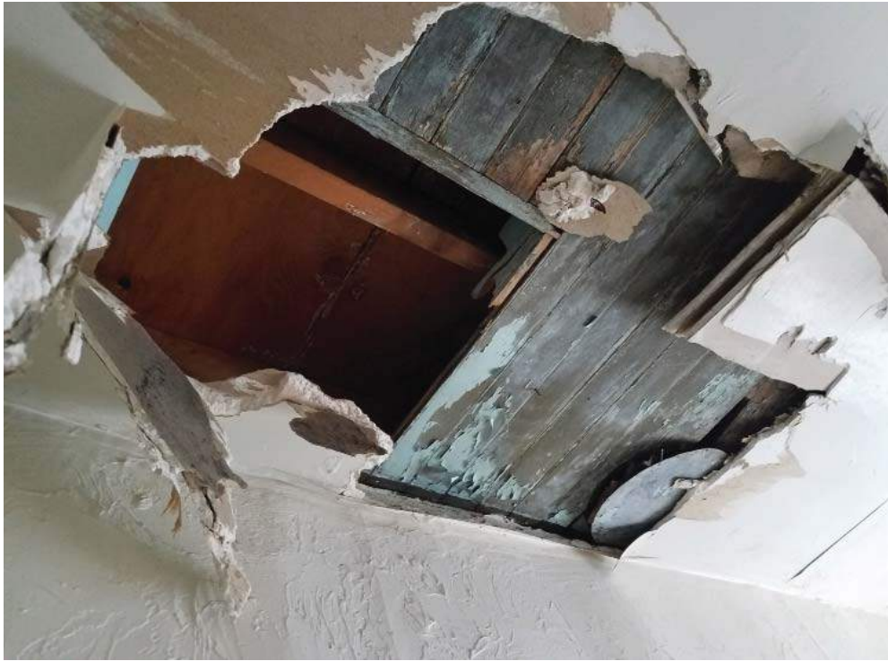
91 - L2 - Sagging Ceiling in Bedroom 206
