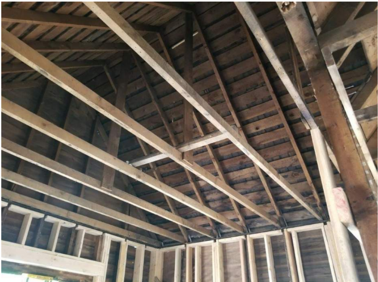
Below: Roof structure of the historic house. Note the intersection of the gable ell to the side-gable of the original hall-parlor house form in the upper right hand corner.
