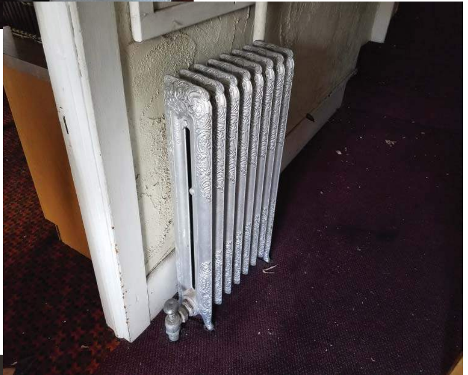
78 - L1 - Typical Radiator
