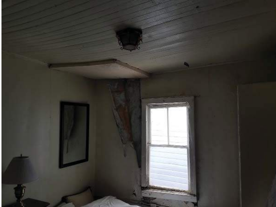
92 - L2 - Sagging Ceiling in Bedroom 207
