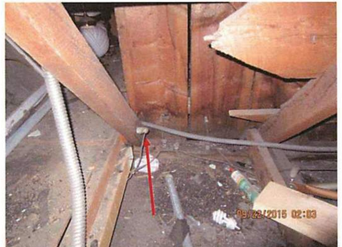
Photo 16 Knob and tube wiring located throughout the attic area
