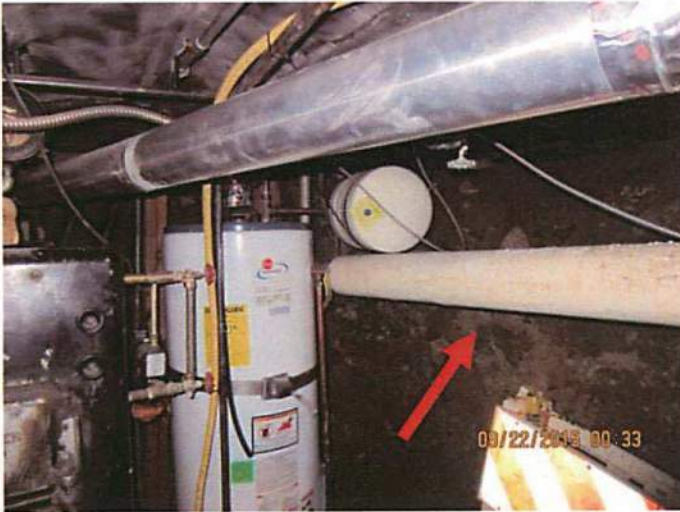
Photo 1 The structure has no concrete or stable foundation. The foundation consists of rubble, dirt and loose stone matter.
