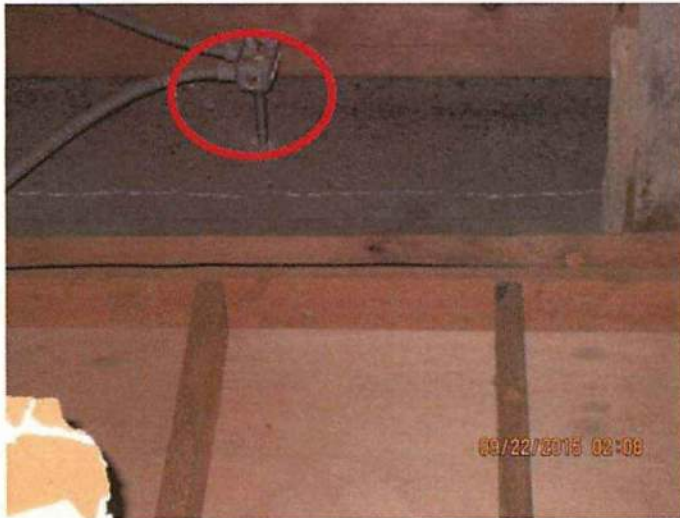
Photo 18 Open electrical boxes noted throughout the building. Electrocutation hazard, fire hazard. Located in attic
