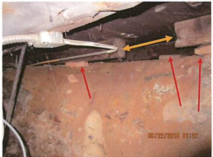
Photo 26 The addition of bracing and shims to prevent settling of the building. Cannot have bearing directly on soils. All bearing is directly on soils. Engineer to justify
