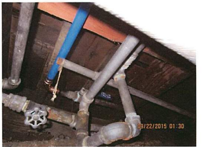
Photo 8 Improperly installed plumbing repairs. Ends not properly capped. Copper to galvanized requires a brass coupler
