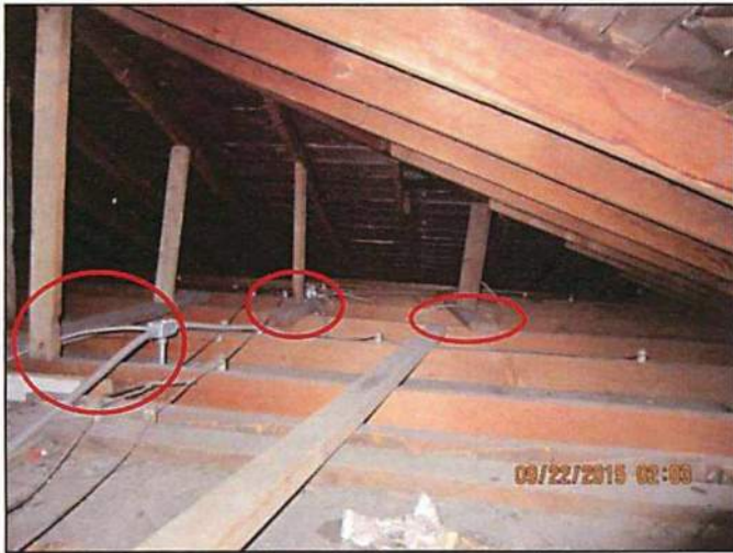
Photo 1 The structural members supporting the roof are not properly installed and are not plumb. Excessive load could cause the members to fail
