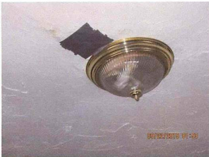
Photo 26 Tape being used to cove water damage next to electrical outlet that feeds light
