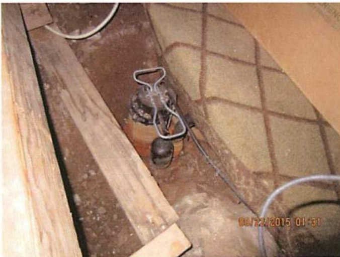
Photo 7 A water/trash pump is located directly below photo 6, the pump is not in working condition
