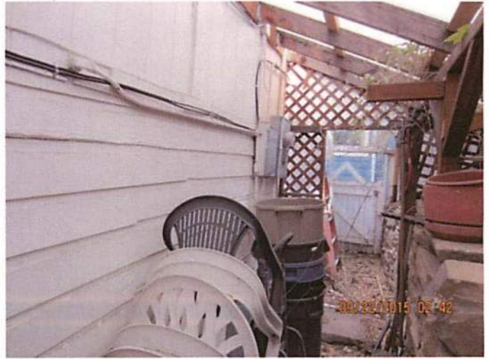
Photo 36 Egress path rear of building. No access to safe location
