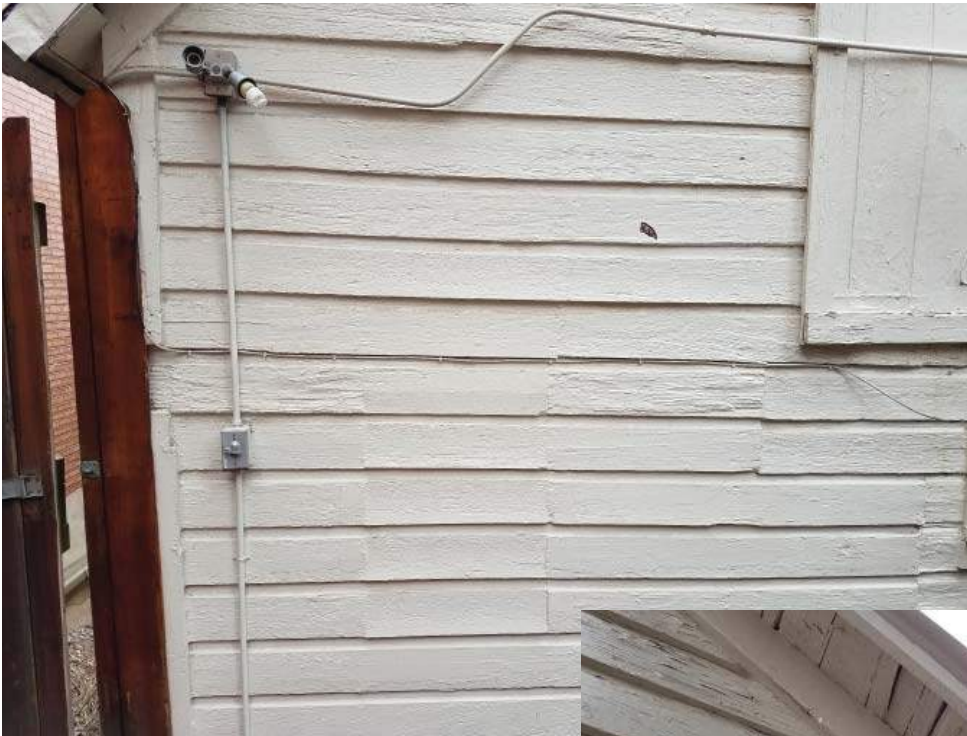
22 - Patched Siding on Wall
