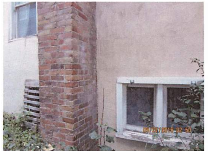
Photo 40 Egress path from other side of building. No safe access to main street
