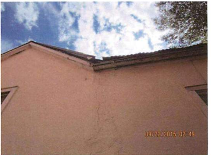
Photo 33 Structural concerns possibly related to the drainage from the roof
