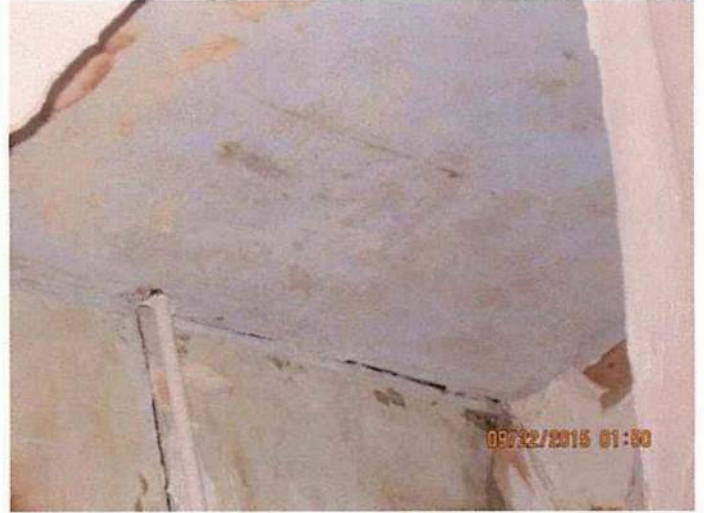
Photo 25 Decay and deterioration noted throughout the building, cause appears to be lack of proper maintenance and infiltration of water from damaged roof
