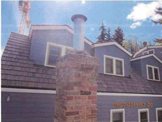
Photo 1 The chimney shows signs of decay and instability. To be removed or evaluated by a structural engineer
