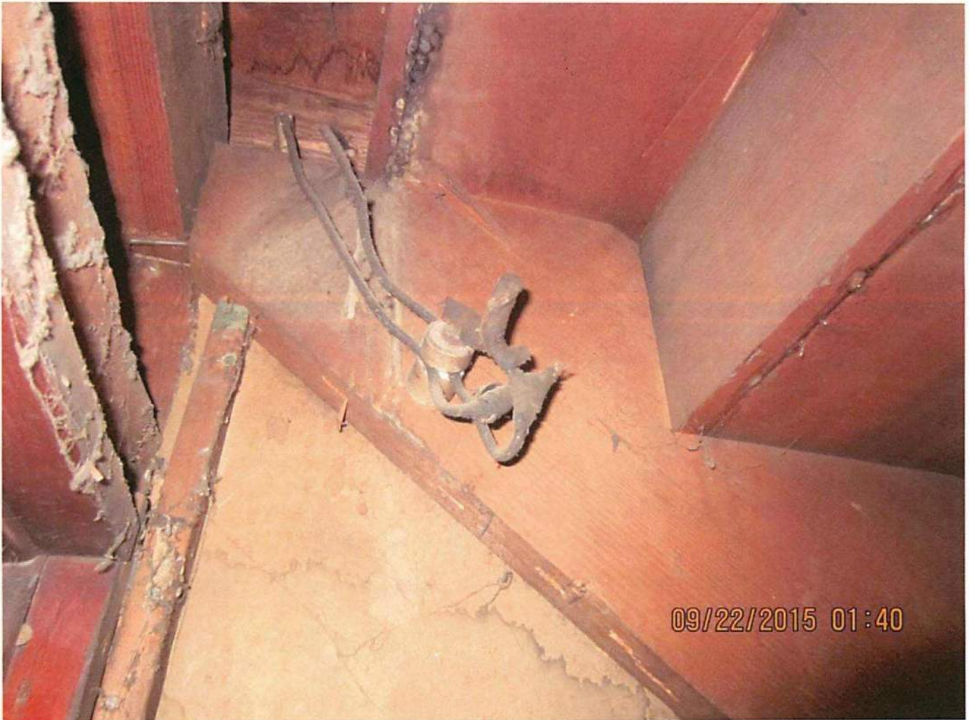
Photo 14 Knob and tube electrical is located throughout the building. Knob and tube type wiring is classified as a possible health, life and safety concern if not properly maintained. It is common practice and a requirement of the electrical code to remove knob and tube wiring if any portion of the building is upgraded with newer electrical wiring. The building shows numerous upgrades in wiring and electrical upgrades, such as electrical panels, breakers, outlets and lighting. The knob and tube may not be able to support the current electrical upgrades in a safe manner and may be a fire concern. An electrical engineer needs to evaluate the electrical for the entire building before the electricity is turned on.
