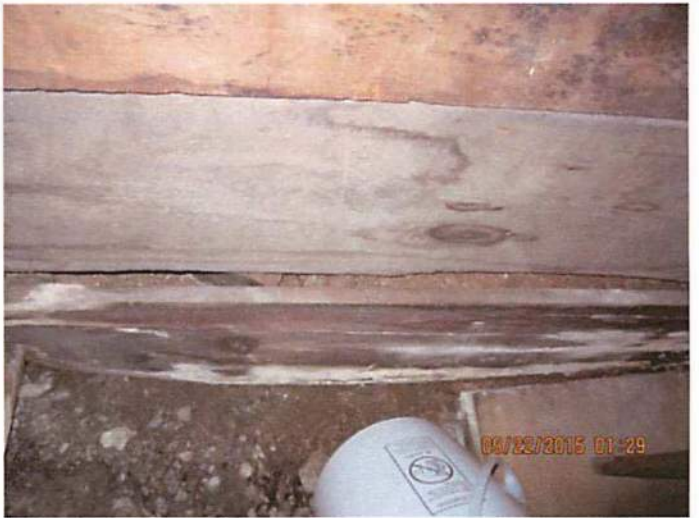
Photo 8 Wood backing being used to prevent rubble from filling the storage area. Backing is failing and decayed . Serious mold and water concerns
