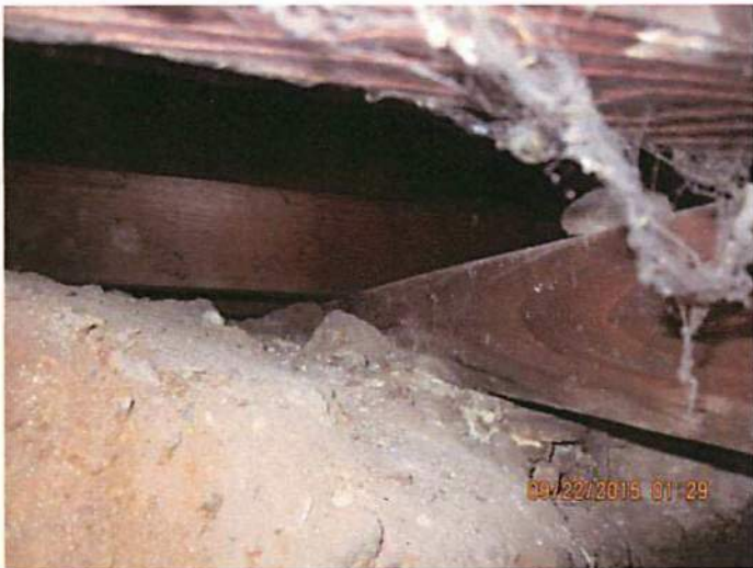
Photo 7 The floor joist of the structure are resting directly on top of dirt and rubble. Not permitted under building codes
