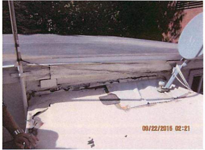
Photo 29 Roof appears to have been recently repaired but some areas are damaged and show signs of possible water infiltration
