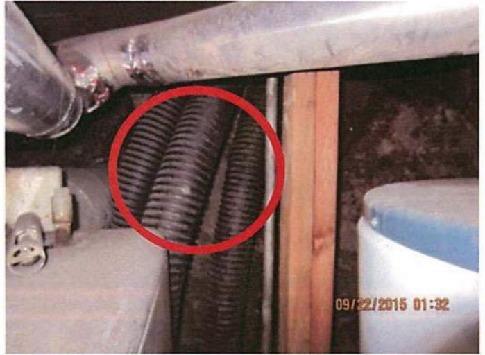
Photo 6 A drainage system was improperly installed and permitted to drain directly on top of the dirt floor causing decay, mold and erosion
