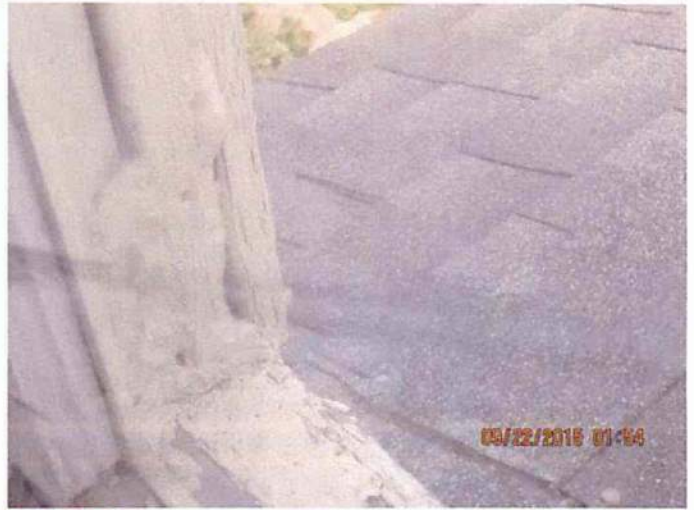
Photo 23 Decay and deterioration noted throughout the building, cause appears to be lack of proper maintenance and infiltration of water from damaged roof
