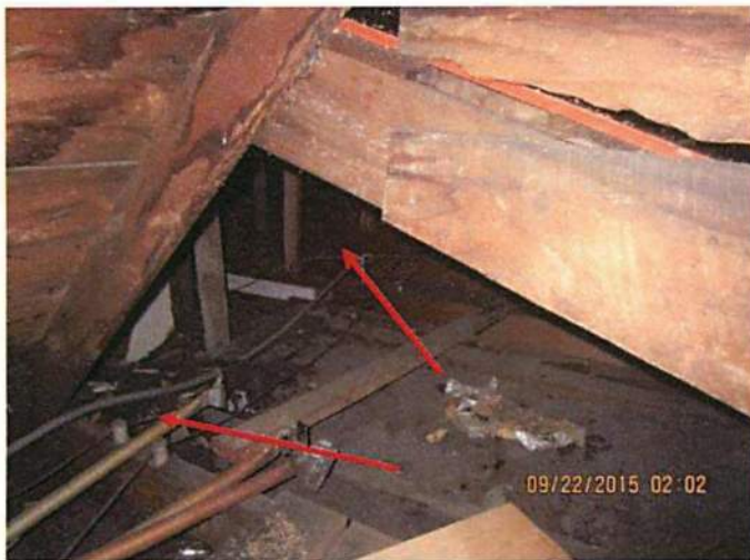
Photo 15 Knob and tube wiring located throughout the attic area
