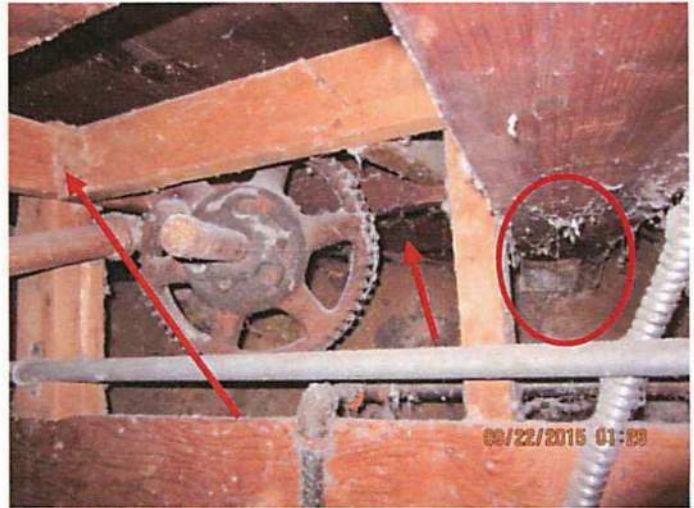
Photo 22 Floor joist bearing directly on dirt. Shims and bracing added for support. Improperly installed
