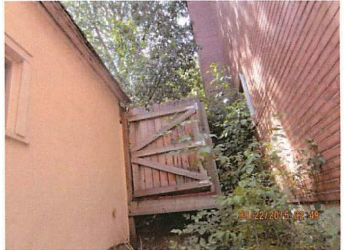
Photo 38 Side view of non-usable egress from rear of building
