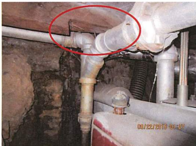
Photo 27 Over notching of floor joist. Area above, dining room
