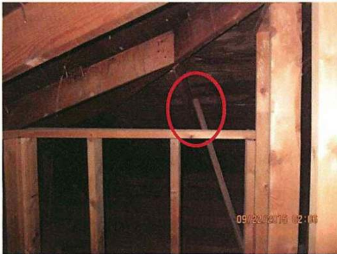
Photo 5 Support member not properly fastened
