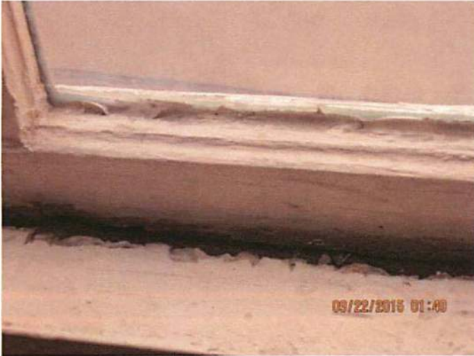
Photo 17 Several windows on the second floor have separated and have been nailed shut. This is consistent with wacked and warped walls due to structural stability of the building
