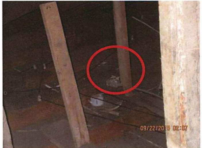
Photo 19 Open electrical boxes noted throughout the building. Electrocutation hazard, fire hazard. Located in attic
