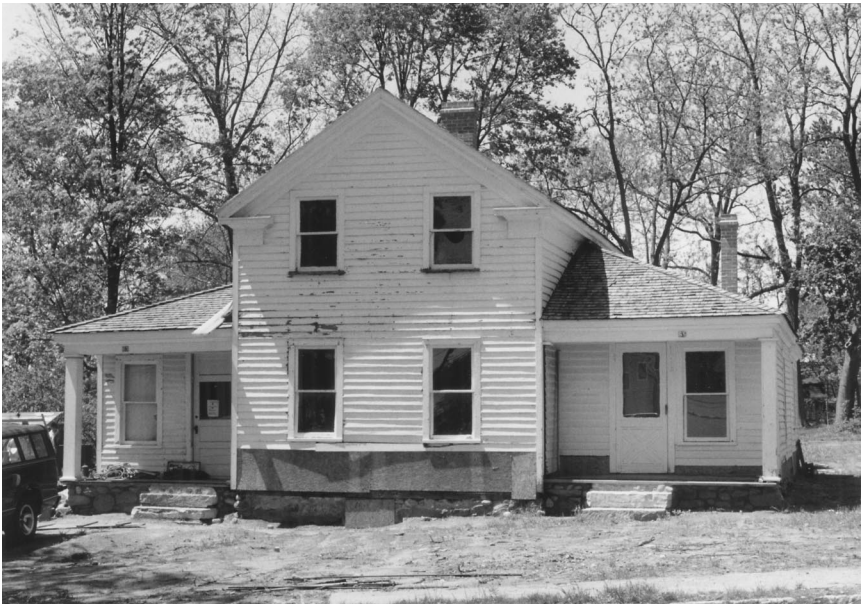
Fig. 9. The James and Ellen G. White house under restoration (2000). Photograph taken by Michael S. Nassaney.
