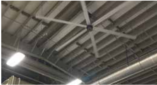
Fan reduces stratification of air
