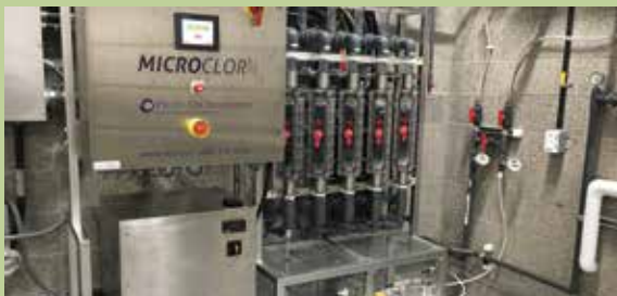
On-site chlorine generation
