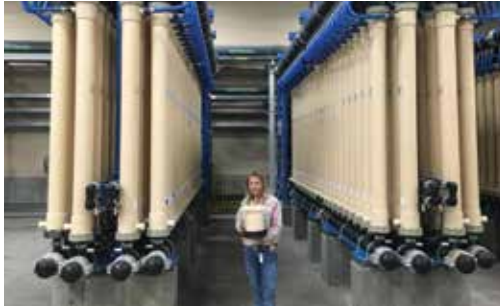
Quinns Junction WTP microfilters
