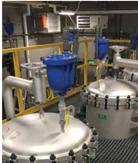
Creekside WTP filters
