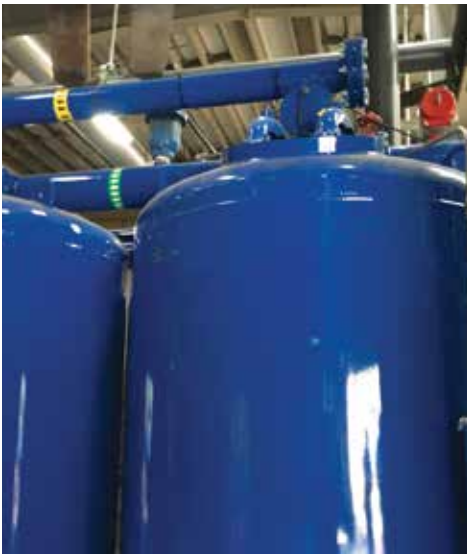
Quinns Junction WTP manganese filters
