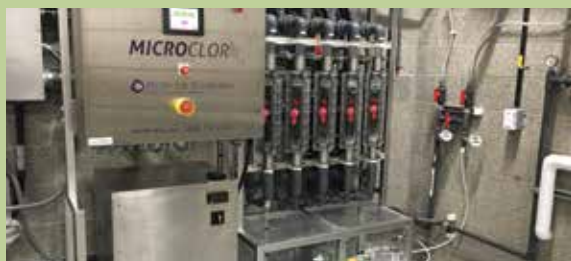
On-site chlorine generation
