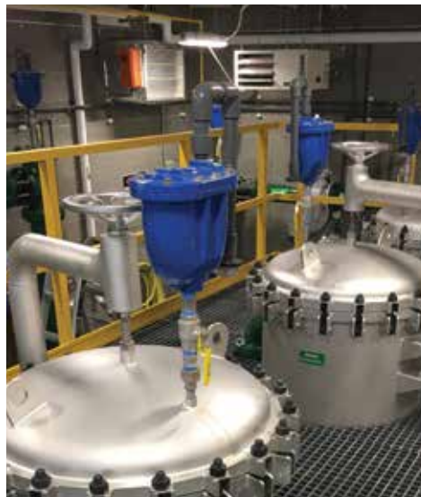
Creekside WTP filters
