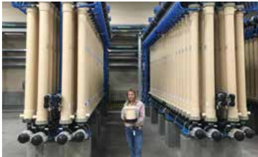
Quinns Junction WTP microfilters
