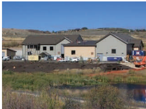
Quinn's Junction Water Treatment Plant
