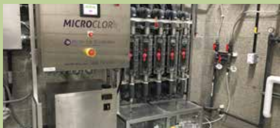
On-site chlorine generation
