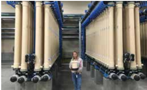
Quinns Junction WTP microfilters
