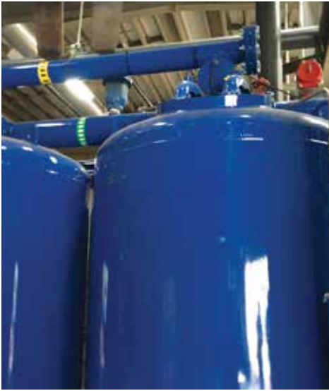
Quinns Junction WTP manganese filters
