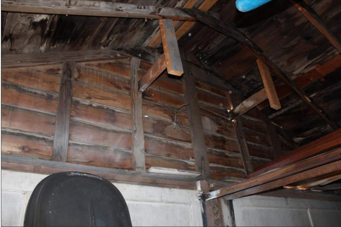
Figure 9. Interior of south gable end of garage at 1503 Park Avenue, 2018, view facing south.
