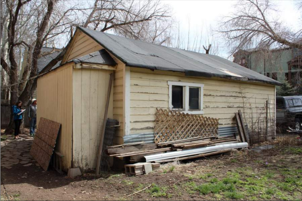
Figure 7. North and west sides of garage at 1503 Park Avenue, 2018, view facing southeast.
