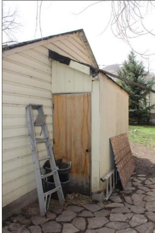
Figure 6. Ca. 1995 shed-roofed addition on north side (rear) of garage at 1503 Park Avenue, 2018, view facing west.
