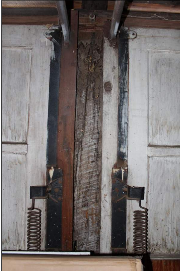
Figure 11. Door-opening and bracing hardware on original garage doors at 1503 Park Avenue, 2018, view facing south.
