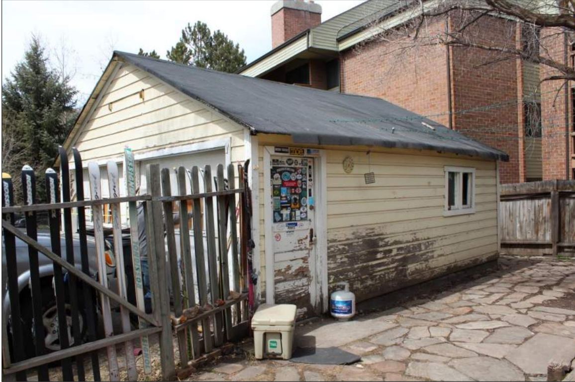
Figure 5. South and east sides of garage at 1503 Park Avenue, 2018, view facing northwest.
