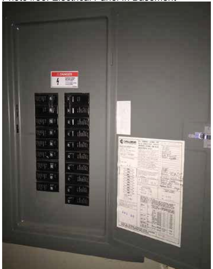
Photo #53: Electrical Panel In Basement
