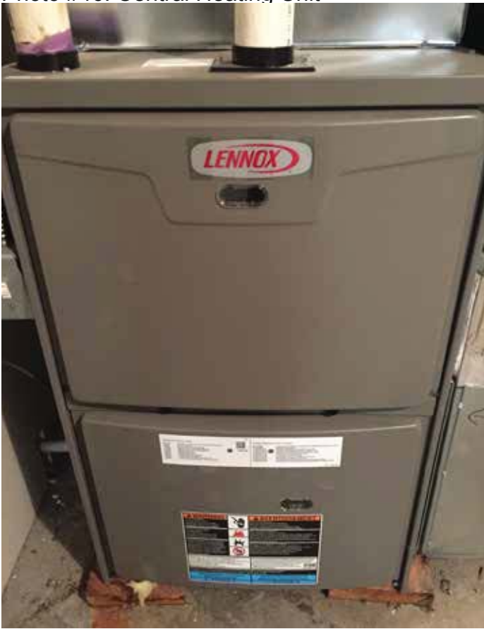
Photo #46: Central Heating Unit
