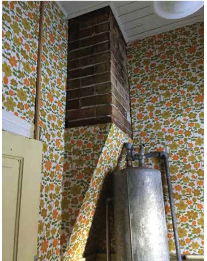
Photo #24: Chimney Within Bathroom
