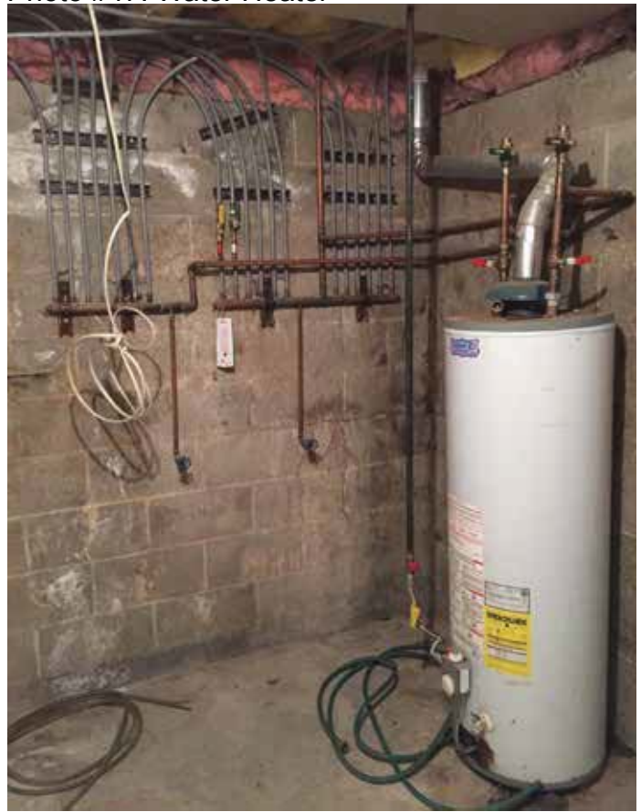
Photo #47: Water Heater
