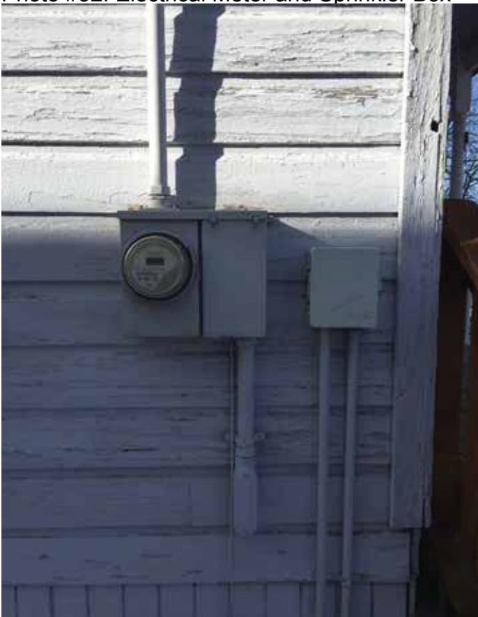
Photo #52: Electrical Meter and Sprinkler Box
