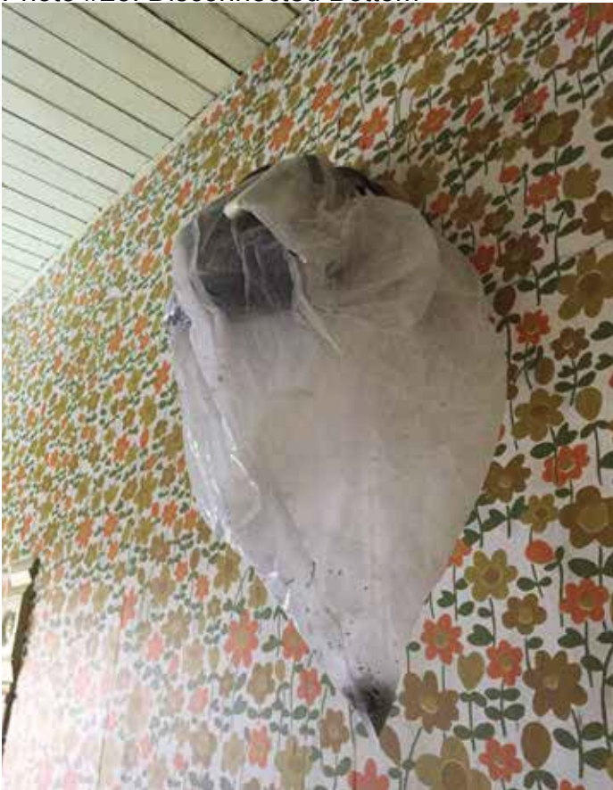
Photo #25: Disconnected Bottom
