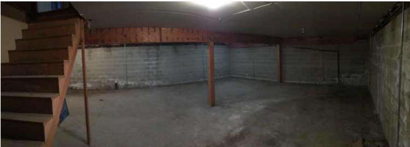
Photo of the interior of the basement. Note the signs of efflorescence on the walls. The heavy timber framing is new and was likely installed when the basement was constructed.
