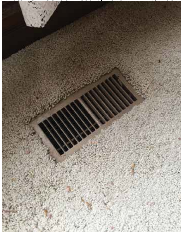
Photo #51: Central Heating Vent In Dining Room
