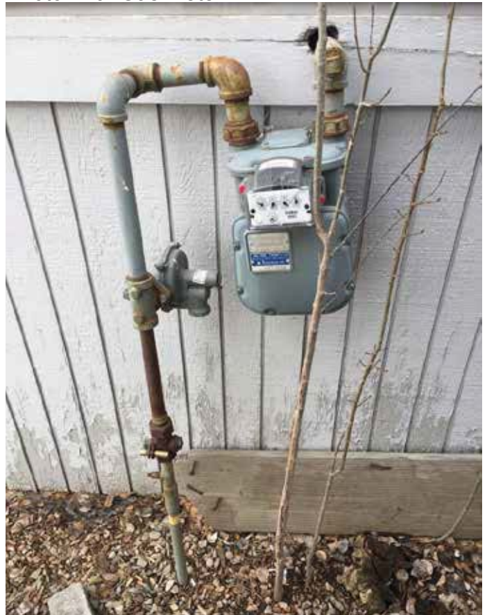
Photo #49: Gas Meter
