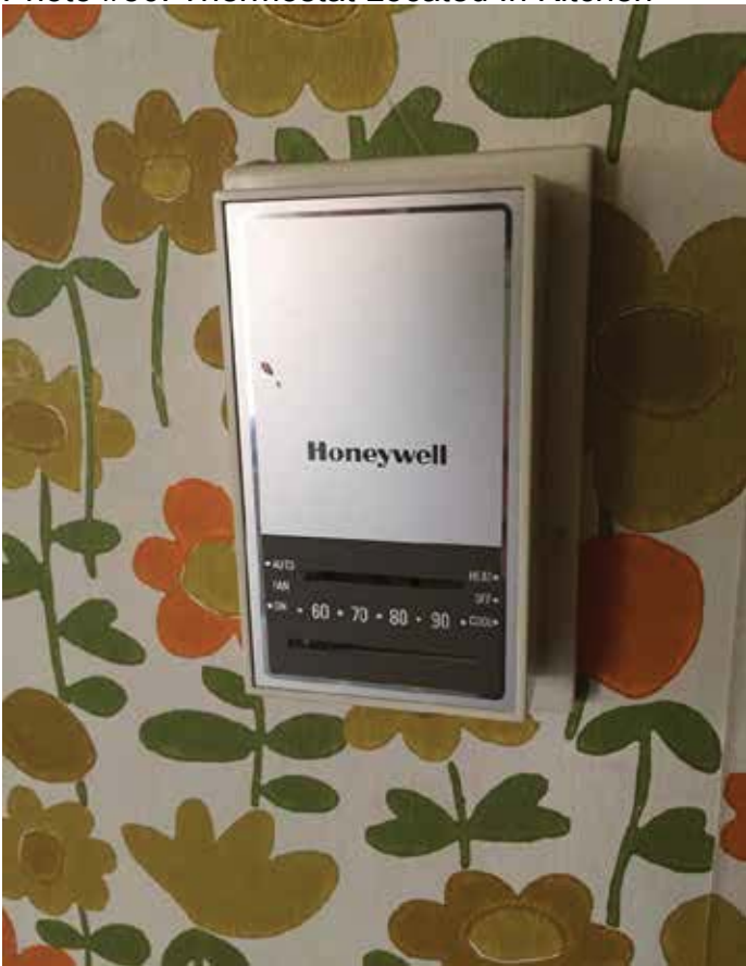
Photo #50: Thermostat Located In Kitchen
