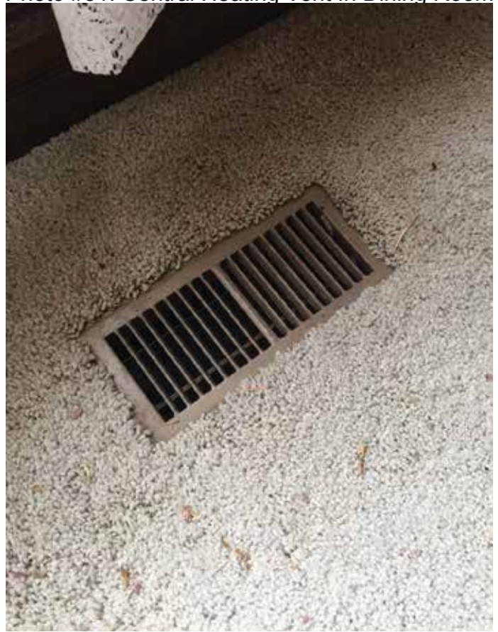
Photo #51: Central Heating Vent In Dining Room
