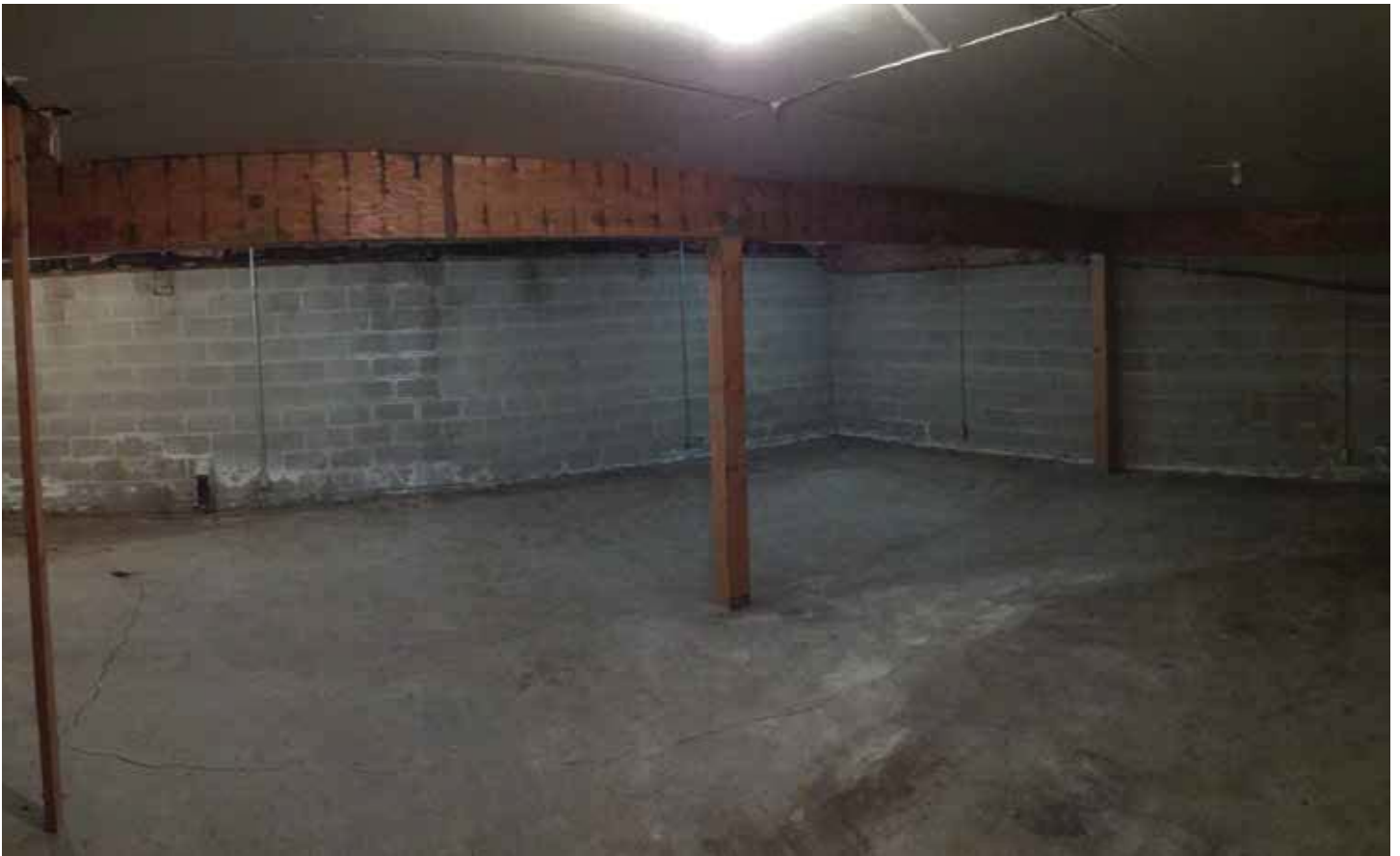
Photo #10: Basement Level Slab With New Beam and Columns Holding Main Level Floor
