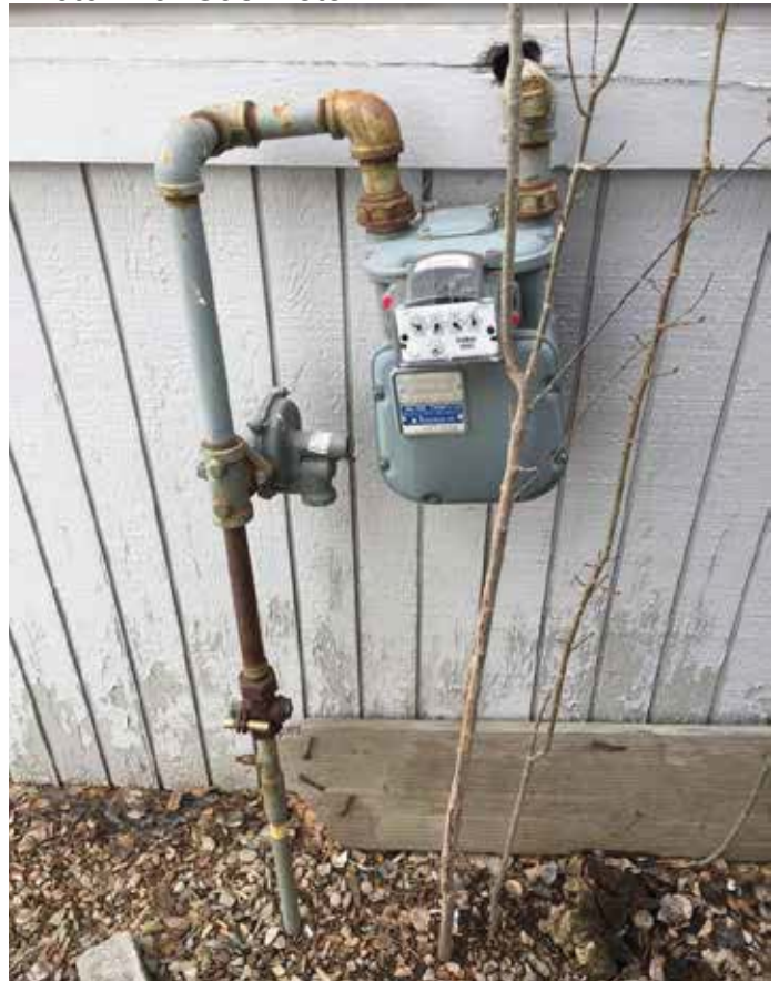
Photo #49: Gas Meter
