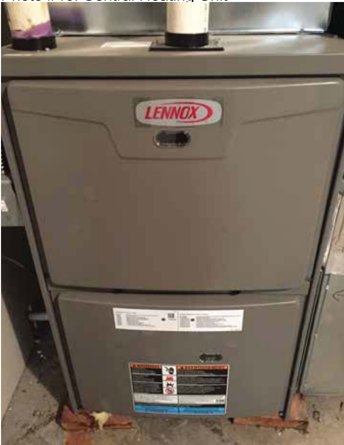
Photo #46: Central Heating Unit
