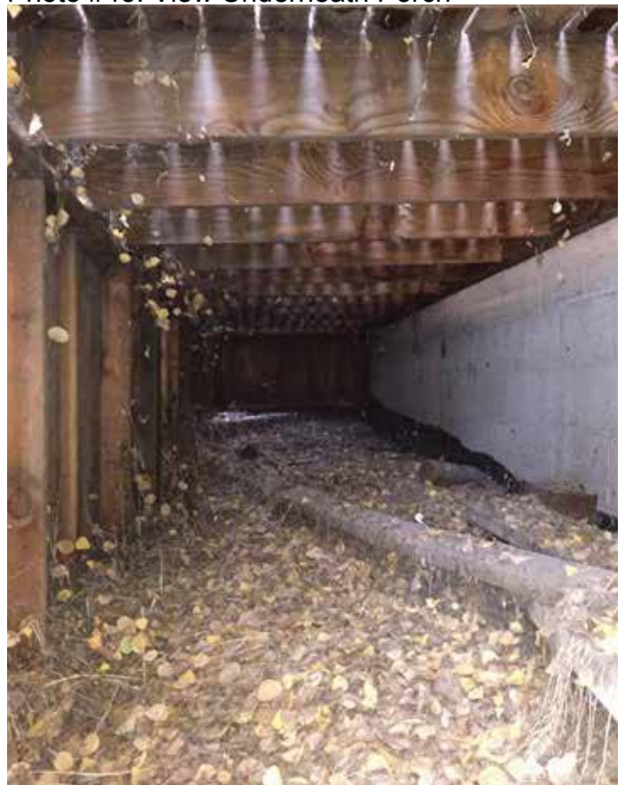
Photo #45: View Underneath Porch
