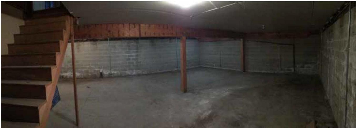
Photo of the interior of the basement. Note the signs of efflorescence on the walls. The heavy timber framing is new and was likely installed when the basement was constructed.
