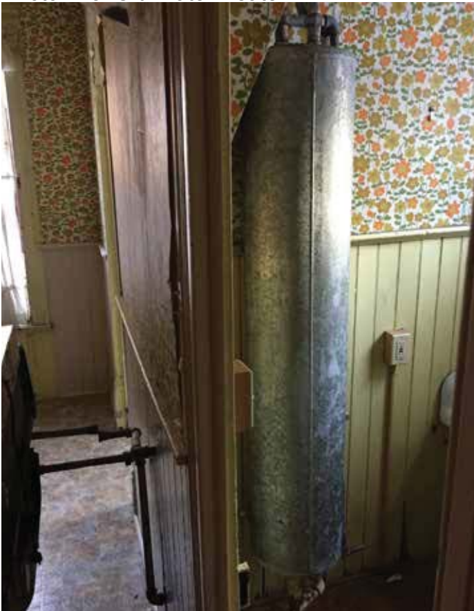
Photo #48: Old Water Heater
