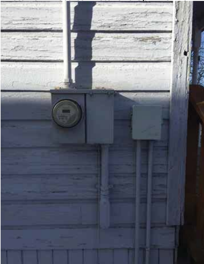
Photo #52: Electrical Meter and Sprinkler Box
