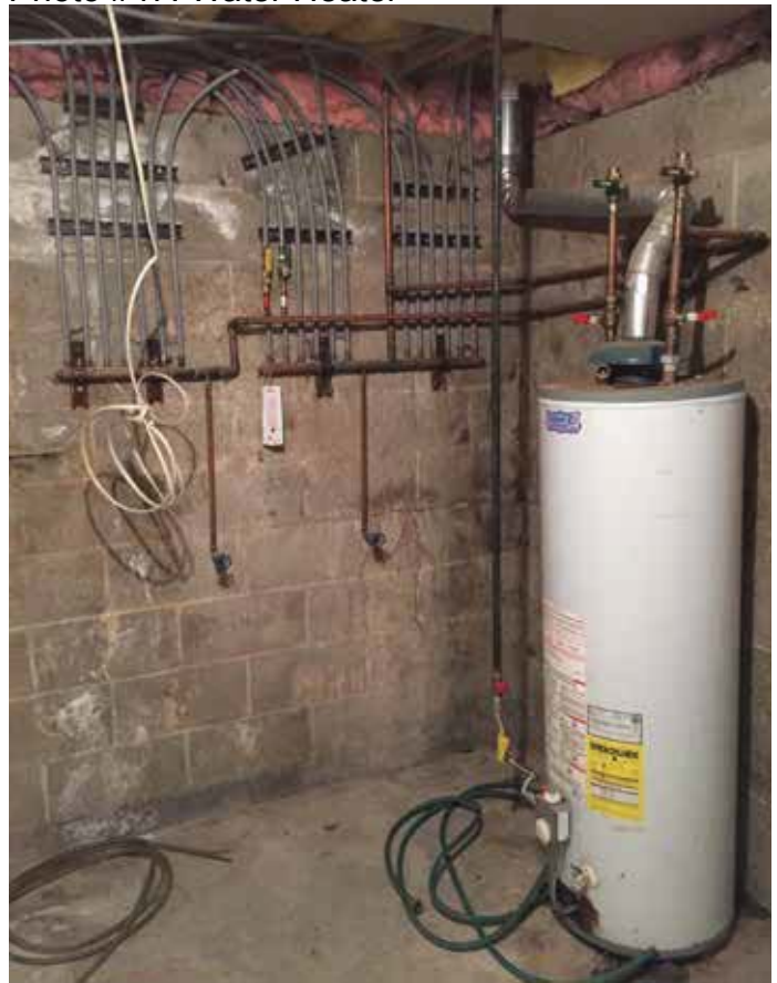
Photo #47: Water Heater
