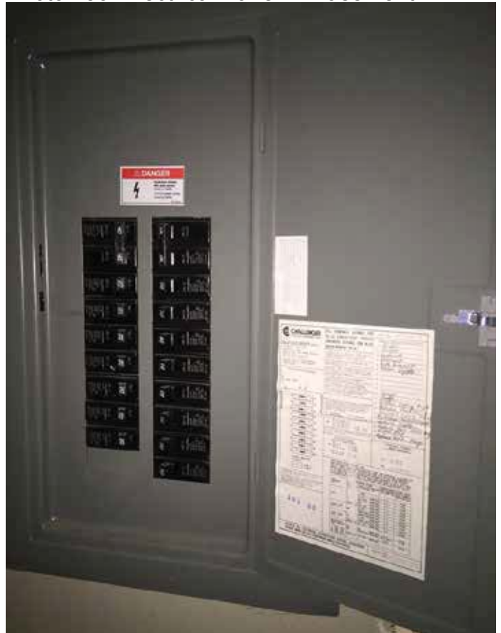
Photo #53: Electrical Panel In Basement
