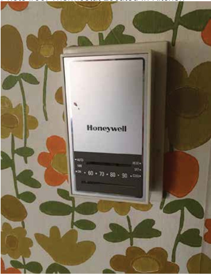
Photo #50: Thermostat Located In Kitchen
