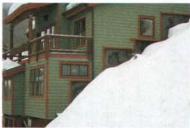
Foundation wall too exposed
