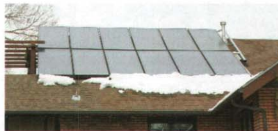
Solar panels visual impacts are minimized
