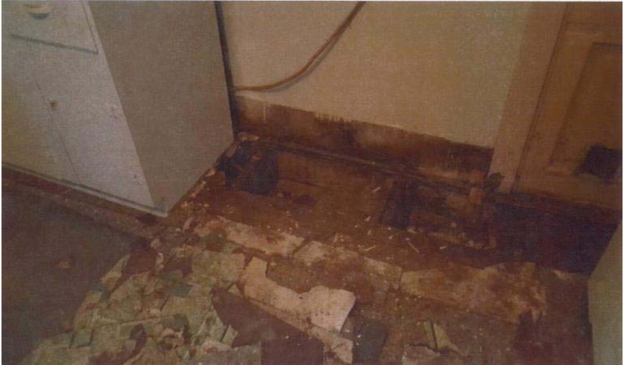
Rotted floor in kitchen against east (rear) wall.
