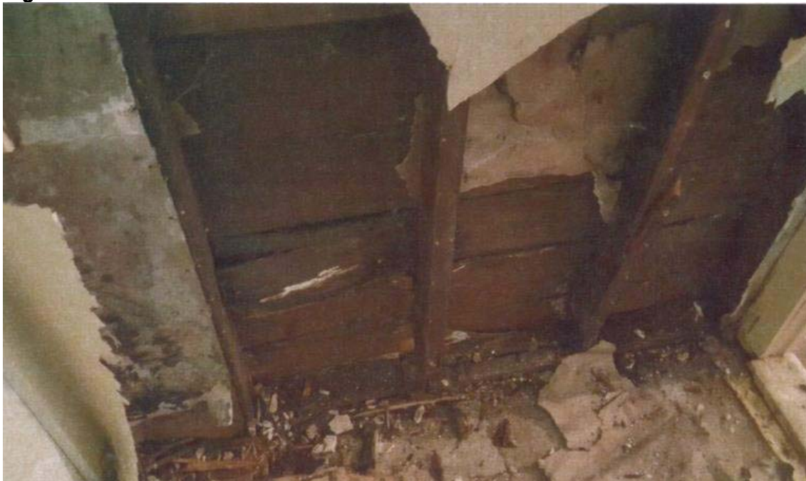
Rotted wall in the bathroom.
