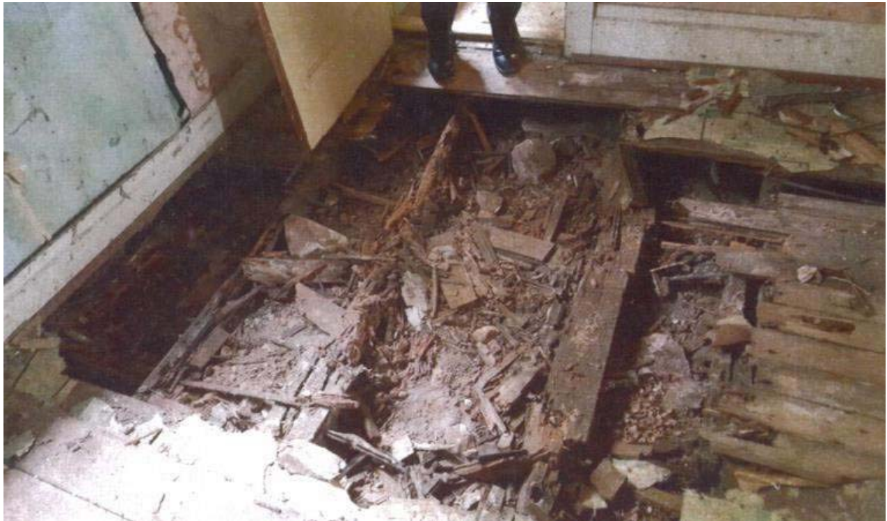
Rotted floor in north bedroom.
