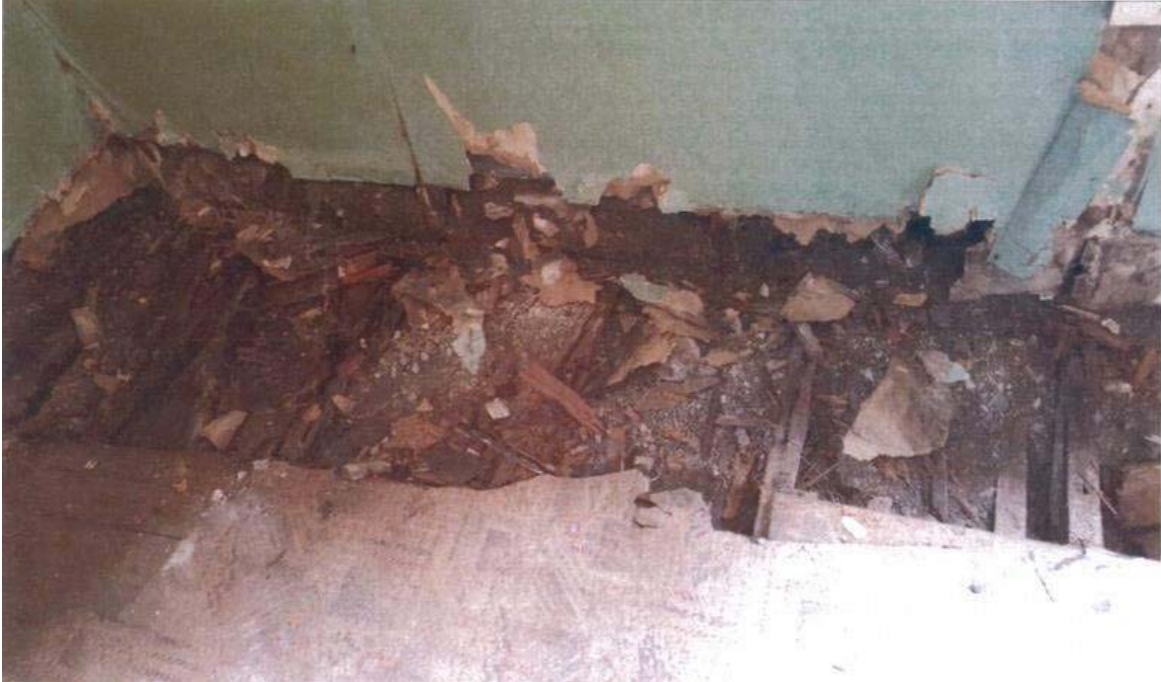
Rotted floor in the south bedroom against the west wall.
