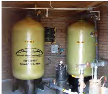
Dual vessels containing MetSorb plumbed in series for added consumer protection
