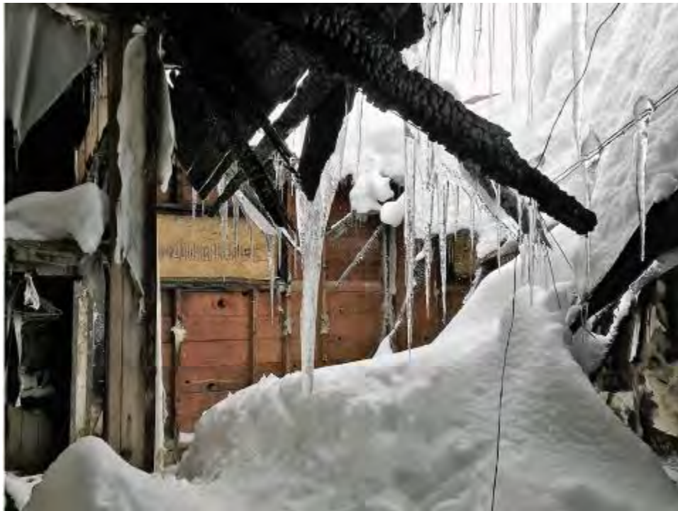
Photo of interior of c.1969 addition and historic wall of the house. Due to the hole in the roof of the c.1969 addition, the back portion of the historic house and the c.1969 addition have been largely exposed to the elements.
