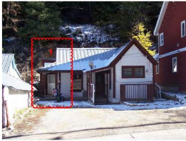
This photograph shows the location of Addition 1. On the west (façade) elevation, it is clad in wood siding and appears largely identical to the addition shown in the c.1941 tax photograph.
