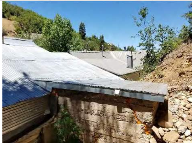
This photograph taken from the southeast corner of the site shows the rough-poured concrete root cellar/mechanical room (Addition #2). Also note the corrugated metal siding on the east (rear) wall of Addition #1.
