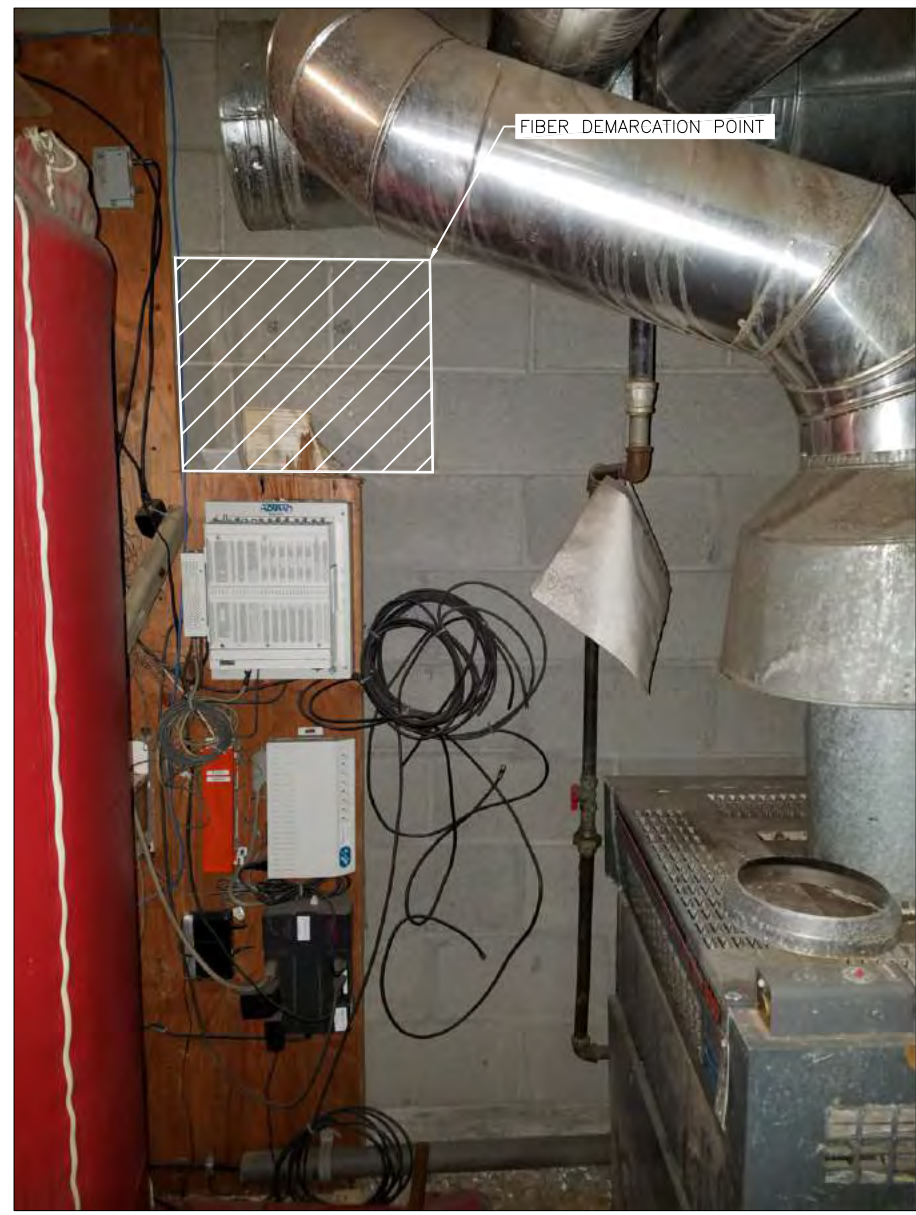
VIEW OF FIBER DEMARCATION POINT
