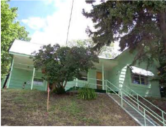
C.2009 reconnaissance survey photo of the house. Note the metal porch rails that match those on the concrete stairs.
