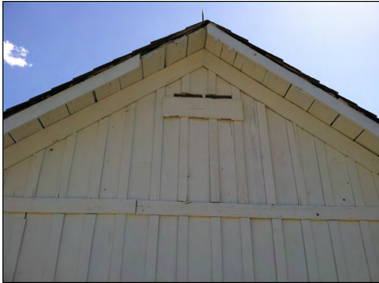
Figure 99. A missing section of fly rafter on the gable end of the tool shed.
