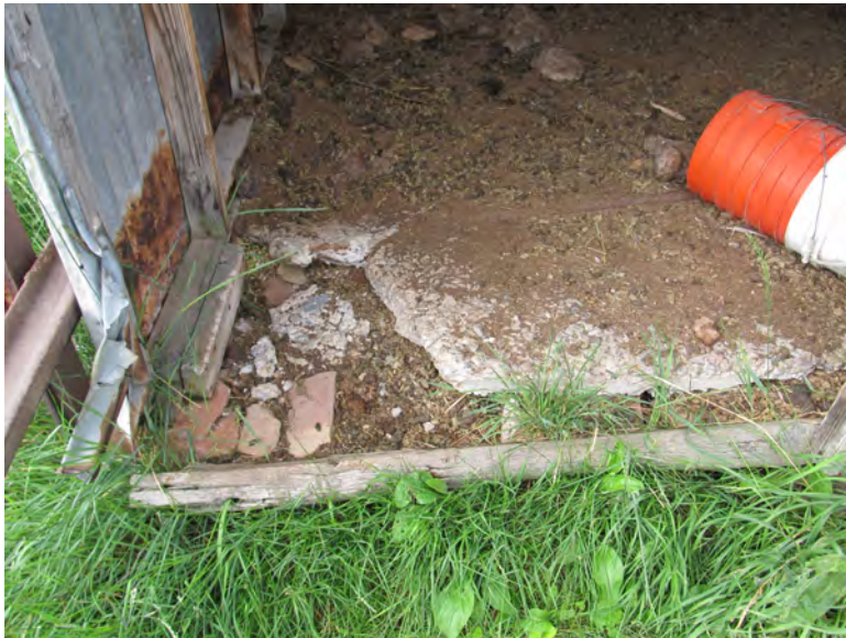
Figure 95. Damaged concrete floor and deteriorated wood sill on northeast side of animal shelter.
