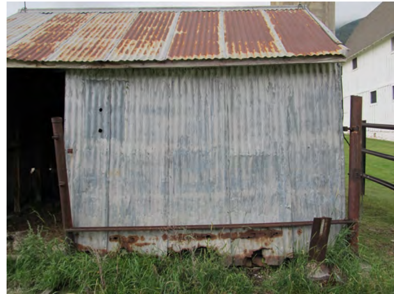
Figure 96. Corroded and detached metal panels on the walls and roof of the animal shelter, facing southwest.
