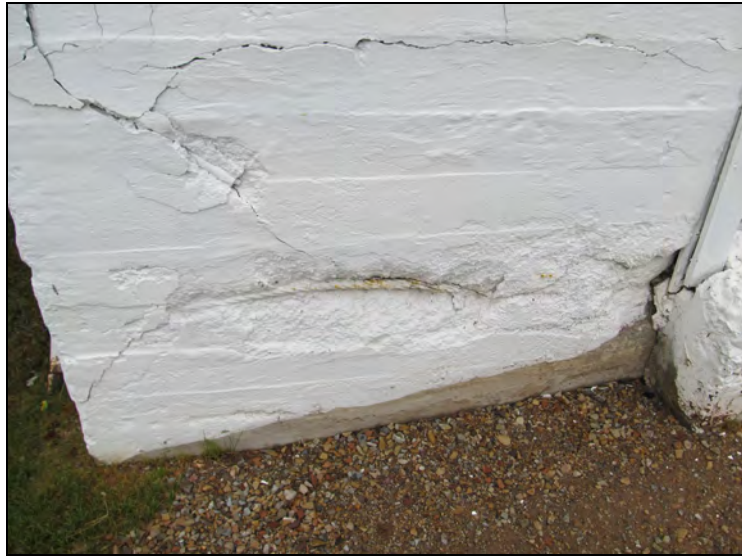
Figure 88. Cracking and spalling concrete on the milk house addition, facing southeast.
