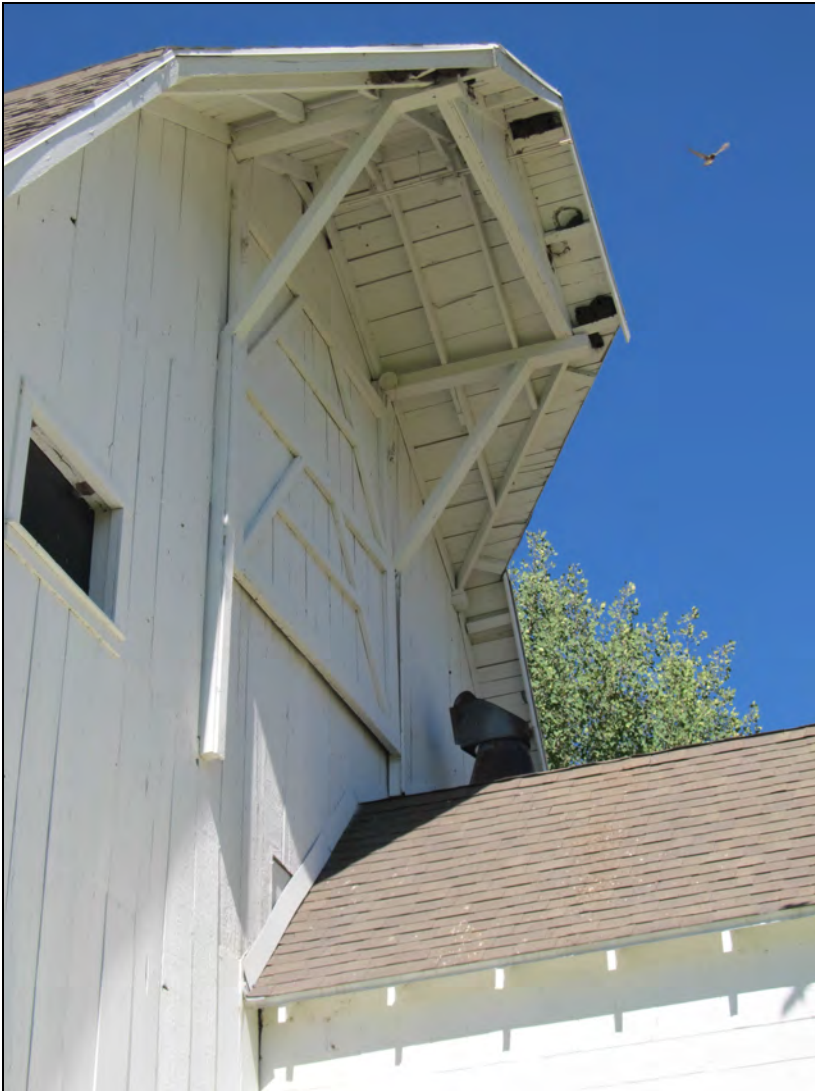
Figure 35. Northeast end of barn showing gable end and sliding doors to hay mow on upper level.
