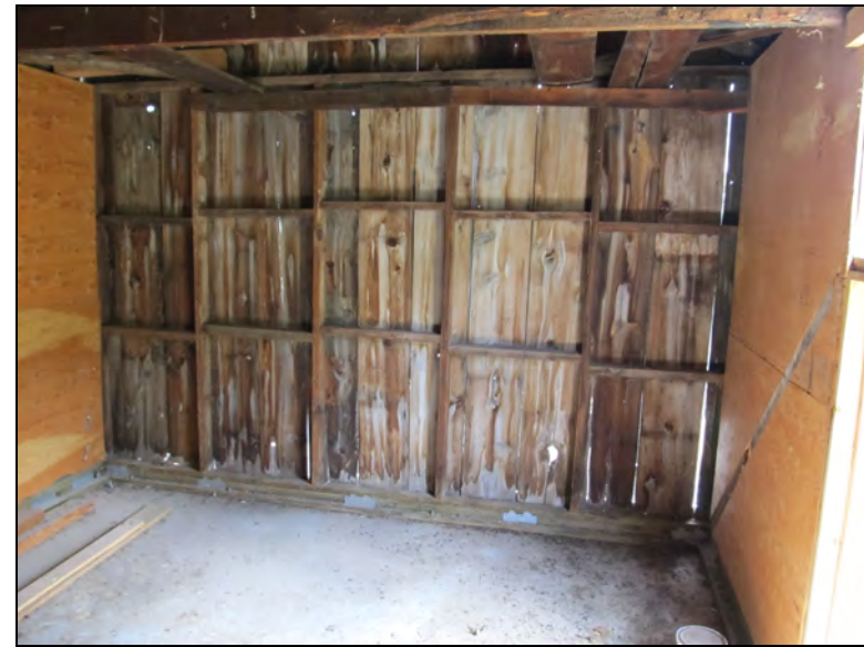
Figure 98. Modern interior plywood sheathing abutting a historic end wall of the granary.
