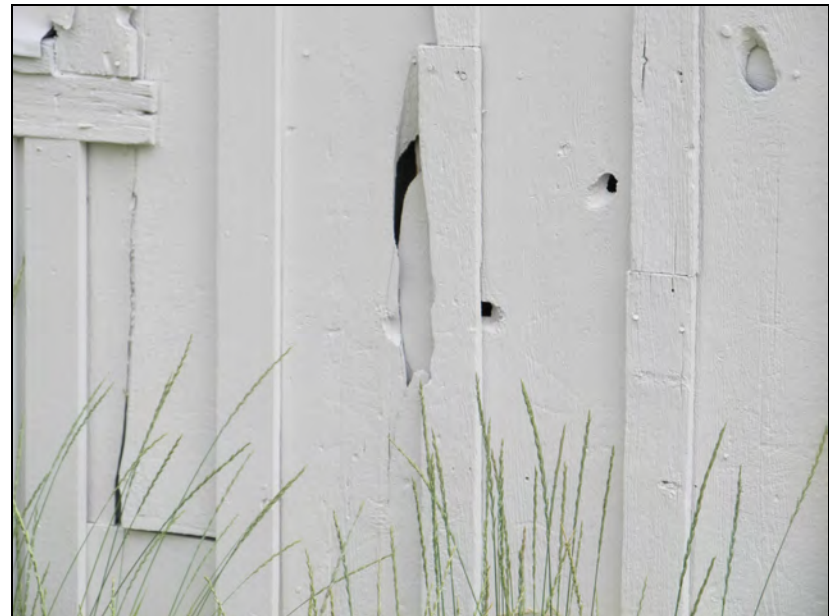
Figure 97. Evidence of past damage and repairs to the exterior board-and-batten walls of the granary.
