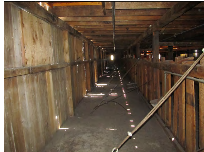
Figure 92. Cable bracing along a side aisle on the main level of the barn.
