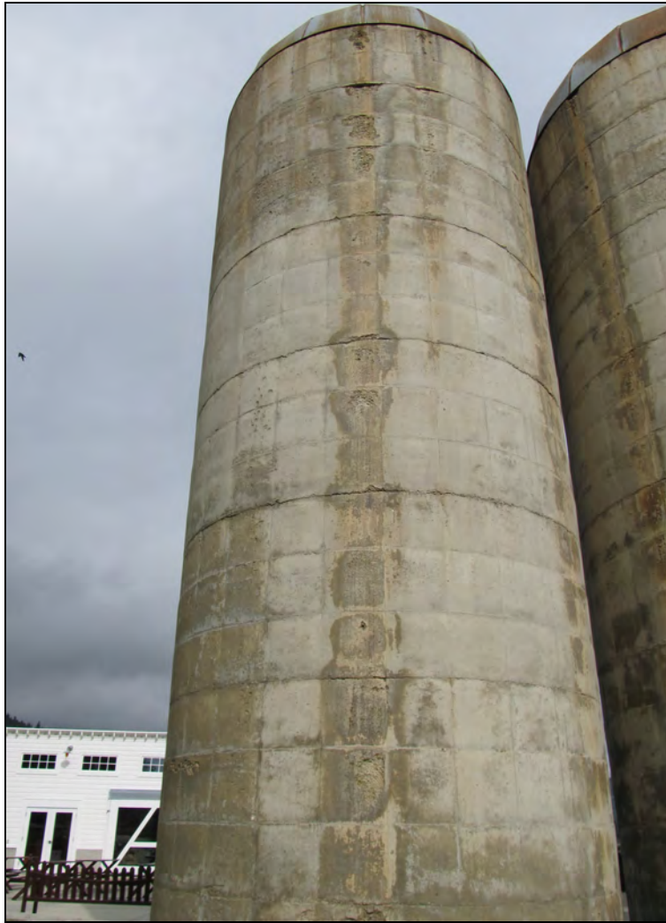
Figure 102. Rain runoff patterns on grain silos have caused some concrete discoloration, spalling, and metal corrosion; facing north.
