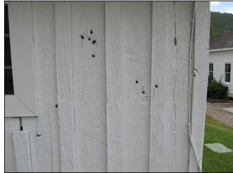
Figure 101. Past damage to the board-and-batten siding of the bunkhouse, facing northeast.
