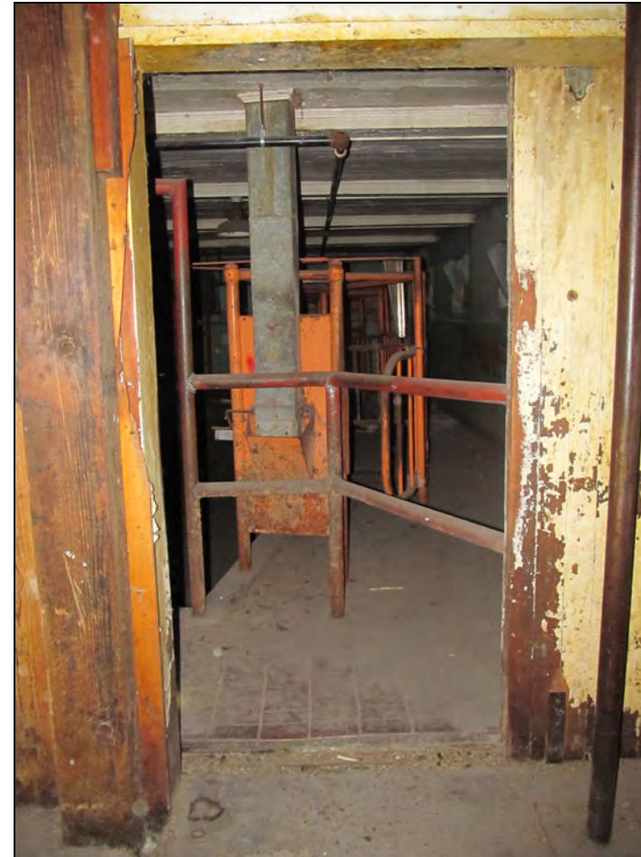
Figure 48. Door in northeast end of barn providing access to milking parlor, facing northeast.
