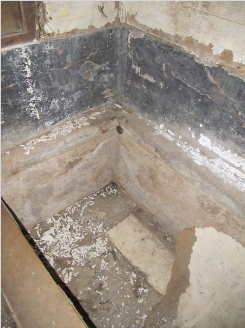
Figure 93. Paint deterioration on concrete walls of milk house interior.
