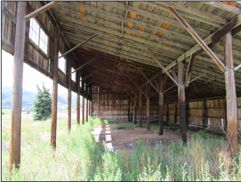
Figure 105. Interior view of Osguthorpe shed showing missing windows, water staining, moisture damage at wall bases, and roof repairs.
