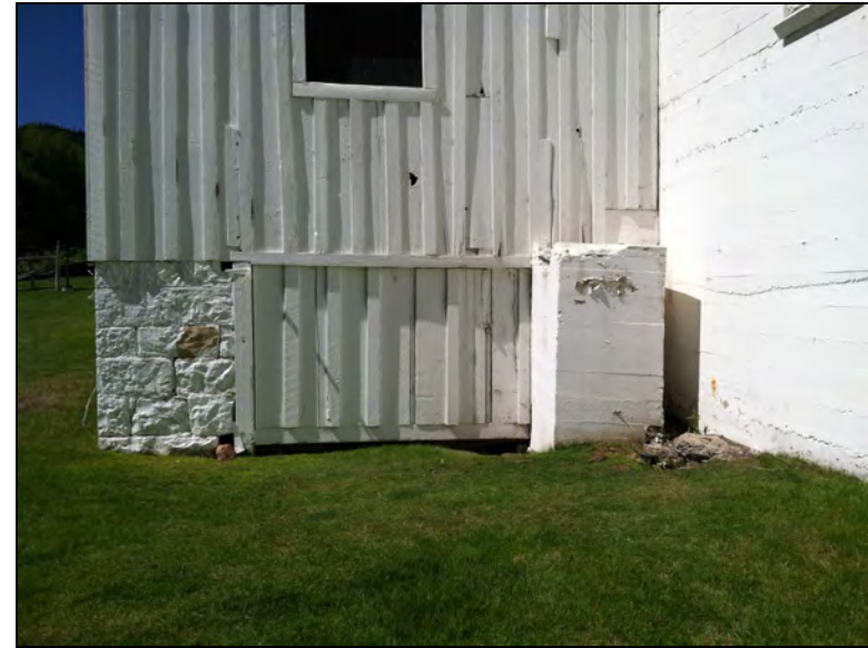
Figure 37. Board-and-batten door on northeast side of the barn leading to lower-level crawl space.
