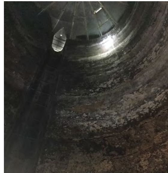
Figure 104. Grain silo interior, looking upward, showing concrete abrasion and discoloration.
