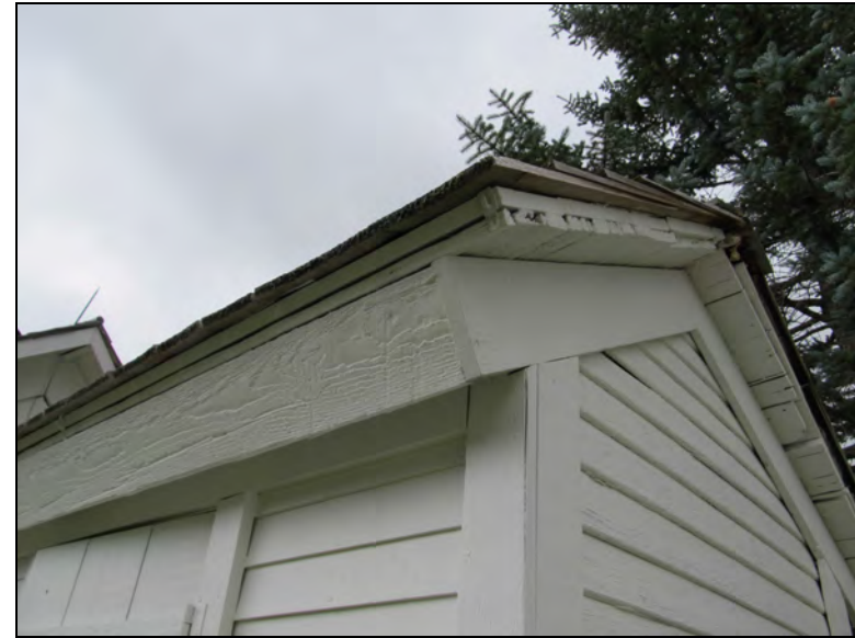
Figure 100. A new fascia board installed when the outhouse was reconstructed, facing south. Past deterioration of the roof sheathing is visible.
