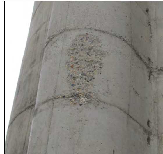
Figure 103. Concrete spalling and exposed aggregate on a grain silo wall.
