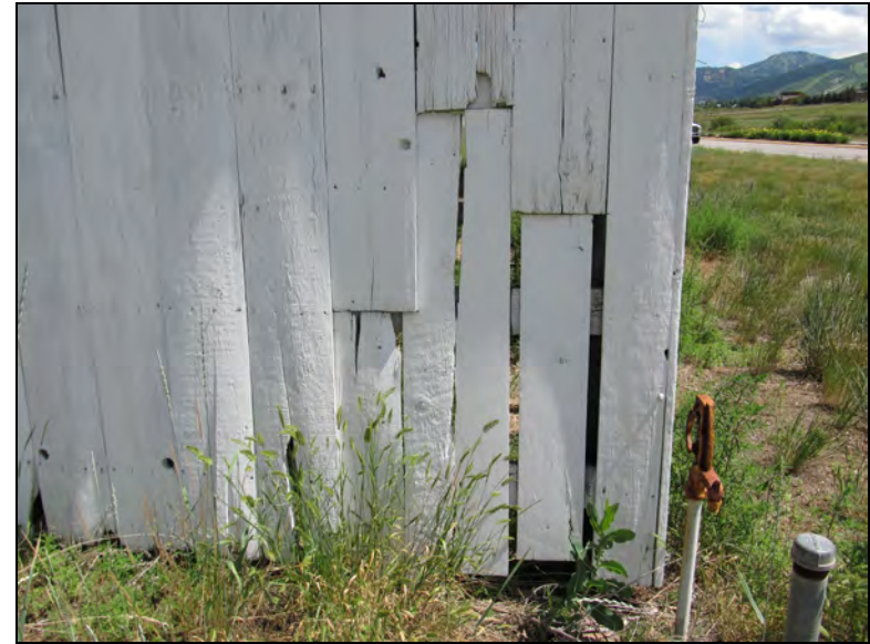
Figure 106. Cracking, rot, and detachment of wood siding on the northwest side of the Osguthorpe shed, facing northeast.
