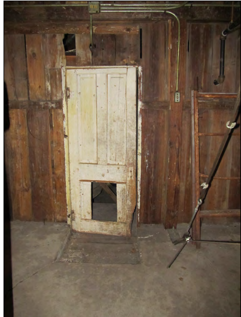
Figure 94. Damaged four-panel door leading from barn to milk house vestibule, facing northwest.
