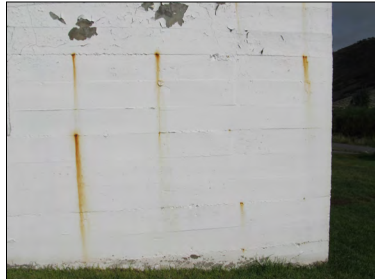
Figure 91. Corrosion and peeling paint on wall of milking parlor due to irrigation system overspray, facing northwest.
