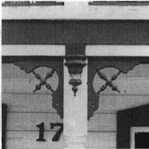
These original wood porch brackets have been kept in repair. A good coat of paint has prevented decay.
