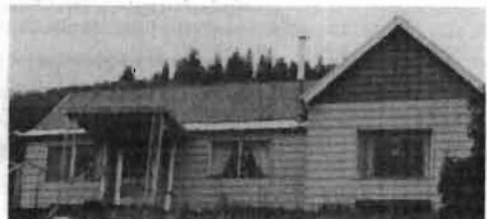
The lap dimension of this synthetic siding has altered the character of this house. The wrought iron porch supports are also not appropriate, and the new windows with horizontal emphasis are not typical of historic houses.
