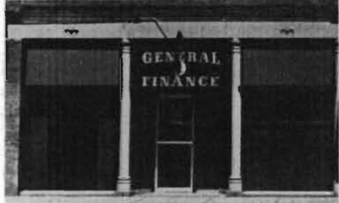
One appropriate position for a sign is in the clerestory panel. In this case, it is positioned to emphasize the entrance of this business. Notice the contemporary storefront elements. The door, however, is not appropriate because of its unfinished metal frame.
