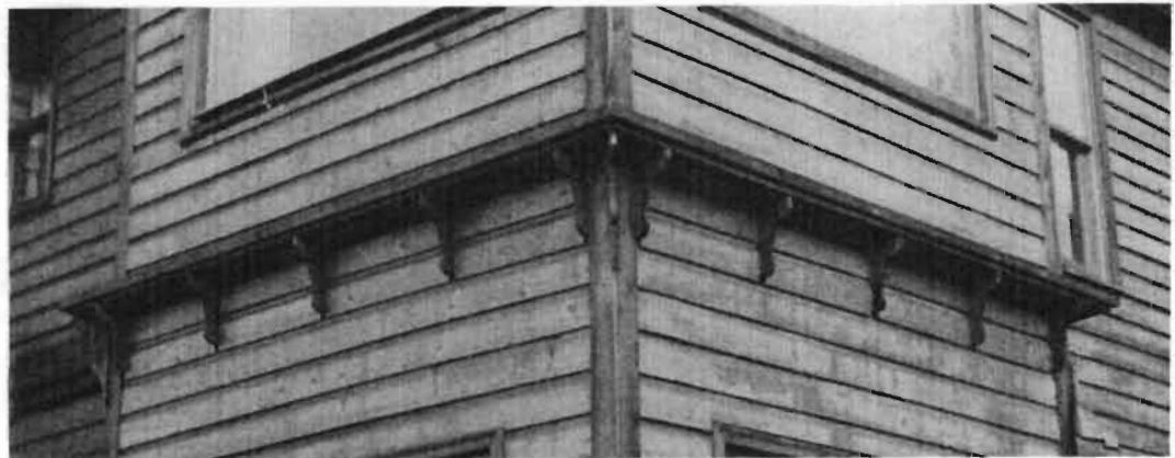
Simplified details, such as these brackets, may be substituted for the originals when necessary.
