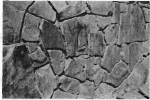
The stone in this new wall is obviously a veneer. The random pattern distracts from the more formal patterns of the street.
