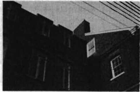
The new windows on the left are similar in size and shape to the older neighbor. (The small panes on the right would not be appropriate in Park City).
