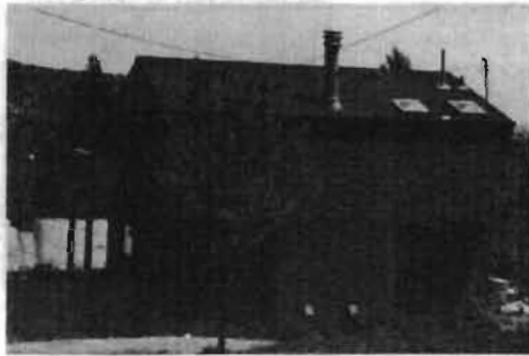
New siding that matches the lap dimension of existing houses is preferred.
