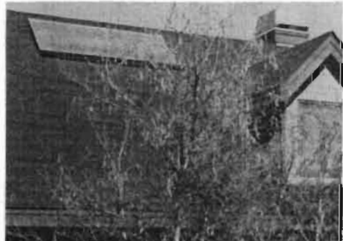
This collector is away from the street view and lies close to the roof.
