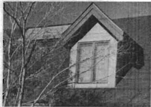
This collector is away from the street view and lies close to the roof.
