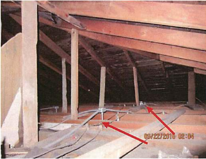
Photo 17 Knob and tube wiring located throughout the attic area
