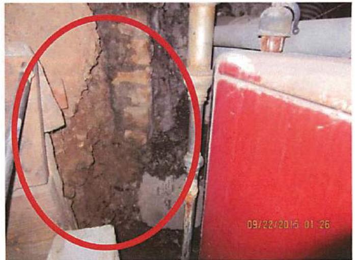
Photo 2 Decay of the rubble foundation due to water infiltration
