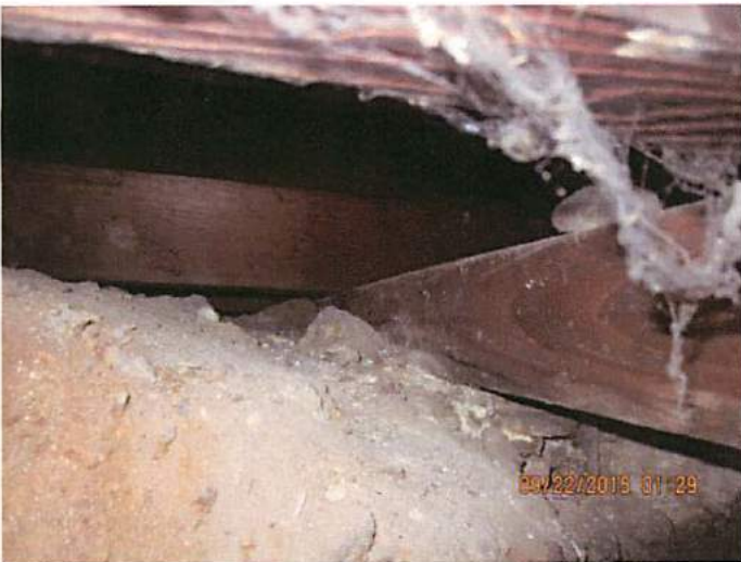
Photo 7 The floor joist of the structure are resting directly on top of dirt and rubble. Not permitted under building codes
