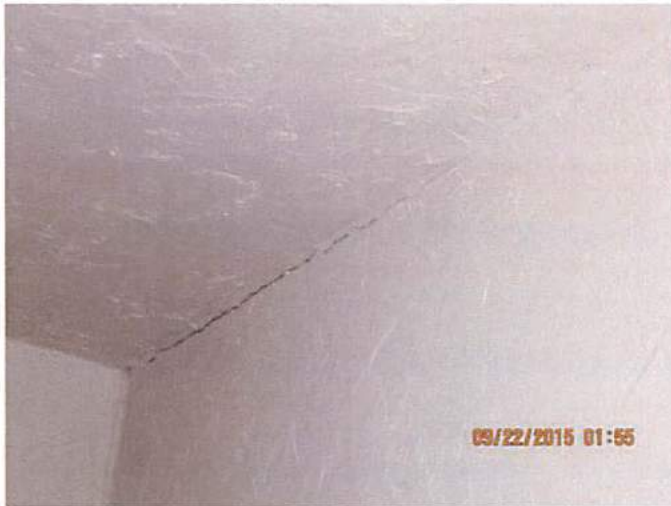
Photo 13 Structural separation in second floor bedroom. Consistent with missing point loads and missing foundation
