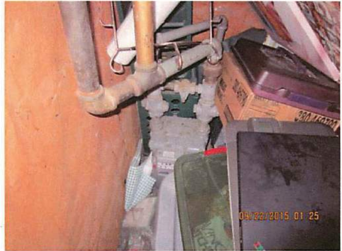
Photo 2 Gas meter is located in a hidden room with possible improper connections to the building. The room is located in the front of the deli between the entry doors
