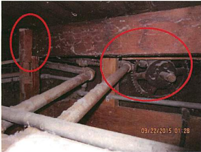
Photo 23 The addition of bracing and shims to prevent settling of the building. Cannot have bearing directly on soils. All bearing is directly on soils. Engineer to justify
