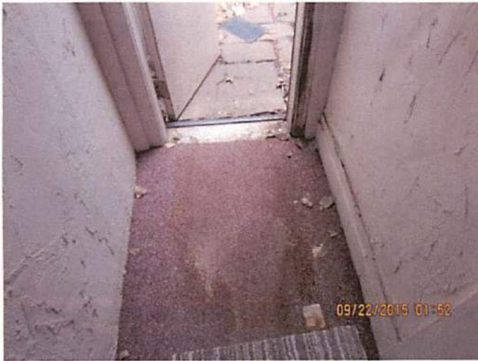
Photo 35 Egress from the back of the dwelling serving 50% of 8 units or 22 occupants cannot be used. Gates are locked to prevent escape and no safe access to the front of the building is provided. Limited egress, direct violation of the fire code for egress requirements for type R-3 buildings and occupant load
