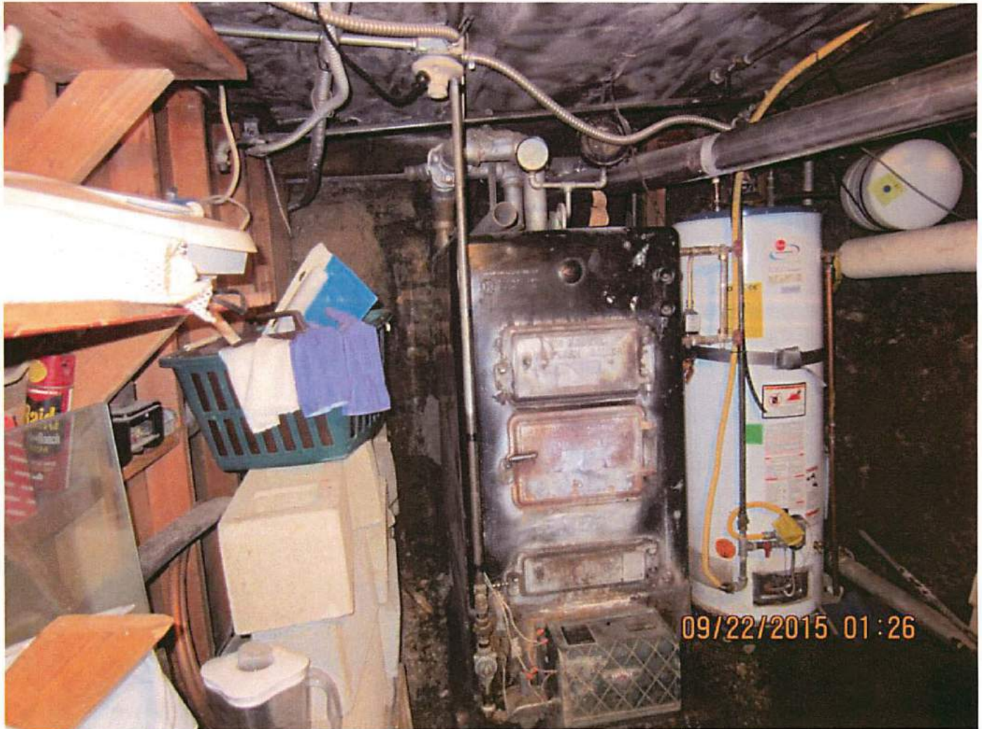
Photo 11 The building is being heated by a 1930's era boiler that has been converted from coal/wood to natural gas. The boiler has no current state boiler inspection tags and required by state law to be inspected annually. It is advised the state boiler be notified for a immediate safety check on the boiler. The gas line that feeds the boiler is unsafe and should be terminated .
