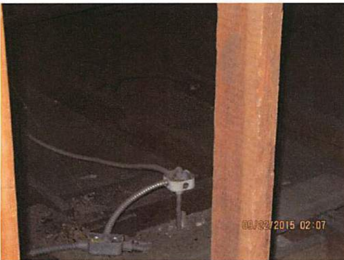
Photo 20 Open electrical boxes noted throughout the building. Electrocutation hazard, fire hazard. Located in attic
