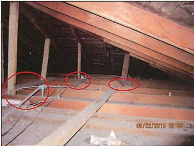
Photo 1 The structural members supporting the roof are not properly installed and are not plumb. Excessive load could cause the members to fail
