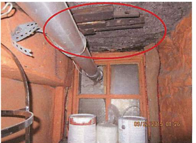
Photo 28 Rail road rails being used as shims for floor above. This area would be Approximately 18 feet into front entry main level.
