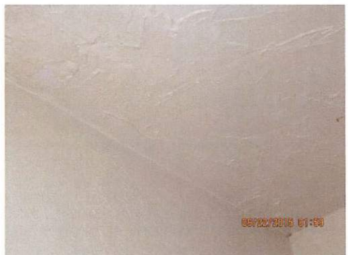
Photo 16 Use of heavy texture was noted on recent repairs. Possibly being used to hide structural separation. Noted cracking and voids behind texture
