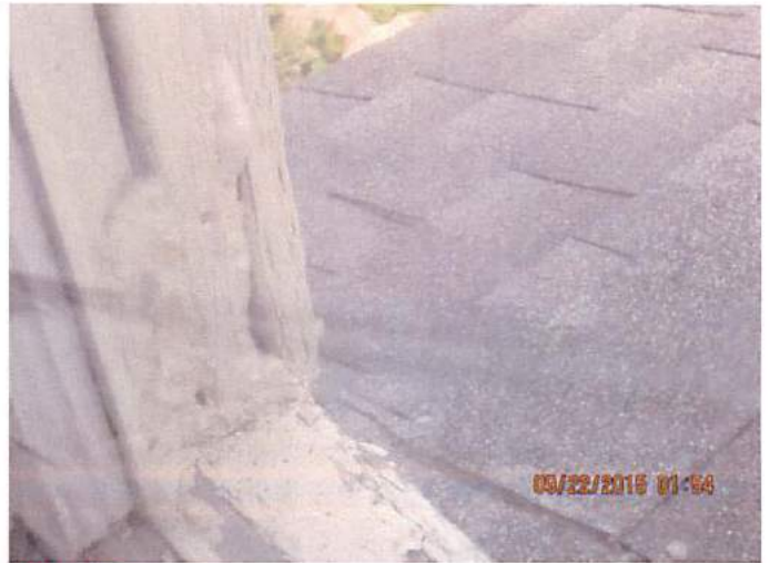
Photo 23 Decay and deterioration noted throughout the building, cause appears to be lack of proper maintenance and infiltration of water from damaged roof
