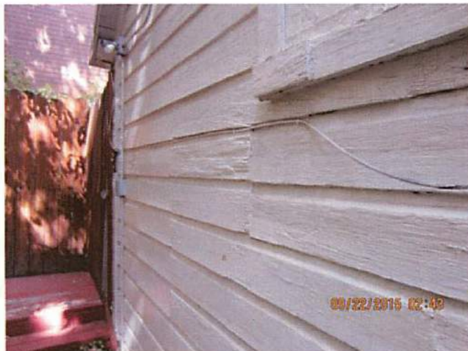
Photo 37 Egress path rear of building. No access to safe location
