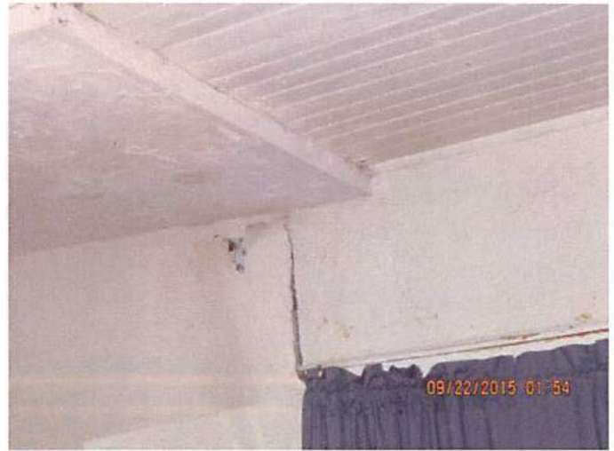
Photo 12 Structural separation in second floor bedroom. Consistent with missing point loads and missing foundation
