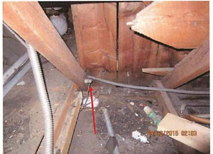
Photo 16 Knob and tube wiring located throughout the attic area
