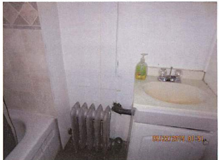
Photo 13 Example of the radiator heating system that uses the boiler to heat the building
