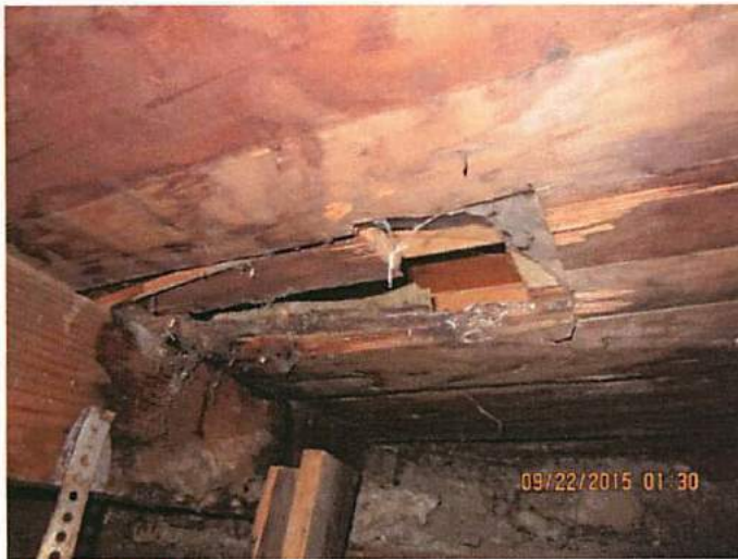
Photo 19 Several shims and braces have been used to level the building. These shims and braces have not been properly installed
