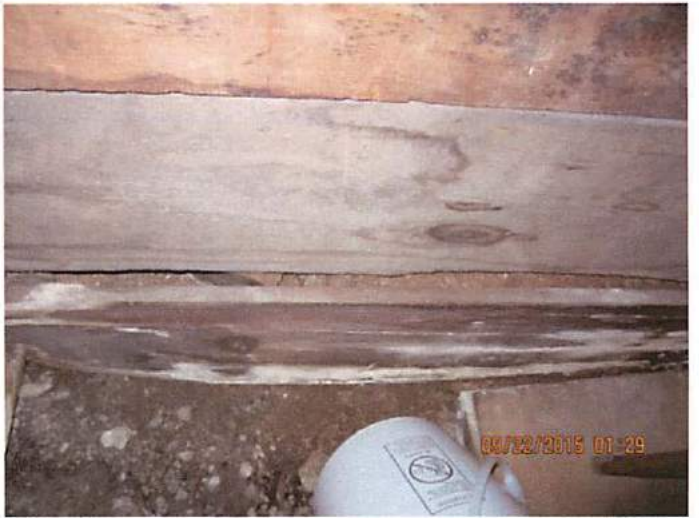
Photo 8 Wood backing being used to prevent rubble from filling the storage area. Backing is failing and decayed. Serious mold and water concerns
