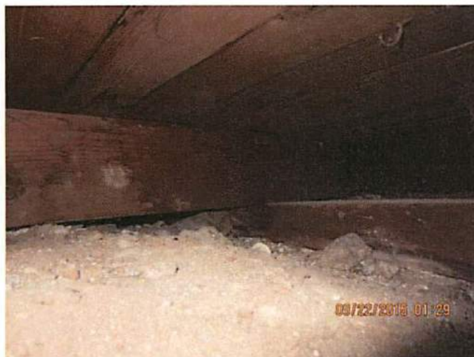
Photo 21 Floor joist are bearing directly on top of soils. This is not permitted by code
