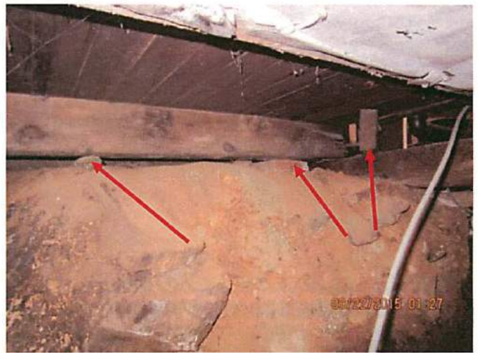
Photo 24 The addition of bracing and shims to prevent settling of the building. Cannot have bearing directly on soils. All bearing is directly on soils. Engineer to justify
