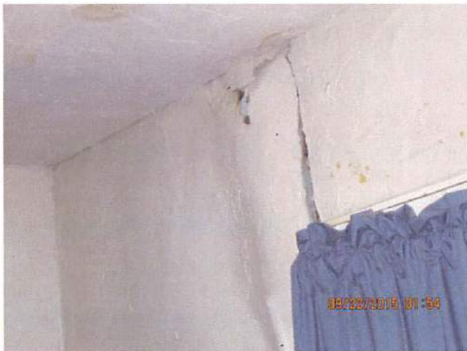
Photo 24 Decay and deterioration noted throughout the building, cause appears to be lack of proper maintenance and infiltration of water from damaged roof
