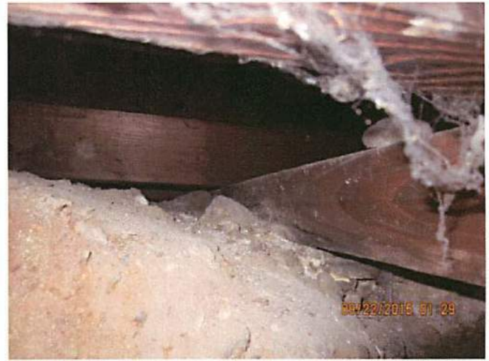
Photo 20 Floor joist are bearing directly on top of soils. This is not permitted by code
