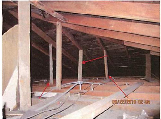
Photo 2 Support members for roof are not adequate for the purpose being served. Engineer to justify
