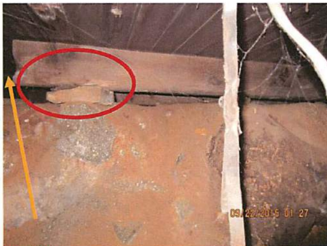
Photo 25 The red circle shows a direct load at the end of a cut off floor joist. The blocking is bearing directly on soils. The yellow arrow shows the removal of a floor joist. The area above is the dining room
