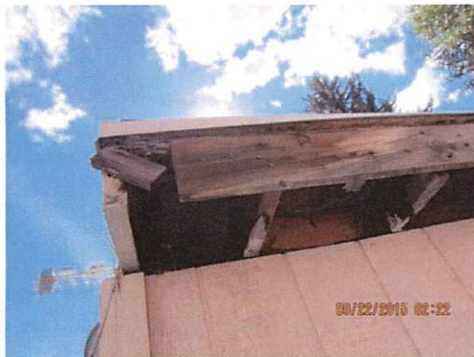
Photo 32 Roof shows sign of decay and rot damage, soffit and fascia are missing, possible location of water infiltration
