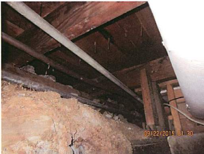
Photo 3 There are numerous pipes consisting of potable water, heating water lines and gas lines that are in direct contact with soils and not properly secured. Decay and deterioration of piping is noted throughout the underground area
