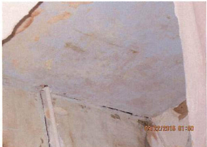
Photo 10 Water damage second floor. Settling cracks noted. Structural engineer to justify
