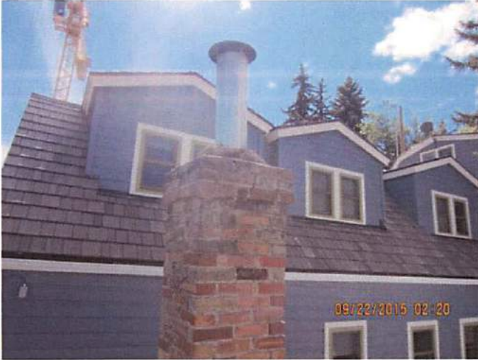
Photo 1 The chimney shows signs of decay and instability. To be removed or evaluated by a structural engineer
