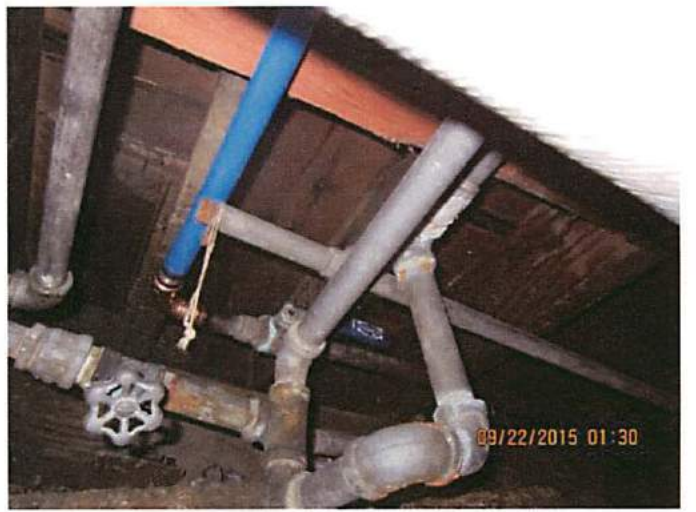
Photo 8 Improperly installed plumbing repairs. Ends not properly capped. Copper to galvanized requires a brass coupler
