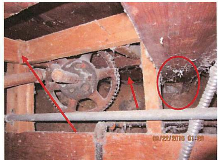
Photo 22 Floor joist bearing directly on dirt. Shims and bracing added for support. Improperly installed
