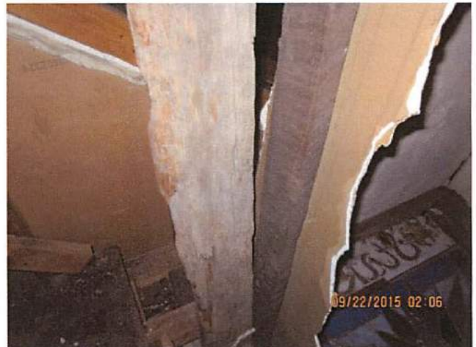
Photo 4 Structural members not properly supported
