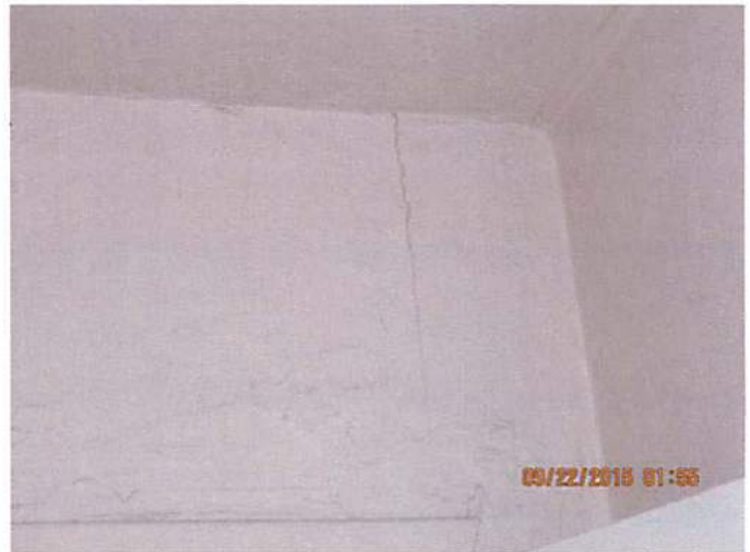
Photo 14 Structural separation in second floor bedroom. Consistent with missing point loads and missing foundation
