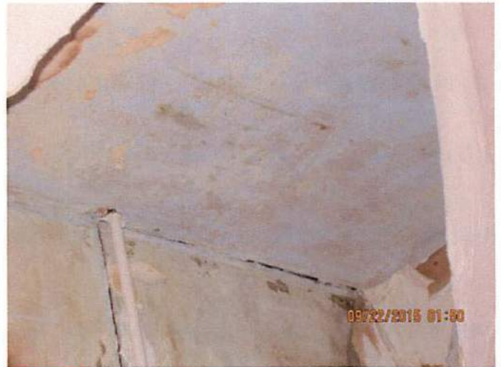
Photo 25 Decay and deterioration noted throughout the building, cause appears to be lack of proper maintenance and infiltration of water from damaged roof
