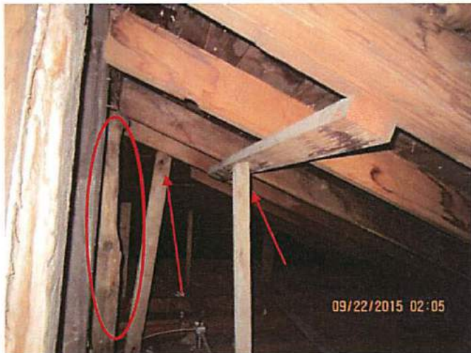
Photo 3 Damaged, decayed or improperly installed structural members
