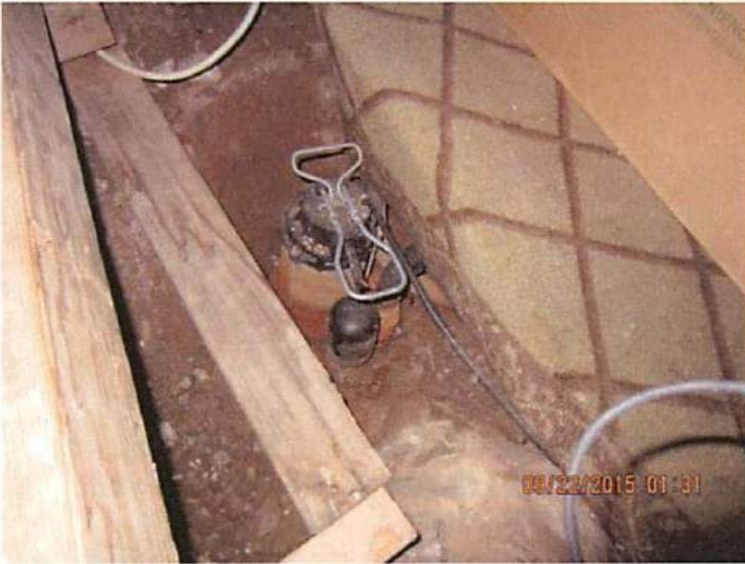
Photo 5 A sump was installed to remove water from the area but was not properly maintained and currently is not in working condition
