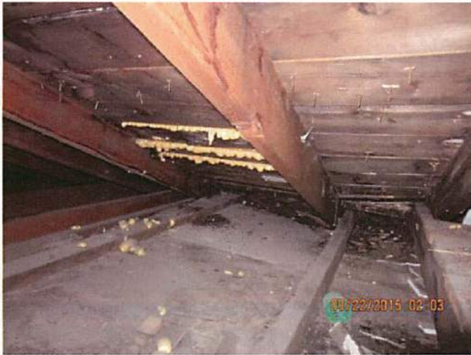
Photo 28 Roof leaks being repaired with a product that is not designed for such use
