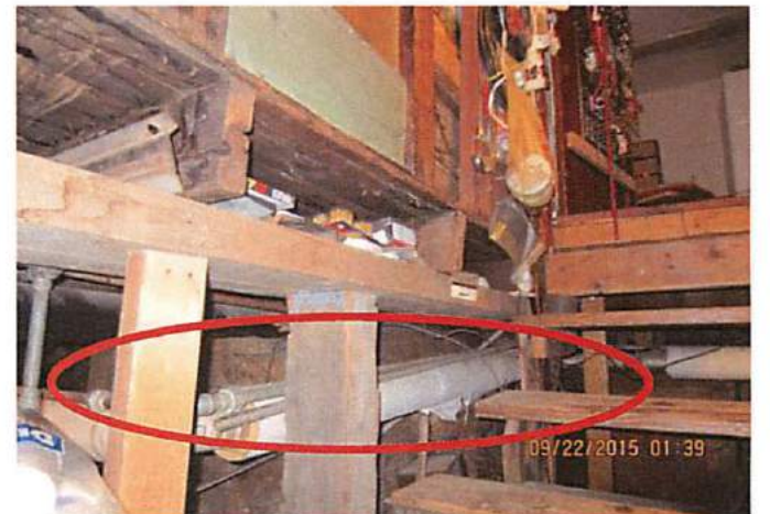
Photo 10 Example of missing foundation under support member. Connection to support from attic 3rd floor
