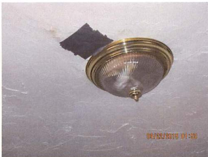
Photo 26 Tape being used to cove water damage next to electrical outlet that feeds light
