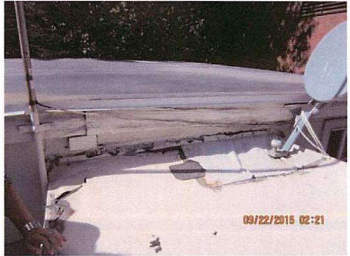
Photo 29 Roof appears to have been recently repaired but some areas are damaged and show signs of possible water infiltration
