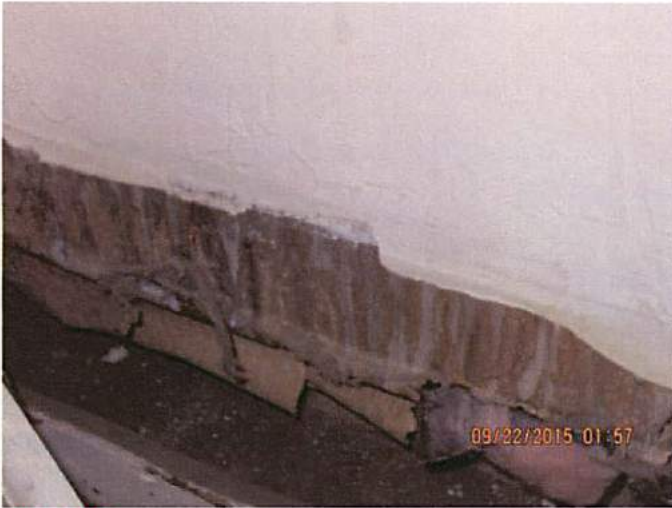
Photo 22 Decay and deterioration noted throughout the building, cause appears to be lack of proper maintenance and infiltration of water from damaged roof
