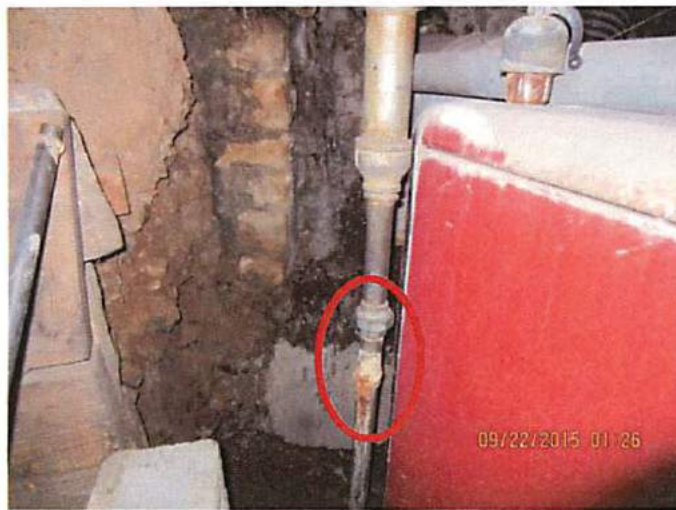
Photo 9 Gas line shows decay and deterioration needs to be shut off ASAP
