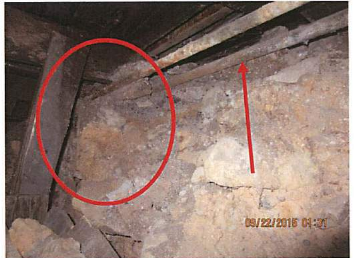
Photo 4 The red circle shows movement of the rubble foundation and decay of the floor joist members resting directly on top of the rubble. The red arrow shows decay of water lines used to heat the structure
