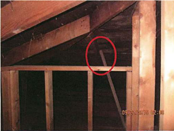
Photo 5 Support member not properly fastened
