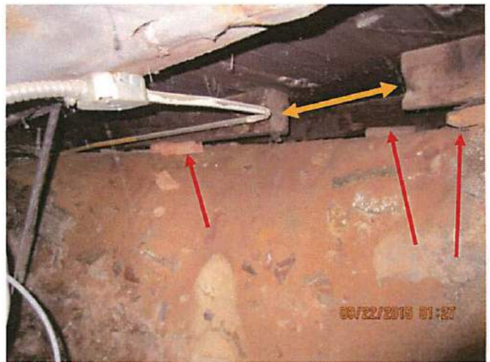
Photo 26 The addition of bracing and shims to prevent settling of the building. Cannot have bearing directly on soils. All bearing is directly on soils. Engineer to justify
