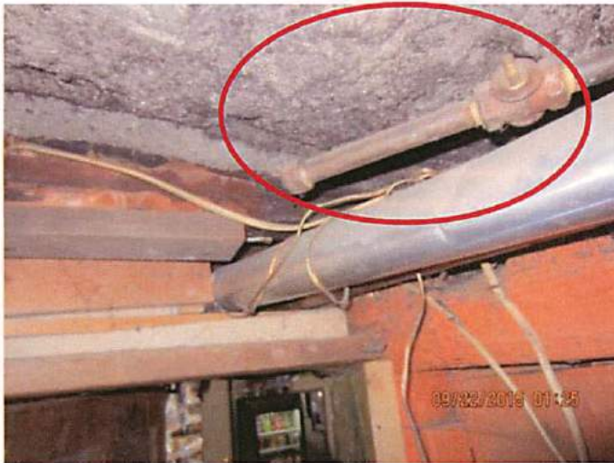
Photo 1 Gas lines that have terminated in hidden rooms that are not properly secured. This room is located in the deli in the front area between entry doors
