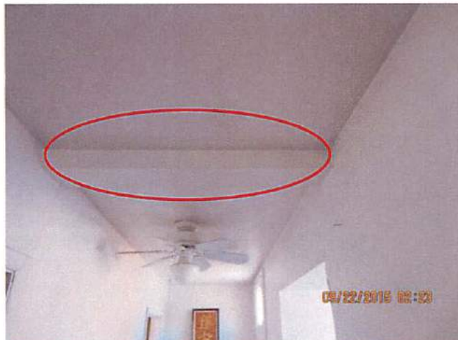
Photo 9 The third level of the structure was added in the 1970's. The addition will need to be evaluated by a structural engineer. The support beam in this photo is missing a point load.
