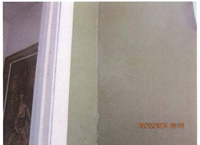
Photo 27 Water damage and structural concern behind wall
