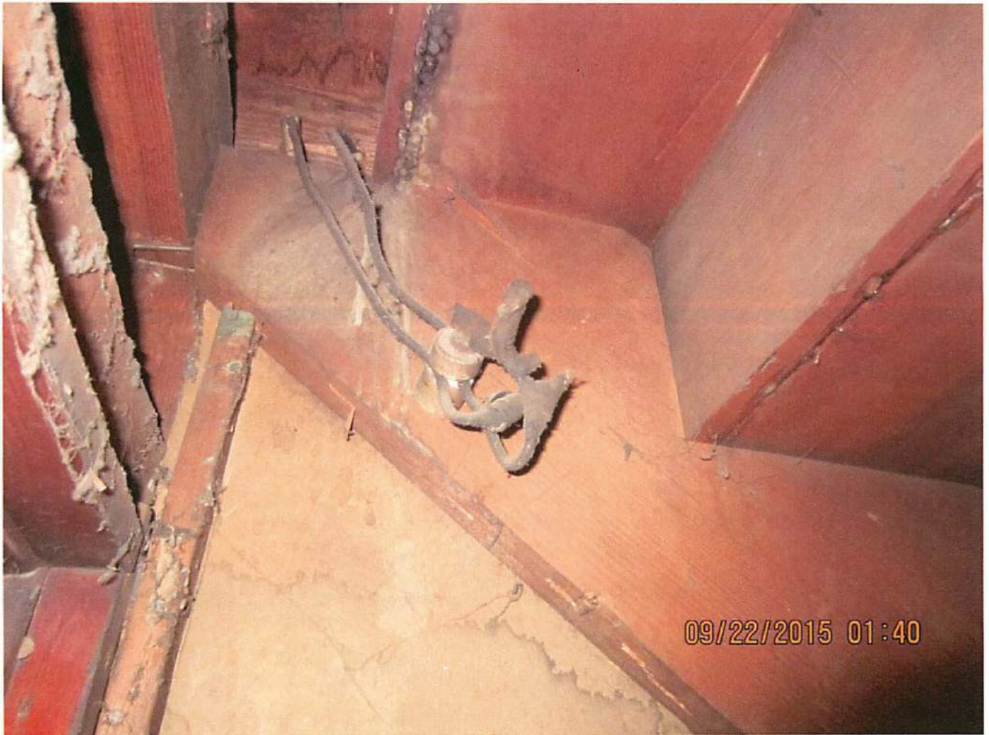
Photo 14 Knob and tube electrical is located throughout the building. Knob and tube type wiring is classified as a possible health, life and safety concern if not properly maintained. It is common practice and a requirement of the electrical code to remove knob and tube wiring if any portion of the building is upgraded with newer electrical wiring. The building shows numerous upgrades in wiring and electrical upgrades, such as electrical panels, breakers, outlets and lighting. The knob and tube may not be able to support the current electrical upgrades in a safe manner and may be a fire concern. An electrical engineer needs to evaluate the electrical for the entire building before the electricity is turned on.
