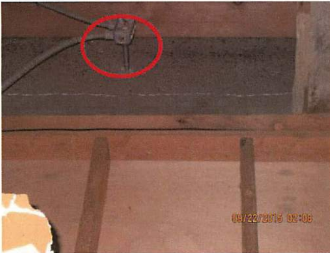
Photo 18 Open electrical boxes noted throughout the building. Electrocutation hazard, fire hazard. Located in attic
