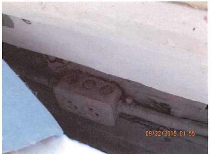
Photo 21 Outlets located under windows that are damaged. Moisture and decay surrounds the electrical outlet
