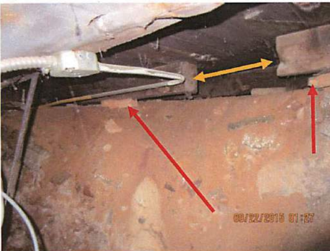
Photo 3 The red arrows show improperly installed shims are blocking to level the floor above. Not permitted on dirt . The yellow arrow shows the removal of floor joist, this is consistent throughout the floor area
