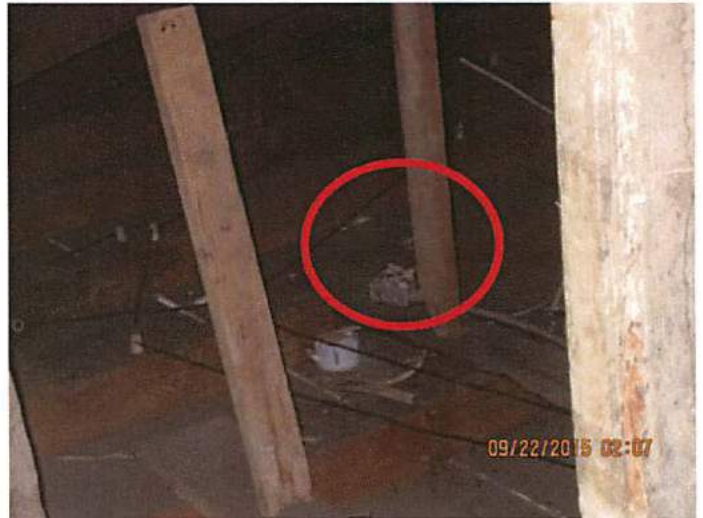
Photo 19 Open electrical boxes noted throughout the building. Electrocutation hazard, fire hazard. Located in attic
