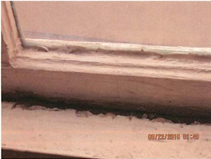
Photo 17 Several windows on the second floor have separated and have been nailed shut. This is consistent with cracked and warped walls due to structural stability of the building
