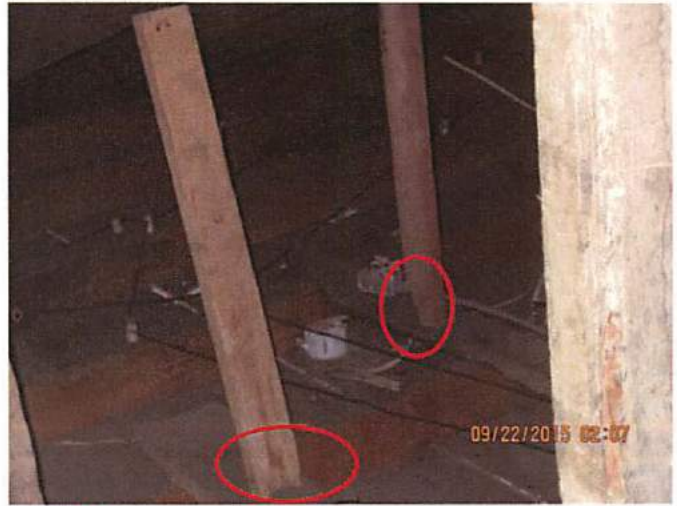
Photo 6 Support members not fastened and are not perpendicular to the load they serve
