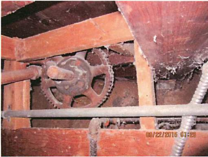
Photo 5 Unknown valves that are not properly maintained, marked or accessible
