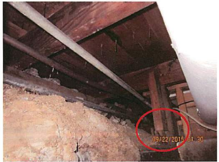
Photo 18 Several shims have been used to level the building. These shims have not been properly installed
