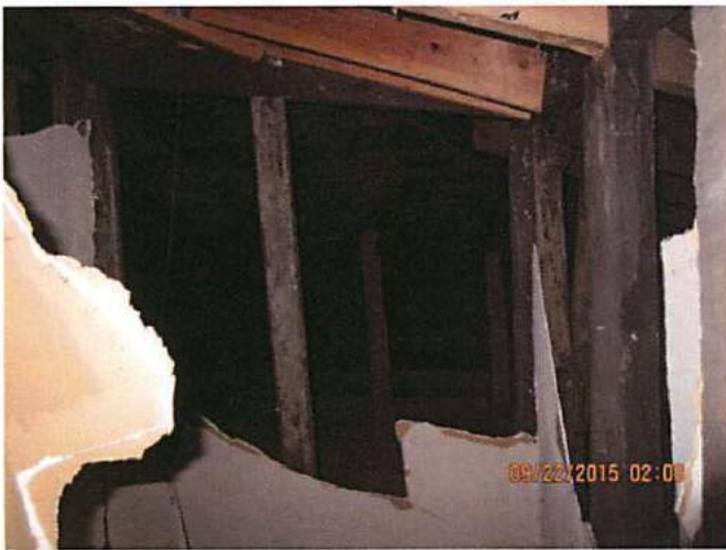
Photo 7 Roof has been repaired, support members not properly installed. Engineer to evaluate and justify
