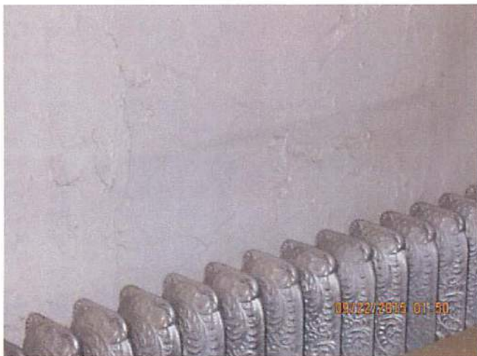
Photo 12 Example of the radiator heating system that uses the boiler to heat the building
