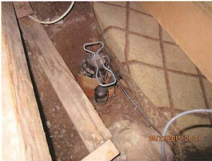
Photo 7 A water/trash pump is located directly below photo 6, the pump is not in working condition
