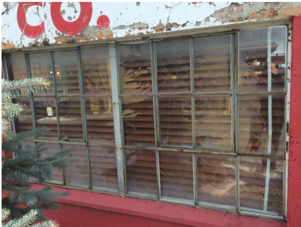
Figure 16. Historic multi-pane steel window on the north side of the building, reflecting typical conditions.
