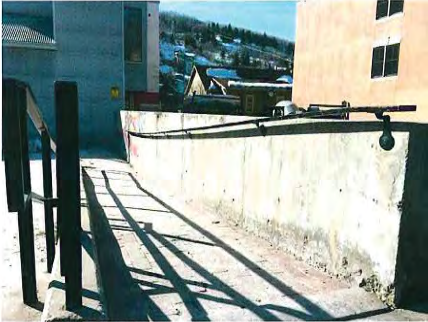
36 Patio - Rectangular Black Steel Mounted Ramp Railing
