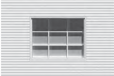
Top: These window openings are tall and narrow with wide trim and are spaced evenly on the wall plane. Middle/bottom: Original window openings and trim should not be altered, nor should the window itself be replaced with a type or style that is incompatible.
