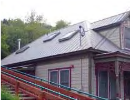
These skylights are flush mounted and unobtrusive when viewed from the public right-of-way.
