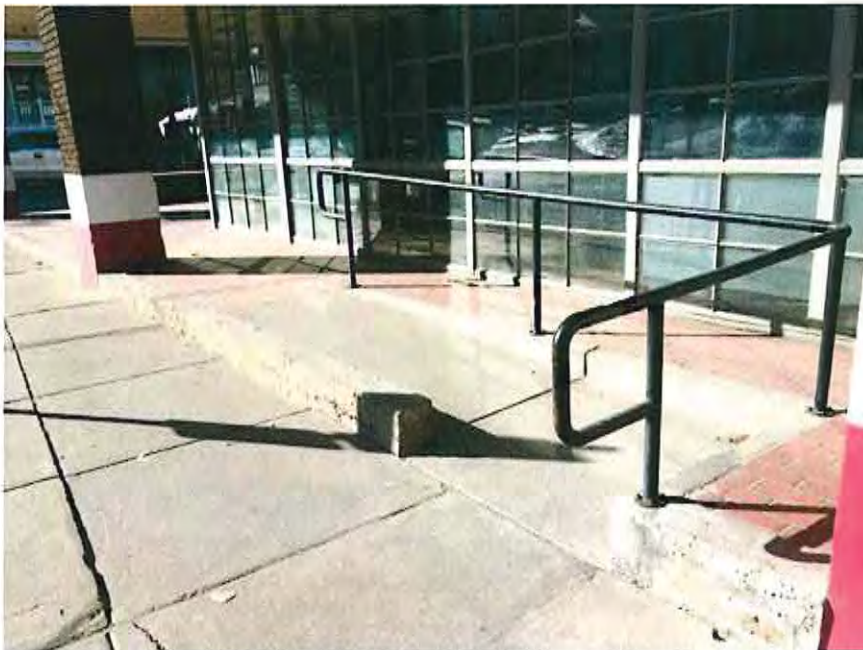
39 Heber Ave to Main Entrance - Black Steel Pipe Ramp Railing
