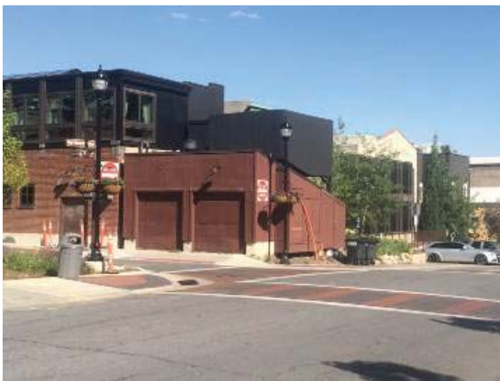
Mechanical equipment at 508 Main Street was installed on the shed roof of the garage and wrapped with the black fencing that shields it from view.
