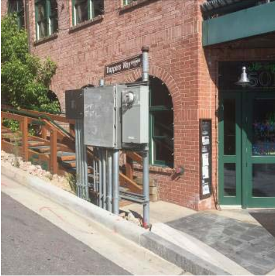
These electrical meters adjacent to 501 Main Street are highly visible and not shielded.
