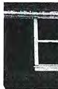
Does not appear operable
