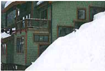
Foundation wall too exposed
