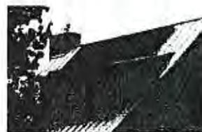
Solar panels located to maximize effectiveness and minimize visual impact
