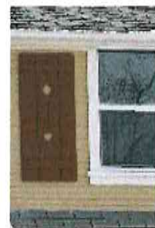
Does not appear operable
