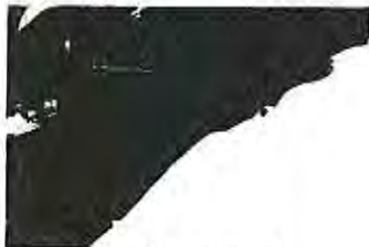
Foundation wall too exposed
