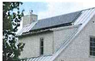
Solar panels located to maximize effectiveness and minimize visual impact
