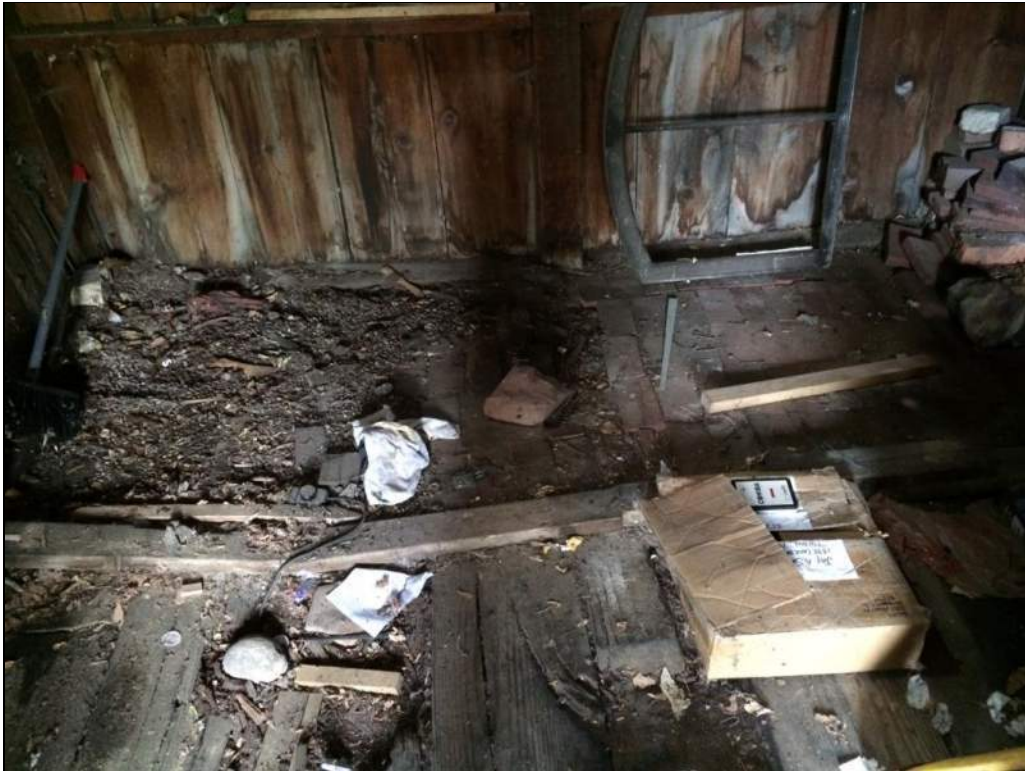
Figure 6. Garage floor, showing brickwork at west end and wood planks covering remainder of floor, facing west.
