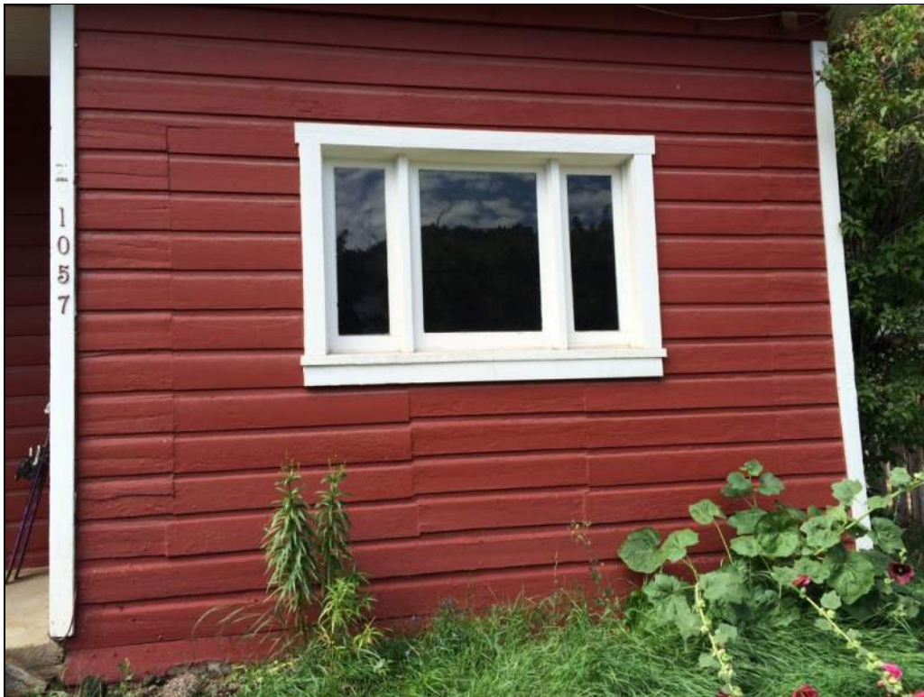
Figure 2. Detail of east façade of house, with original window locations visible in siding.
