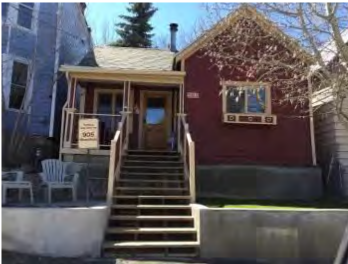
905 Woodside Avenue. Too much of the foundation is exposed. Historically, this house had a stacked stone foundation.
