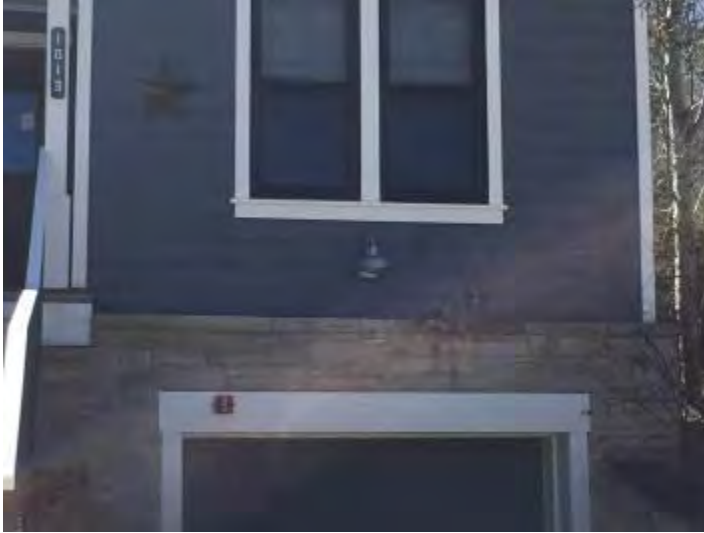
1013 Woodside Avenue. New foundations should not be proud of the historic wall plane.
