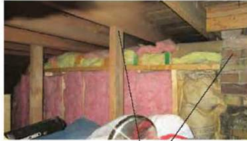
A2 FLAT ROOF RENOVATION STRUCTURE SHOWS THAT THE ROOF OVER THE CURRENT KITCHEN AREA IS NEW CONSTRUCTION. IT APPEARS ON THE SANBORN MAPS BUT IT WAS CLEARLY REMOVED AND RECONSTRUCTED AT SOME RECENT POINT IN TIME. ORIGINAL BRICK CHIMNEY MODERN STRUCTURAL MEMBERS
