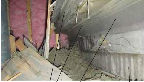
A3 ENCLOSED WITHIN THE ATTIC IS THE ORIGINAL FRIEZE AND FASCIA THAT FOLLOWS THE ORIGINAL HALF OCTAGON ROOF HISTORIC WOOD FASCIA HISTORIC DECORATIVE MOLDING
