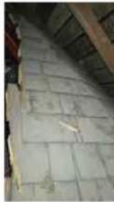
A4 A REMNANT SHOWING 2 SECTIONS OF THE HALF-OCTAGON ROOF IS NOW ENCLOSED IN THE ATTIC WHERE THE HIP ROOF WAS EXTENDED WAS HISTORIC LAP SIDING
