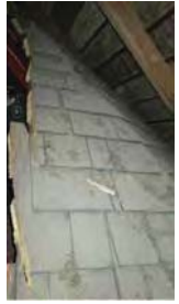
A4 A REMNANT SHOWING 2 SECTIONS OF THE HALF OCTAGON ROOF IS NOW ENCLOSED IN THE ATTIC WHERE THE HIP ROOF WAS EXTENDED HISTORIC LAP SIDING
