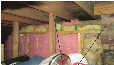
A2 FLAT ROOF RENOVATION STRUCTURE SHOWS THAT THE ROOF OVER THE CURRENT KITCHEN AREA IS NEW CONSTRUCTION. IT APPEARS ON THE SANBORN MAPS BUT IT WAS CLEARLY REMOVED AND RECONSTRUCTED AT SOME RECENT POINT IN TIME. ORIGINAL BRICK CHIMNEY MODERN STRUCTURAL MEMBERS
