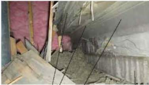
A3 ENCLOSED WITHIN THE ATTIC IS THE ORIGINAL FRIEZE AND FASCIA THAT FOLLOWS THE ORIGINAL HALF-OCTAGON ROOF
