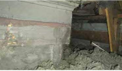
A5 HISTORIC FRIEZE AND FASCIA IS SHOWN AS IT ROUNDED THE FRONT CORNER OF THE HOUSE
