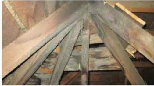
A1 HISTORIC HIP ROOF STRUCTURE OCCURS INSIDE OF CURRENT HIP AND SHOWS THE ROOF WAS ORIGINALLY HALF OF AN OCTAGON
