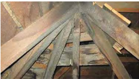
A1 HISTORIC HIP ROOF STRUCTURE OCCURS INSIDE OF CURRENT HIP AND SHOWS THE ROOF WAS ORIGINALLY HALF OF AN OCTAGON
