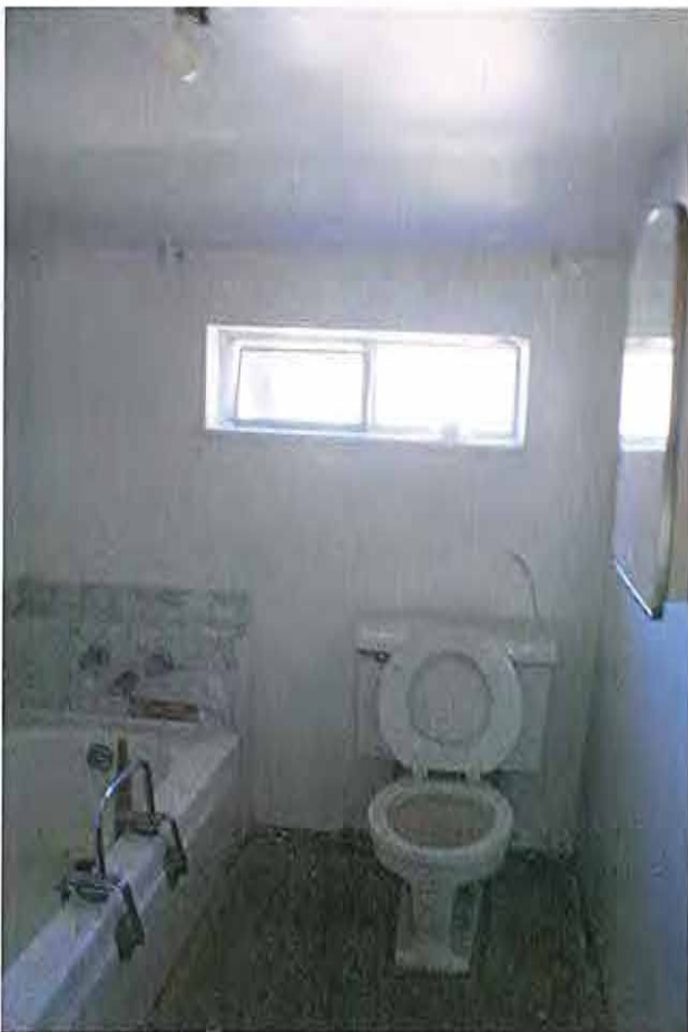
Tub and toilet
