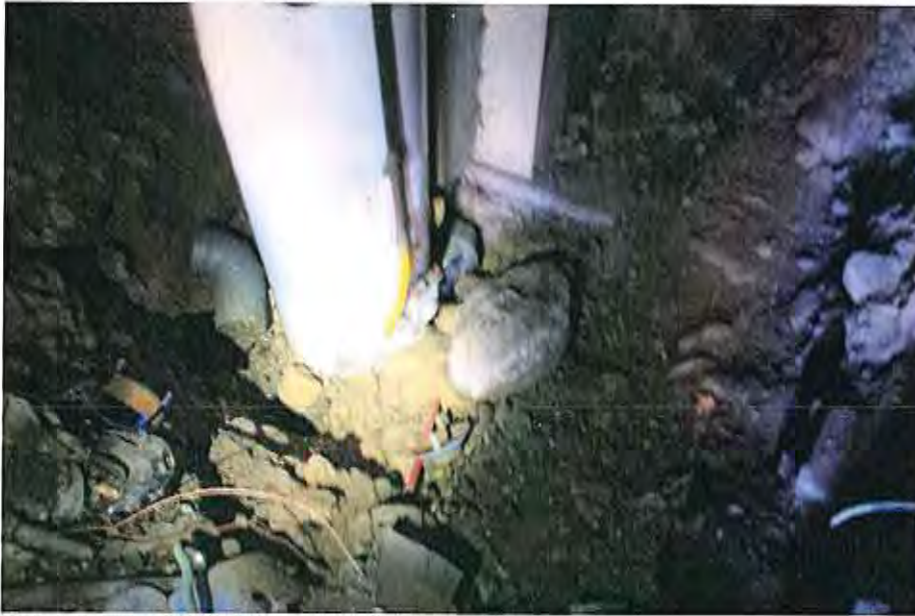
Damage to existing foundation-rubble fallen
