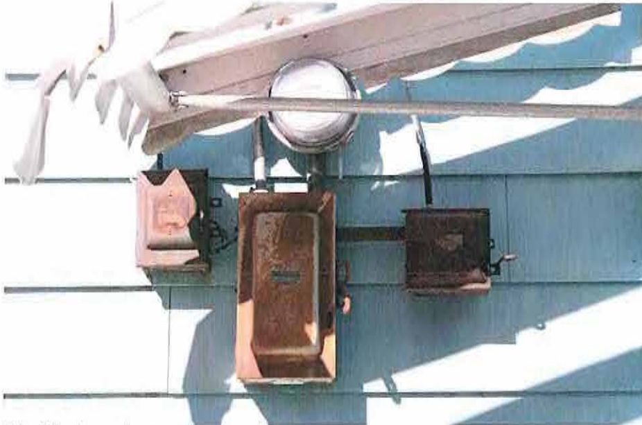
Electrical service-south elevation
