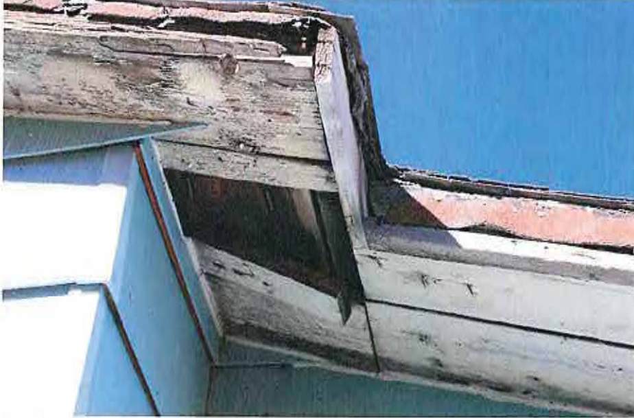
Test materials siding and roofing for asbestos. Assume age of house there will be lead paint.
