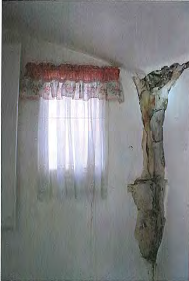
Visible mold-probably hidden mold
