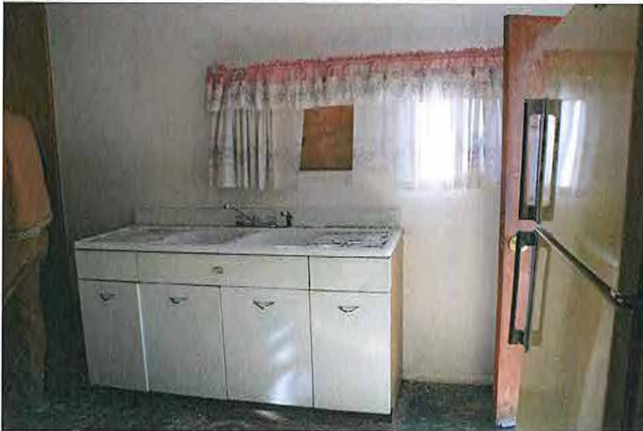
Possible lead piping
