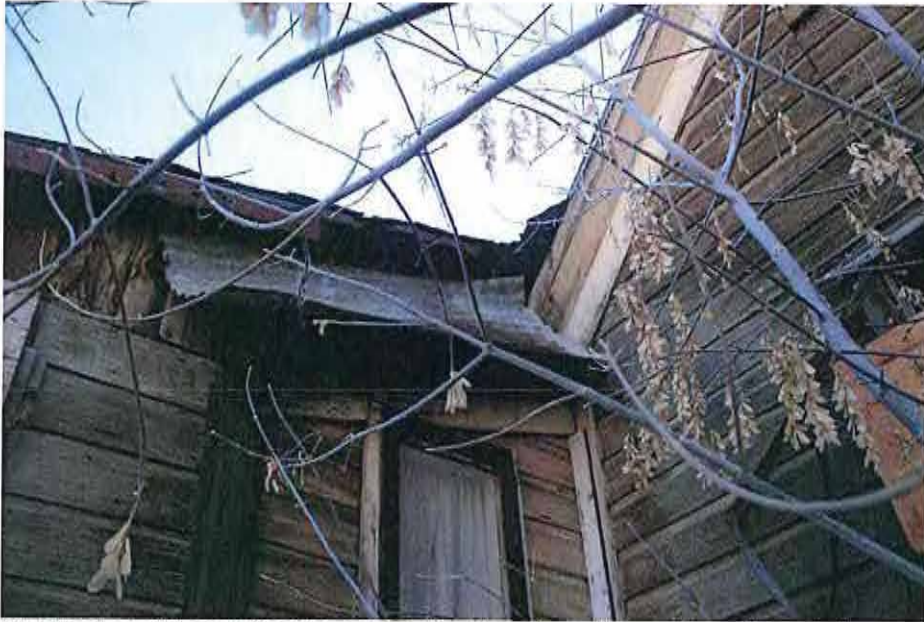
Original soffit and fascia on east side of north-south gable. Intersecting shed roof and soffit and fascia has water damage and layers of makeshift repairs.
