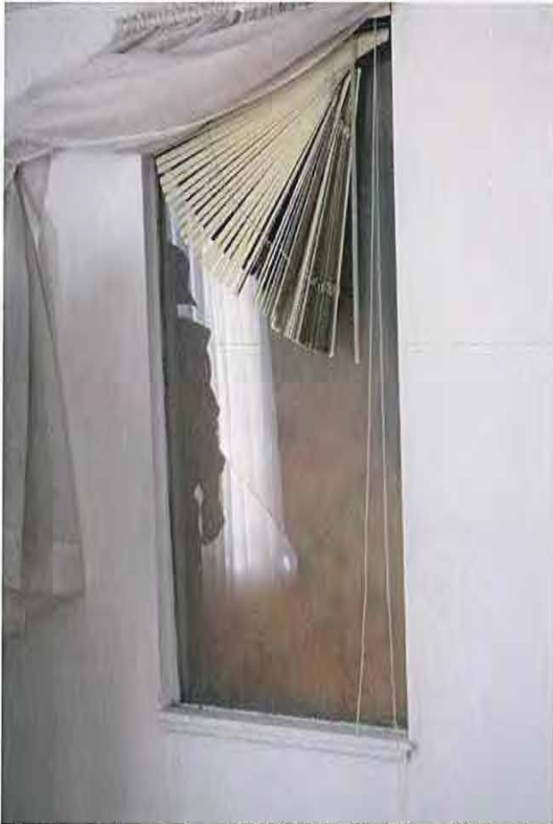
West porch window-2'-7"WX5'-8"H fixed 24" off porch 2" historic wood casing exterior, interior modified
