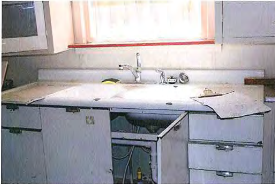
4. Metal kitchen sink and cabinet unit
