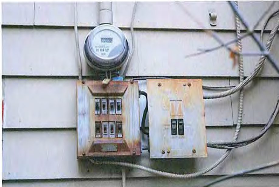
2. Closeup electrical service
