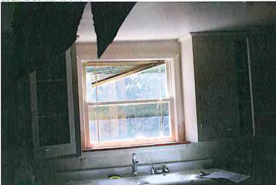
Interior of kitchen window with surrounding cabinets. Note ceiling damage.
