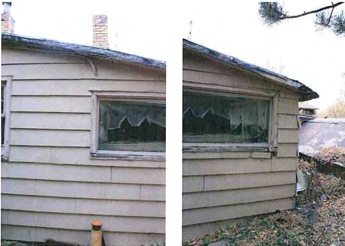
There is a large fixed single pane window in the mechanical room. It is 3'-3" off the ground and 4'-8" W X 2'-2" H. It has similar jamb and sill detail shown above.
