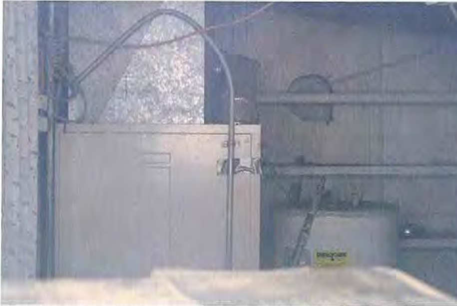
1.Mechanical room-furnace and water heater
