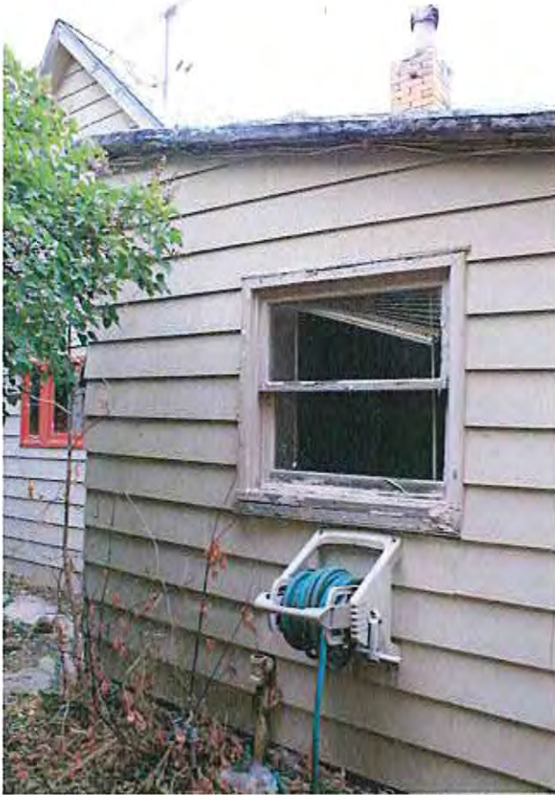
The kitchen window is a wood, single-pane, double hung window. This window is 3'-8 1/2" off the ground and is 3'-0"W X 2'-8"H. The paint is peeling and there is some raw wood. The window detail is similar to above.
