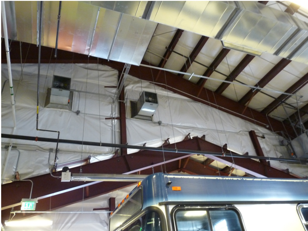
FIGURE B.1-8: EXISTING WALL MOUNTED EXHAUST FANS
