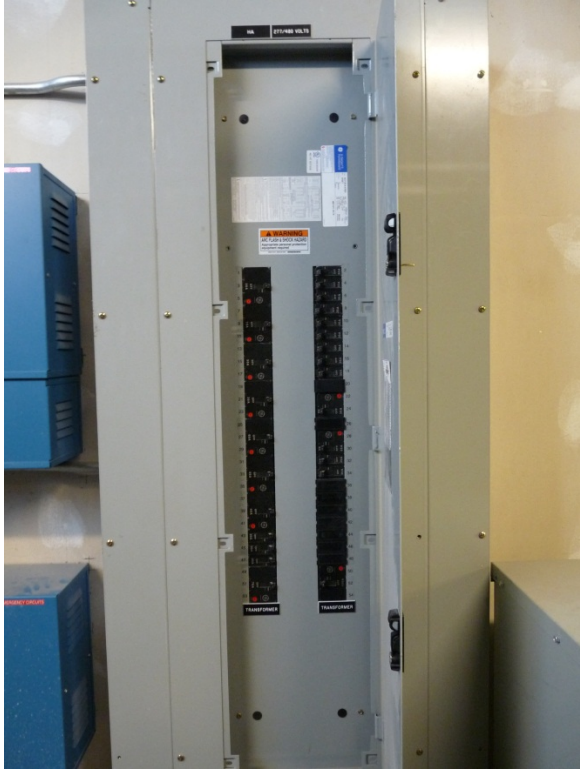
FIGURE B.1-3: EXISTING ELECTRICAL PANEL
