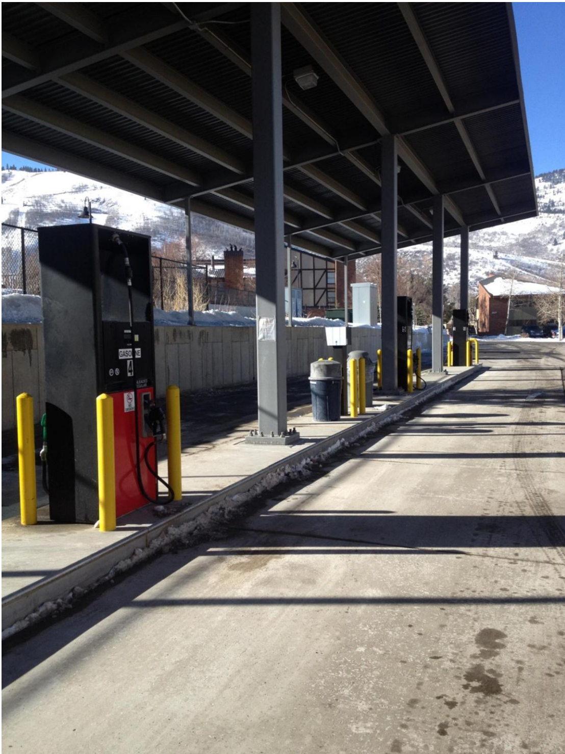
Figure 6. Diesel and Unleaded Dispensers
