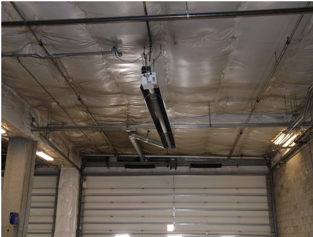
FIGURE B.1-2: EXISTING TUBE HEATER IN THE PARKING AREA
