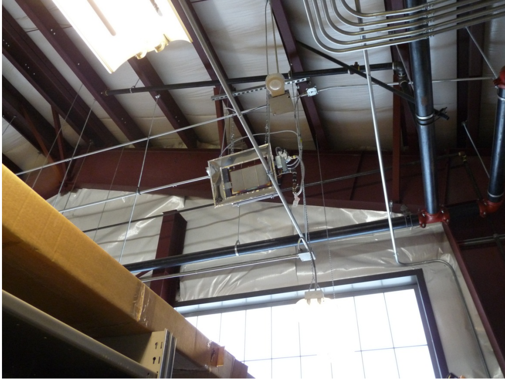
FIGURE B.1-7: EXISTING ELECTRIC UNIT HEATER
