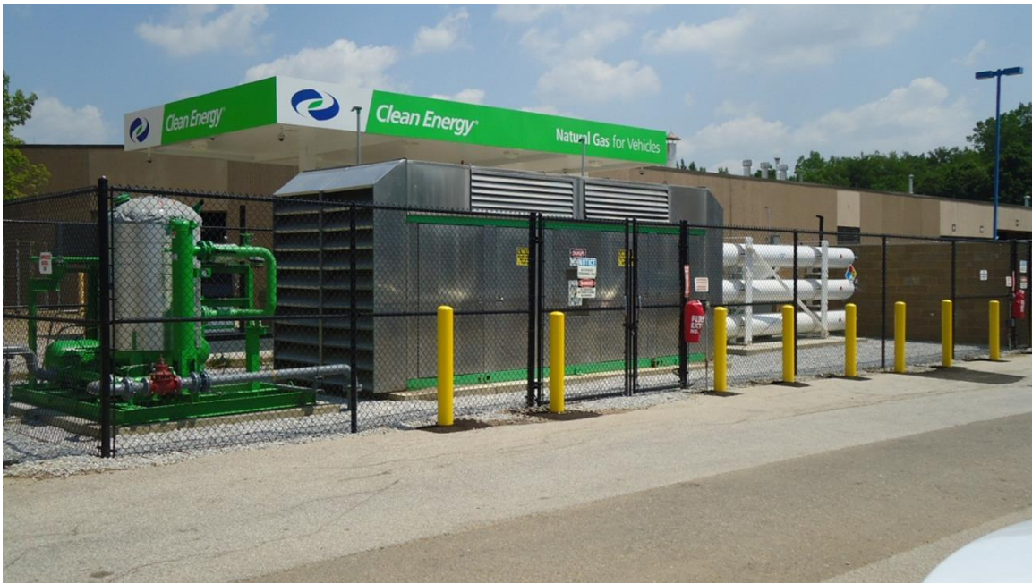
Figure 3. Single IMW (150 hp) skid with dryer, storage and dispenser
