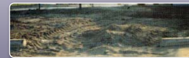
Here, a section of precast curb was completely pulverized by construction equipment at a shopping center.
