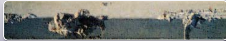
This precast curb was installed fifteen months ago and has been damaged by impact. It is highly susceptible to chemical freeze/thaw damage and will continue to disintegrate.
