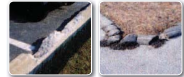
Concrete curb cannot survive even a short period if it is not backed up by soil. Berm always fails the snowplow test.
