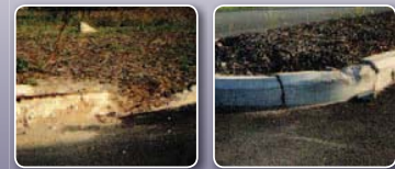
The effects of impact are obvious in these examples of precast curb installed less than three years ago.
