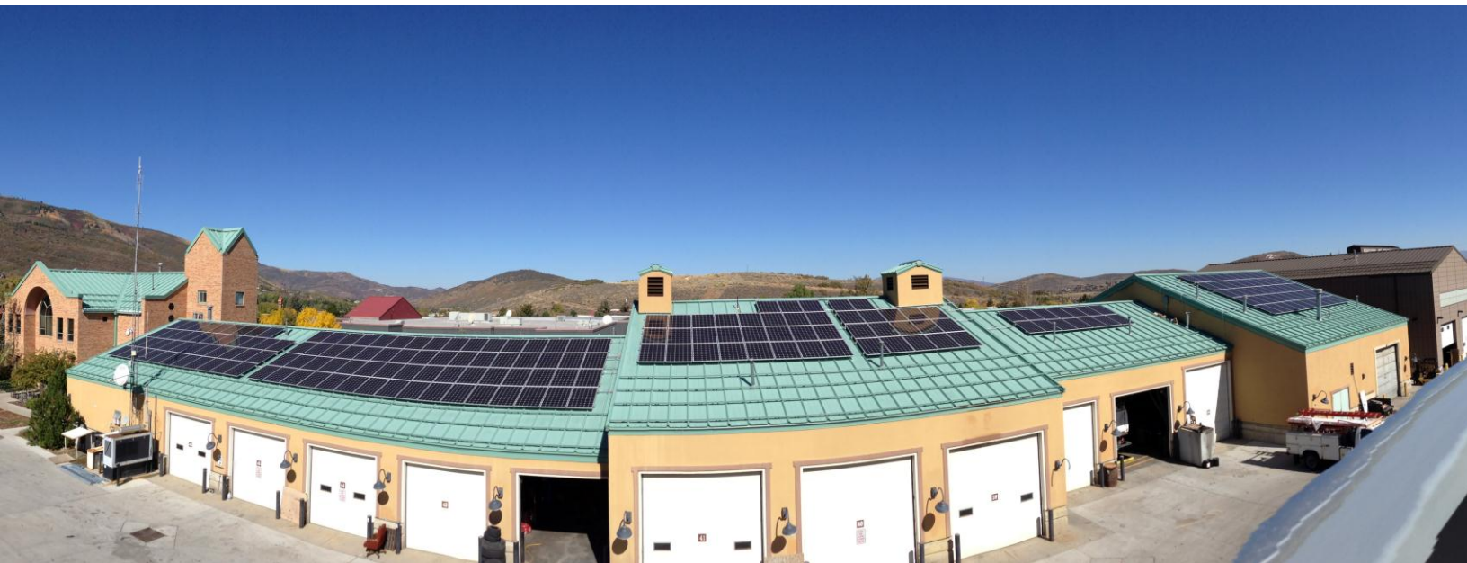
Panoramic Solar Array at Iron Horse Transit Facility
